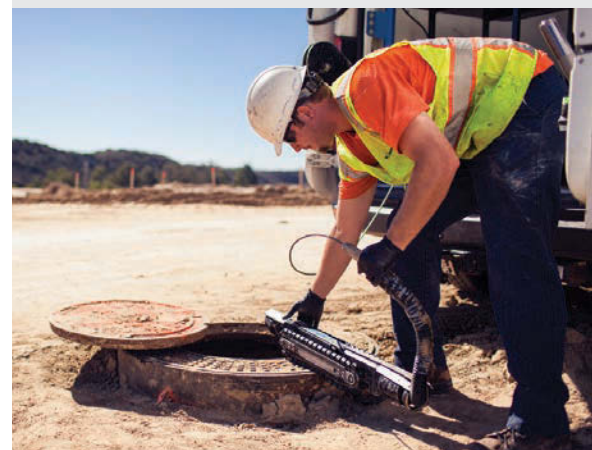
BELOW: After confirming the route for the next run of pipe, Andrew Wise launches a ProTRAK crawler and TrakSTAR camera (RS Technical Services) to inspect a section of pipe just cleaned by the company's jetting team.
