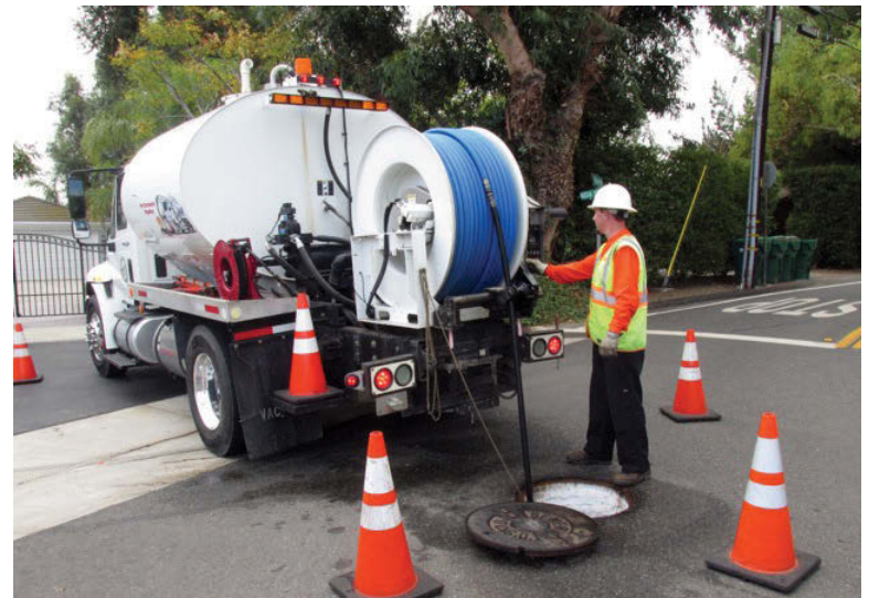
Performance Pipeline Technologies jetter operator Dan Schuler cleans a sewer line with one of the company's five Ramjet V8015 waterjetting trucks from Vactor Manufacturing.
