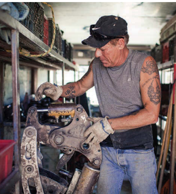
John Barron prepares the HammerHead PB30 hydraulic winch to pull the new HDPE pipe through the existing lateral line.
