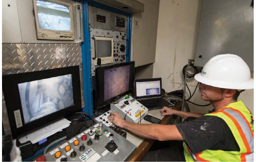
Zach Andrews operates the Aries CCTV system in the control room of the inspection van during a pipe relining project.
