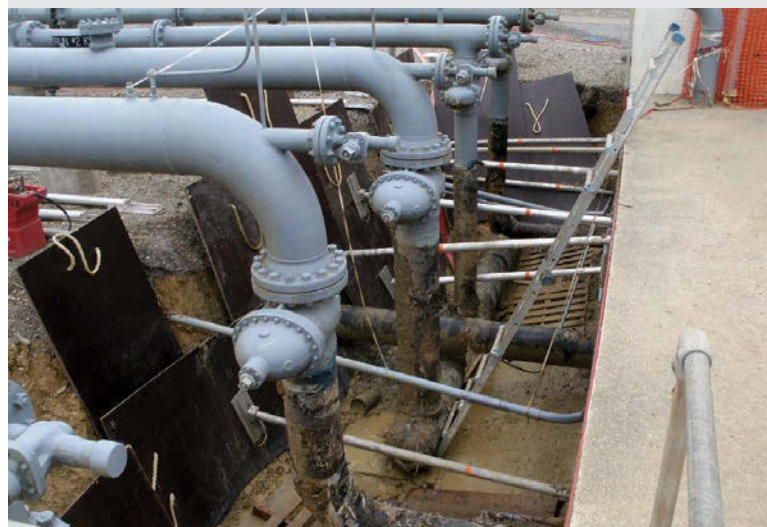
BELOW: The beginning section of the 50-foot-long outflow trench was a maze of piping and shoring board braces.
