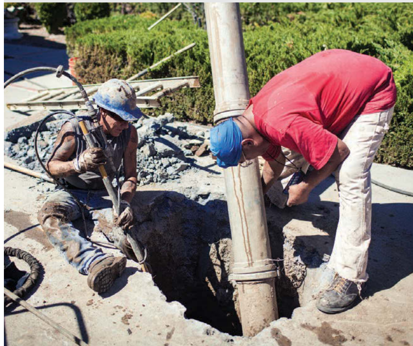
BELOW: John Barron (left) and Fred Cortez use a Vac-Con hydroexcavator to clear debris from the entry pit at the start of a pipe bursting job.
