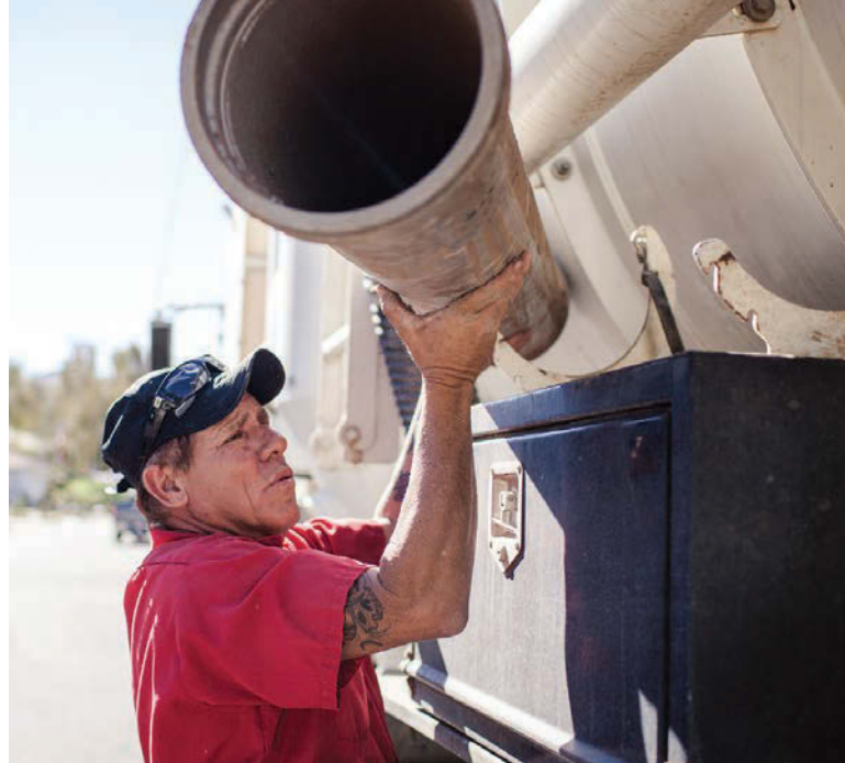
John Barron removes sections of vacuum tube from the side of the Vac-Con as the crew sets up to hydroexcavate an entry pit in a client's driveway.
