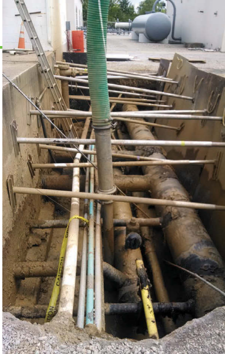
ABOVE: Shoring board braces add to the congestion in the inflow trench.
