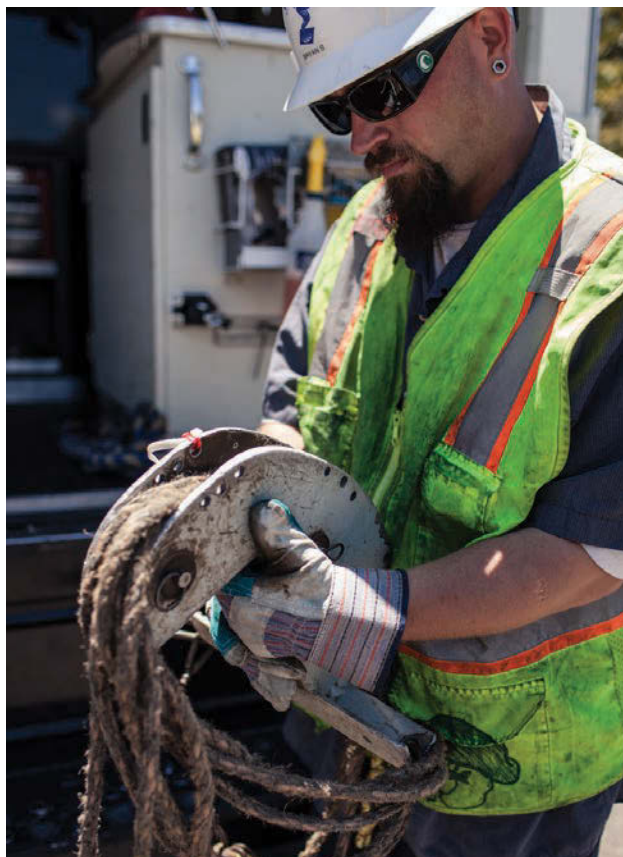
Bryan Sledzinski prepares support equipment for the CUES Ultra Shorty 21 mainline tractor at the start of a 6-inch sewer main inspection.
