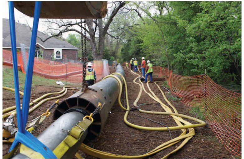
The No-DigTec crew loads the rear 20-inch Mole pneumatic rammer into its casing and checks the air hoses before one of the runs. (Photo courtesy of John Boykin)
