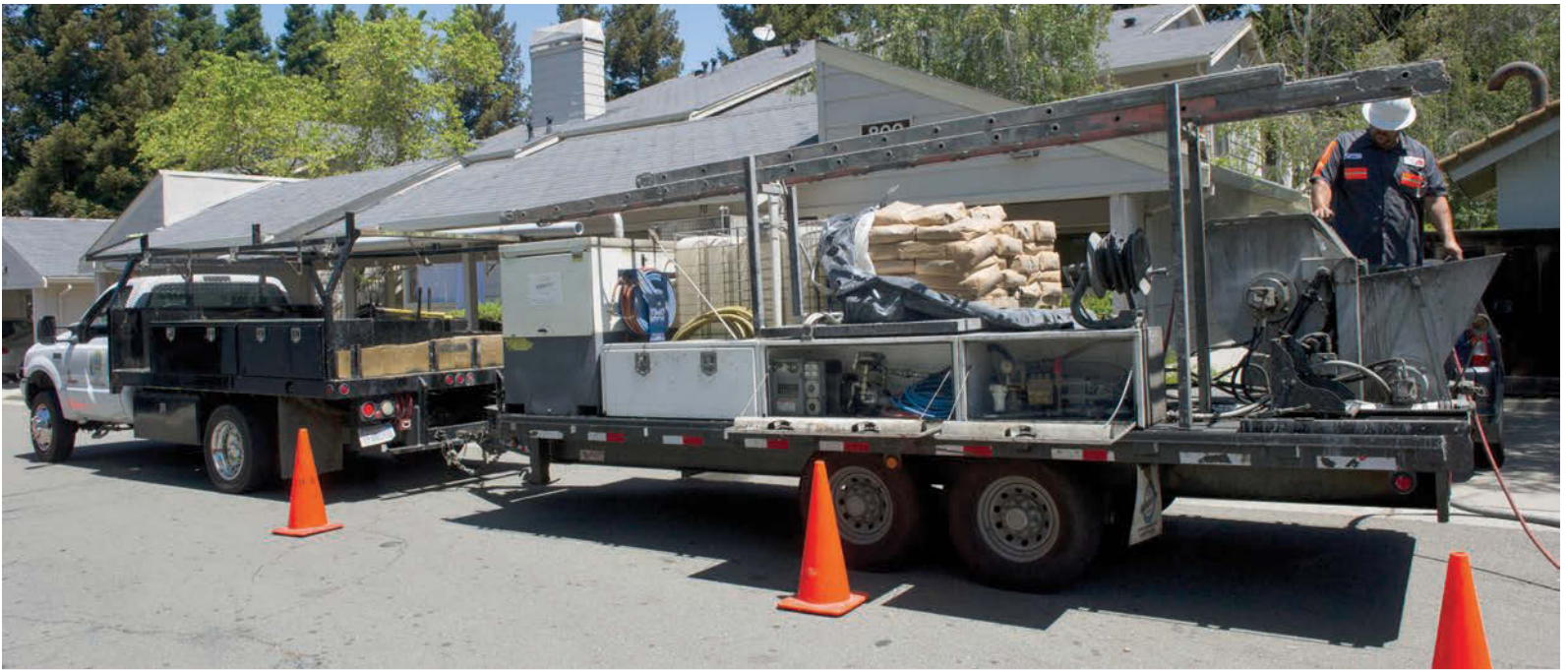
H&R Plumbing's manhole rehabilitation trailer, shown here on a job site, is fully outfitted with equipment and materials from Madewell Products.
