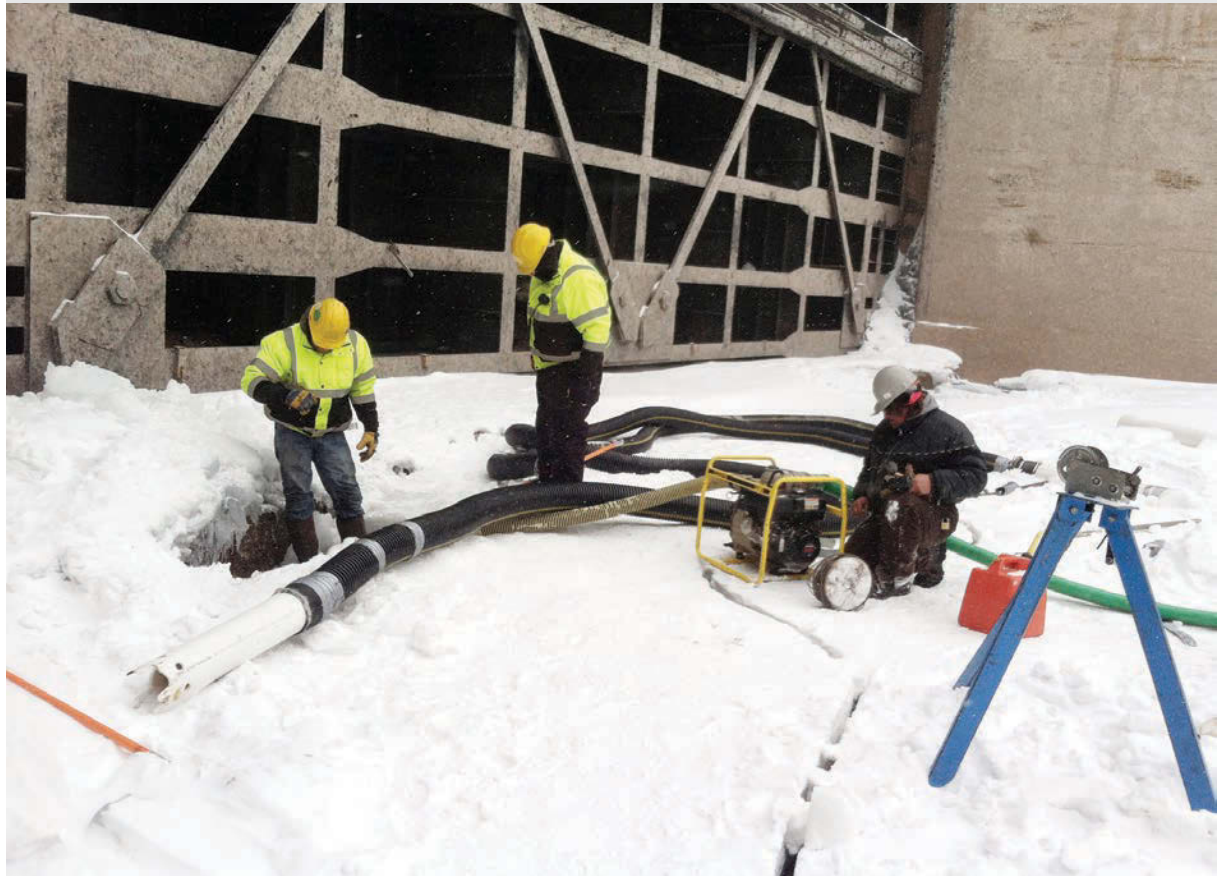
LEFT: Tarps shield a 2100 Series Vactor from the cold. The truck, parked near Gate 2, is 70 feet above the Poe Lock floor. A 90-degree elbow connects the shoot to 260 feet of 8-inch Schedule 40 PVC pipe. (Photos courtesy of Tunnel Vision Pipeline Services) BELOW: Richard Solka (left) and Josh Villeneuve (center) prep a sealed manhole for sediment removal, while Scott LaCombe coaxes a 3-inch dewatering pump to life. Gate 3 holds back the St. Marys River and Lake Huron.
