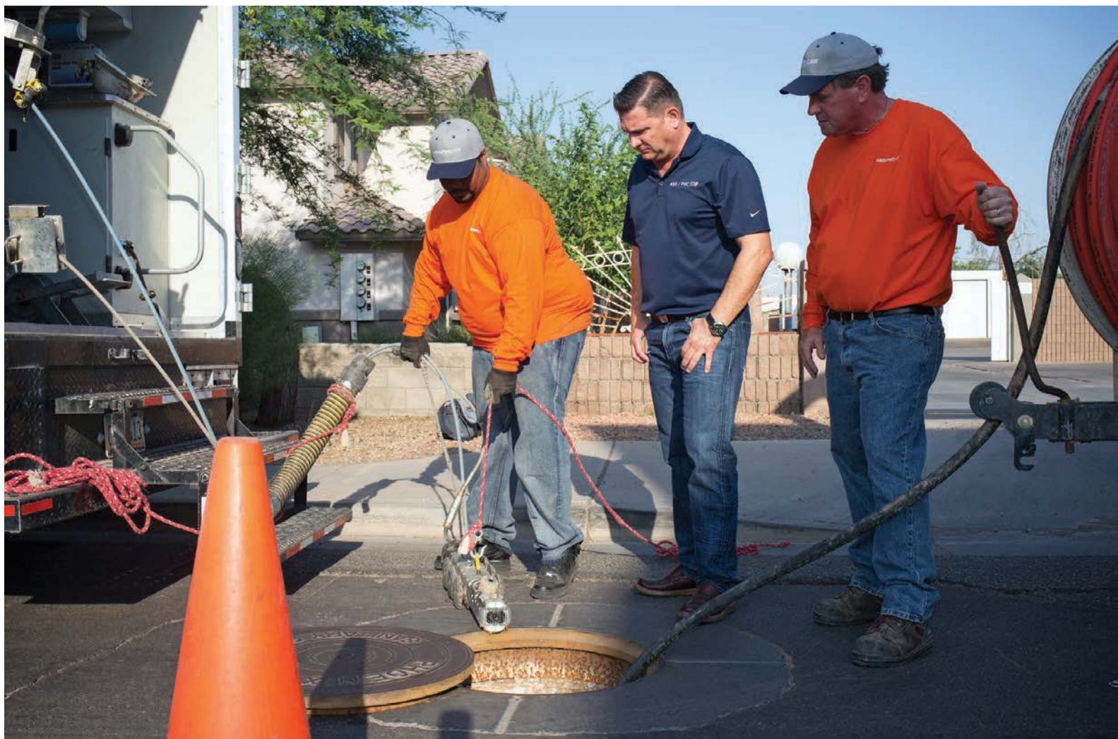
Yusuf Munir (left) lowers a camera into a manhole to begin an inspection with Chris Mihaletos (center) and Tom Verbridge.
