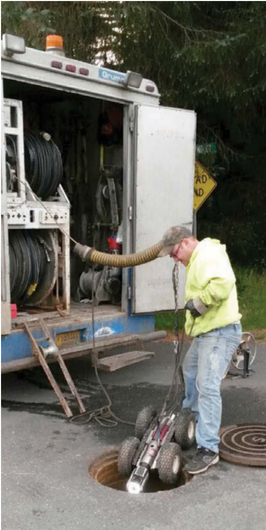
Daniel McCoy, CCTV technician, lifts the Aries camera system, outfitted with big wheels for inspecting large diameter pipe, out of the manhole following an inspection.
