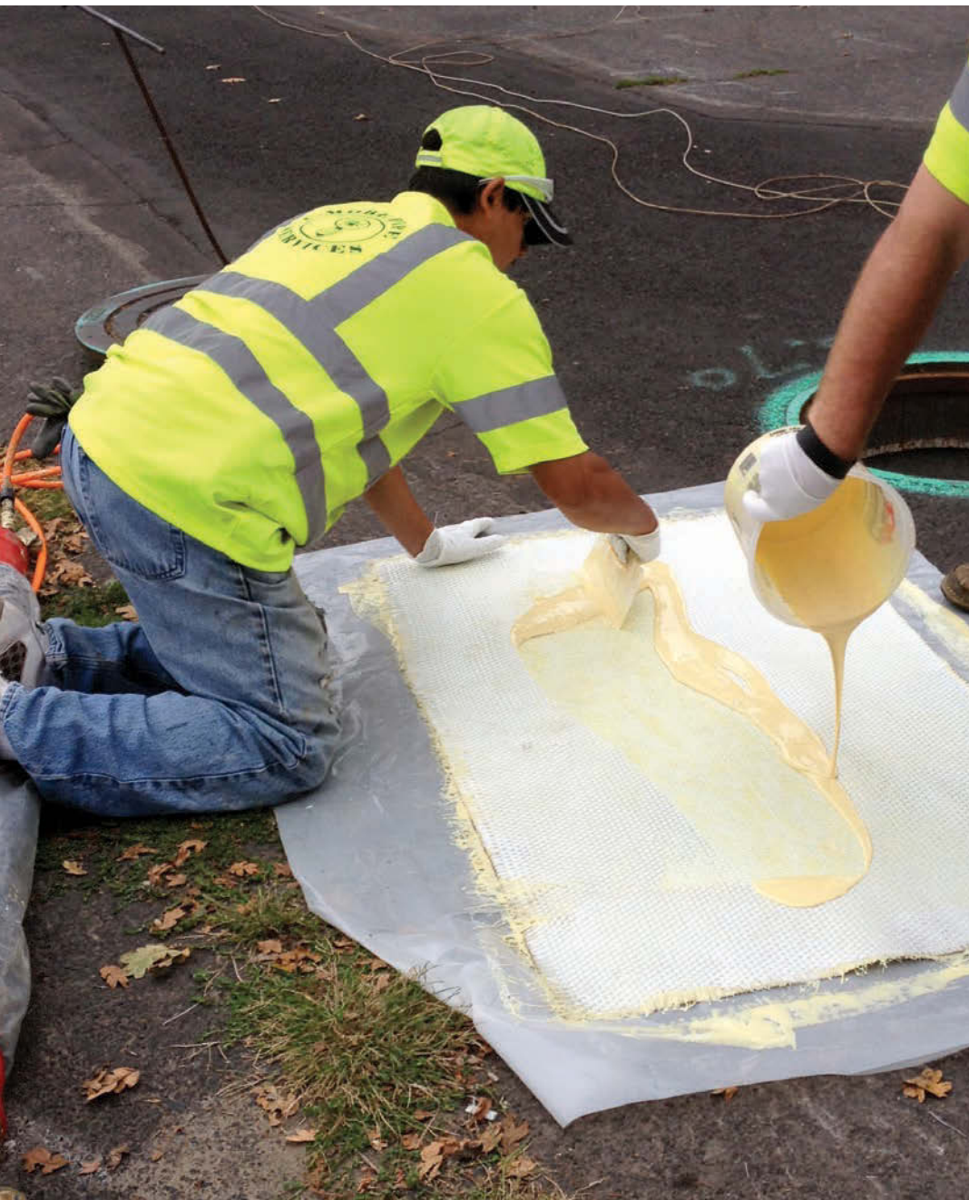
Juan Lorenzano, left, prepares a CIPP point repair blanket for installation for the City of Gladstone, Ore.
