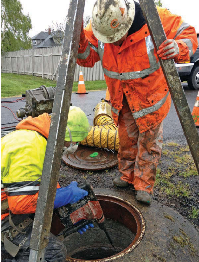
Manhole rehab technician Michael Champagne (left) and crew lead Terry Burrows chip away old joint sealing material before chemically sealing the manhole for the City of Halsey, Ore.
