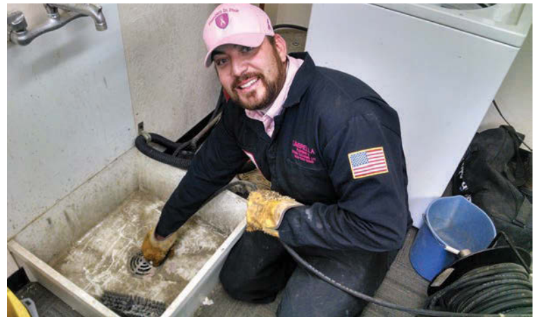
Umbrella Plumbing & Drain Cleaning Owner Marcus Rodriguez sets up to jet out a utility sink drainline.
