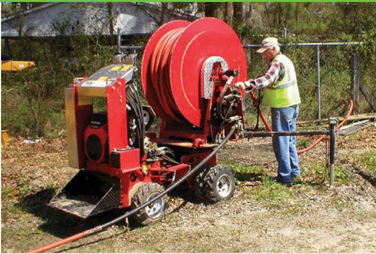
Ronnie Dugas, the owner of Video Pipe Inspection Inc. in Denham Springs, La., operates the company's SideKick easement reel, made by PipeHunter Inc.
