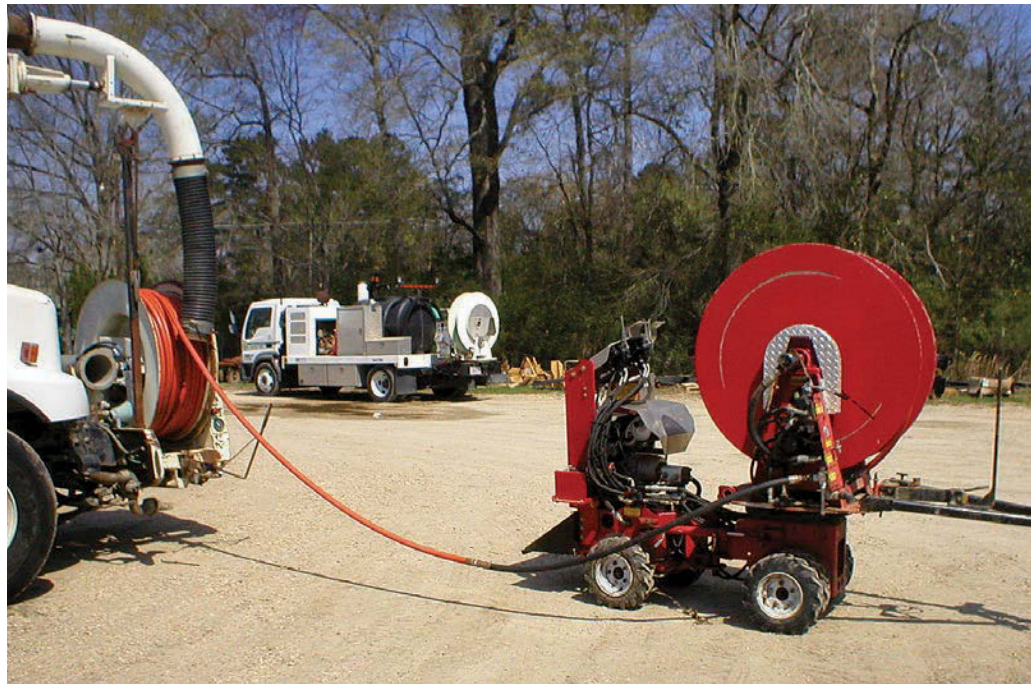
Donny Gerald, a technician at Video Pipe Inspection Inc., uses a SideKick easement reel, made by PipeHunter Inc., to transport a long jetter hose from a vacuum truck to a remote manhole location.
