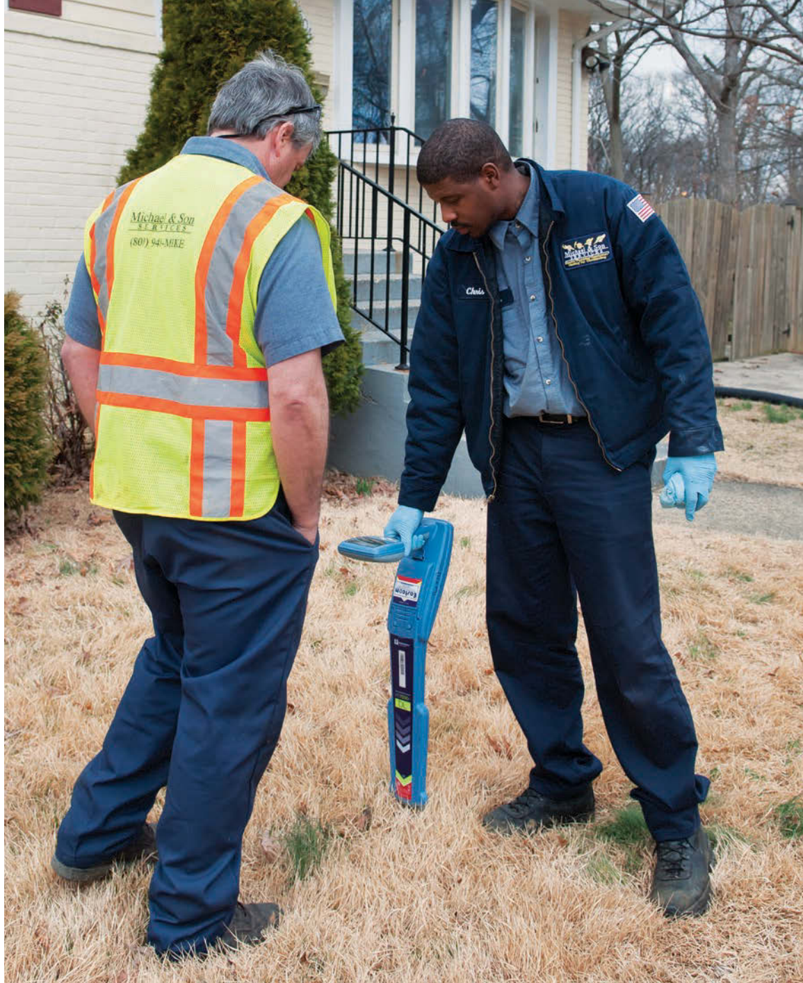
Field technician Ken Scott, left, looks on as Chris Kornegay uses an Eastcom RD7000+ locator to find the sewer line before drilling begins on a residential water line replacement in Alexandria, Va.
