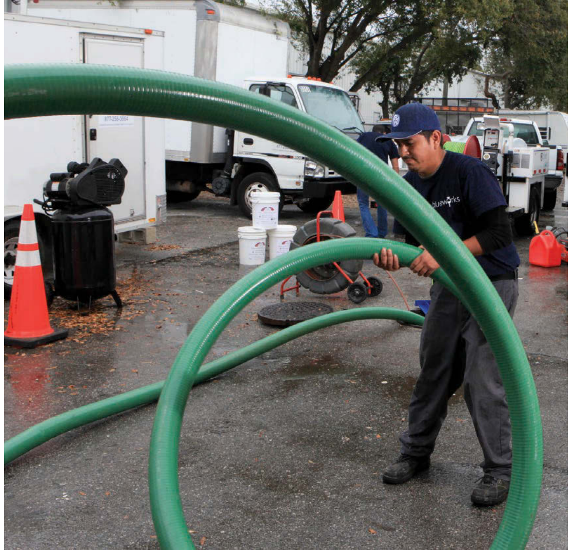
Eric Pinto uncoils a vacuum hose while the crew cleans and inspects a sewer main.
