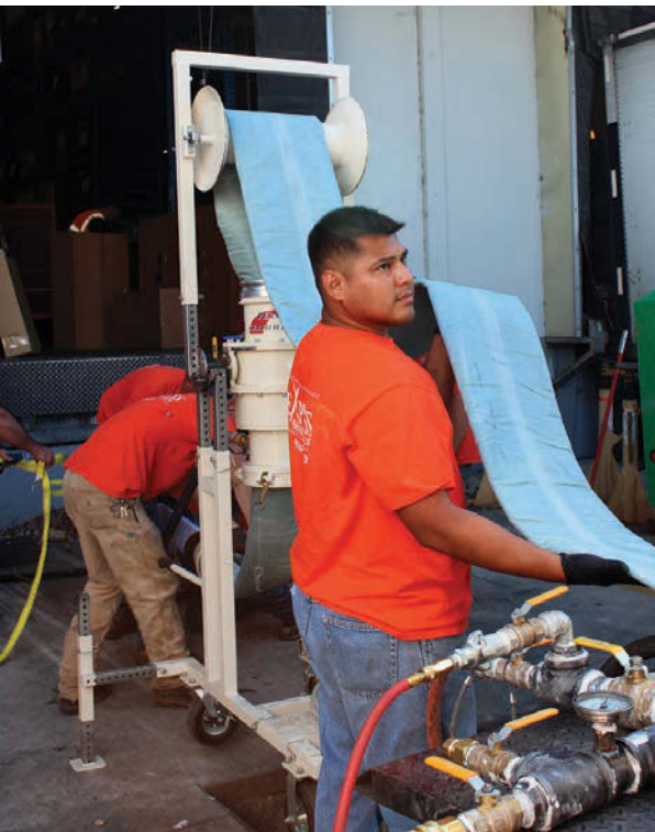
Aaron Gomez, an assistant technician with Express Sewer & Drain, feeds liner from a refrigerated truck into the Perma-Liner Top Gun inverter on a recent job. (Photo by Sang Heinselmann)
