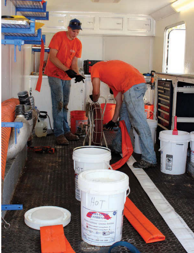
Russell Vankampen, left, and Ruvim Oleyic of Express Sewer & Drain prep the 4-inch liner inside a specialized trailer used for lateral lining. (Photo by Sang Heinselman)
