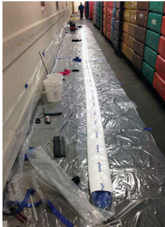
With the calibration bladder inserted, the Nu Drain liner from Nu Flow is ready to be rolled up and moved to the insertion point.
