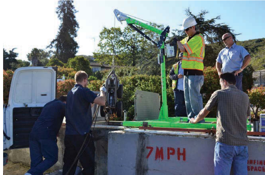
CCTV inspection equipment is most commonly damaged during insertion and removal through the manhole. Proper training and care is critical to keeping your operation up and running. (Photography by Jim Aanderud)
