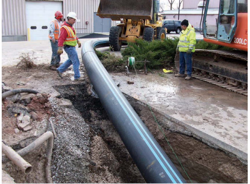
A John Deere payloader guides the 18-inch HDPE pipe and feeds it into the hole from the street, while a green tracer wire slides in beside the pipe.
