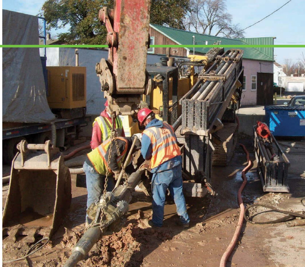
A chain and excavator boom help lift a 20-inch rock reamer as workers break apart the bore assembly in preparation for pulling drill rods to the south side of the Fox River power canal in Menasha, Wis. (Photos courtesy of Waas Boring and Cable)
