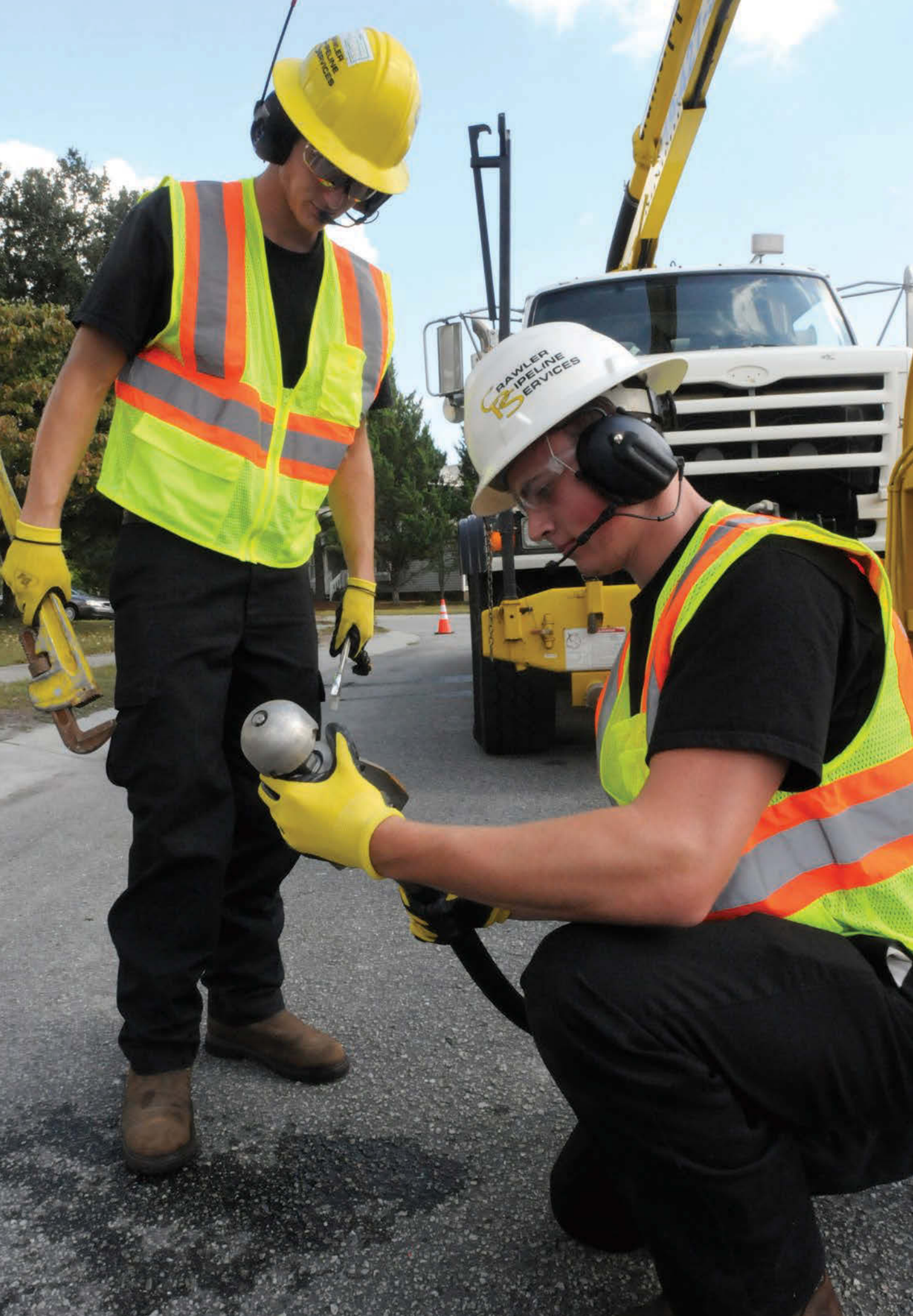
Crawler Pipeline Services technicians Dylan Williams (left) and Cody Thompson attach a cleaning nozzle to the water supply line from their Vac-Con truck.
