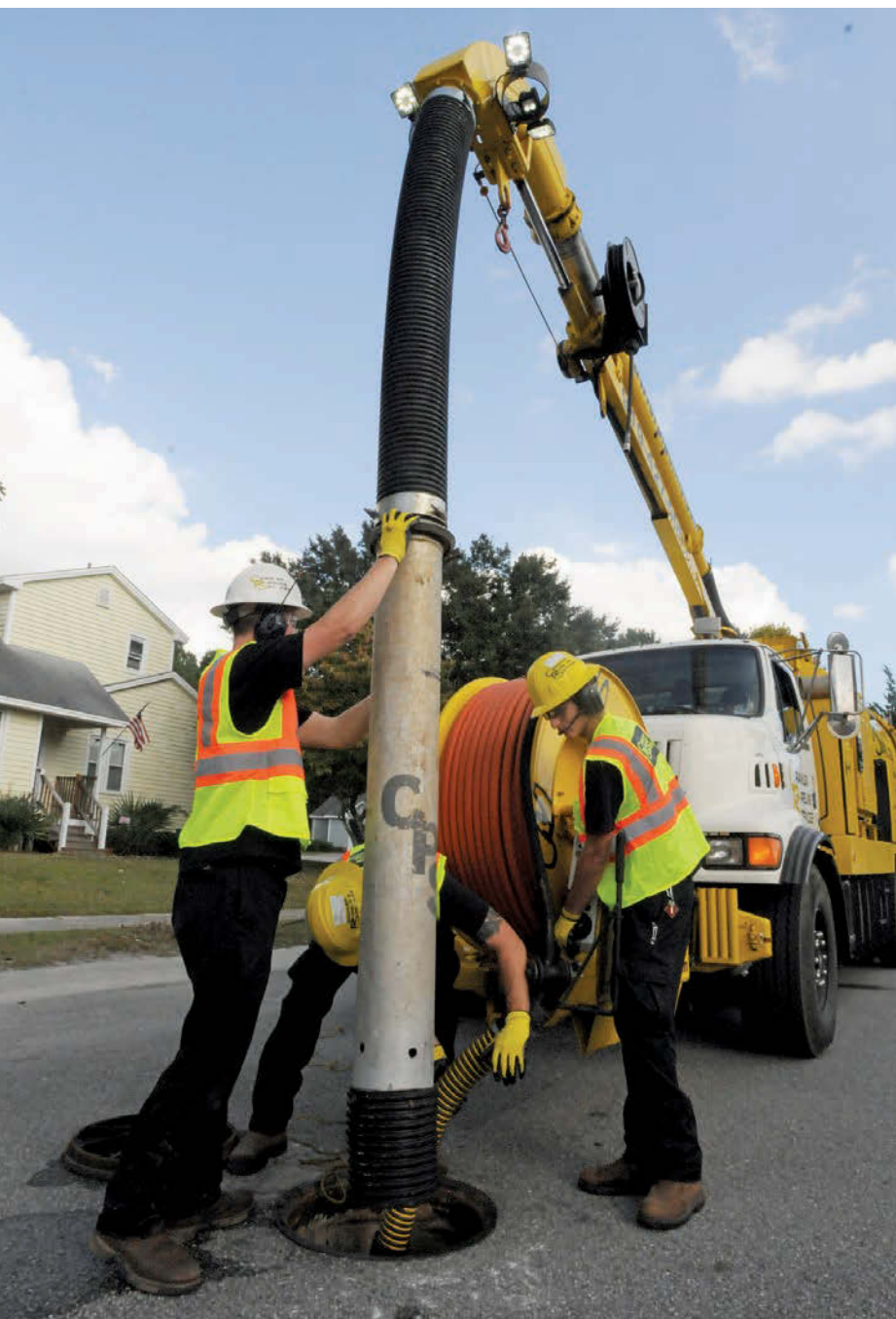
Technicians Cody Thompson, Trevor McGhee and Dylan Williams (from left) retrieve the Vac-Con's suction tube from a manhole.
