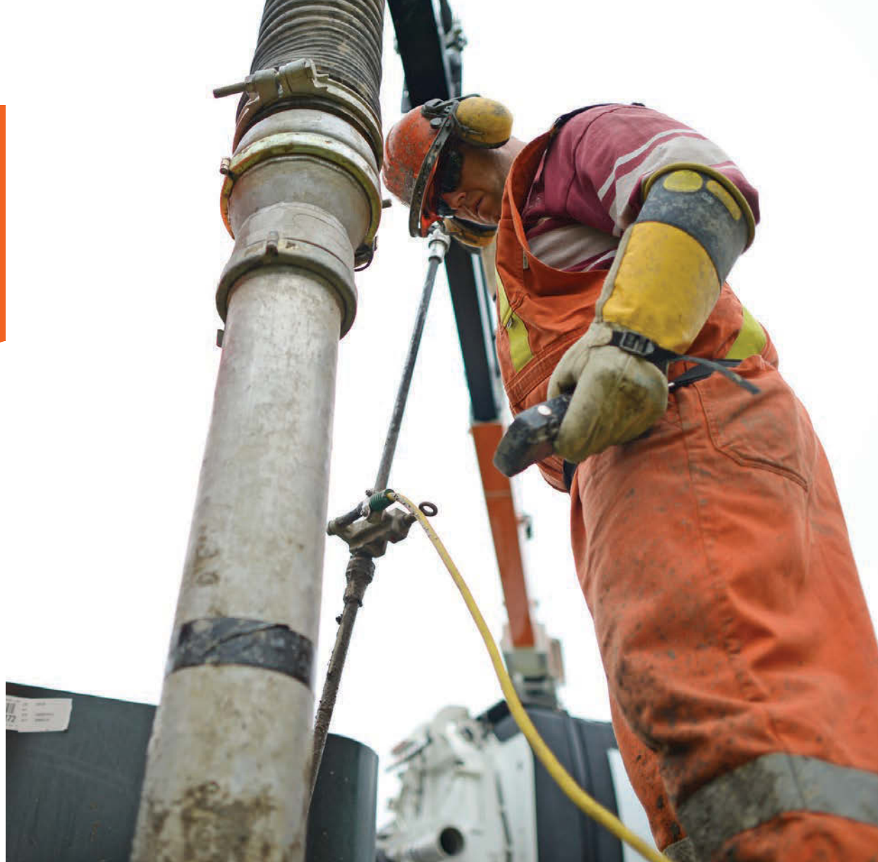
NCM Hydro Vac Owner and CEO Kris Norris excavates post holes for a sound barrier fence. Water, gas and fiber optic lines were all present.
