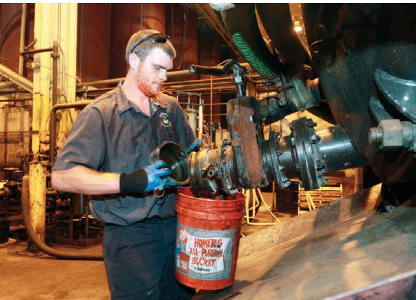
ODYSSEY employee Robert Davis catches wastewater discharge at Everclear of Ohio in Austintown, Ohio.
