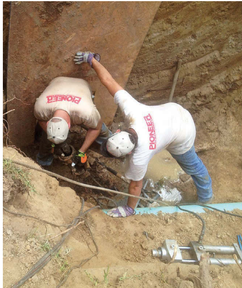
Matt Holtz and Brian Hester from Pioneer Comfort Systems notice that the bursting head looks a little strange as it emerges through the resistance plate. A 4-inch cast iron check valve is wrapped around the head. (Photos courtesy of Pioneer Comfort Systems)
