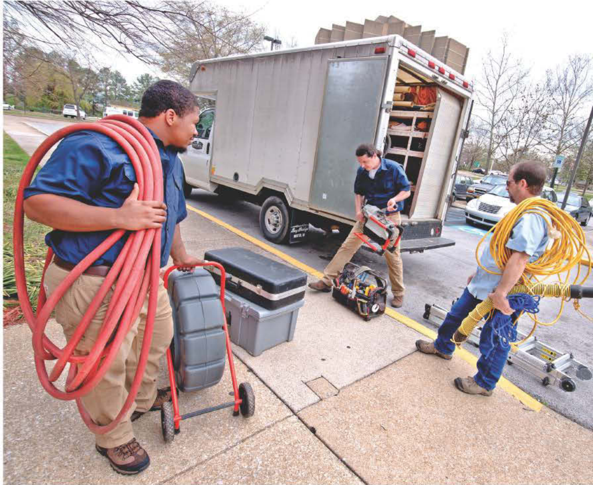
Daniel Baker and crew members Danzel Owens and Terry Turner unload equipment for a drain inspection job on the roof of Dogwood Manor, an 18-story high-rise in Chattanooga, Tenn.
