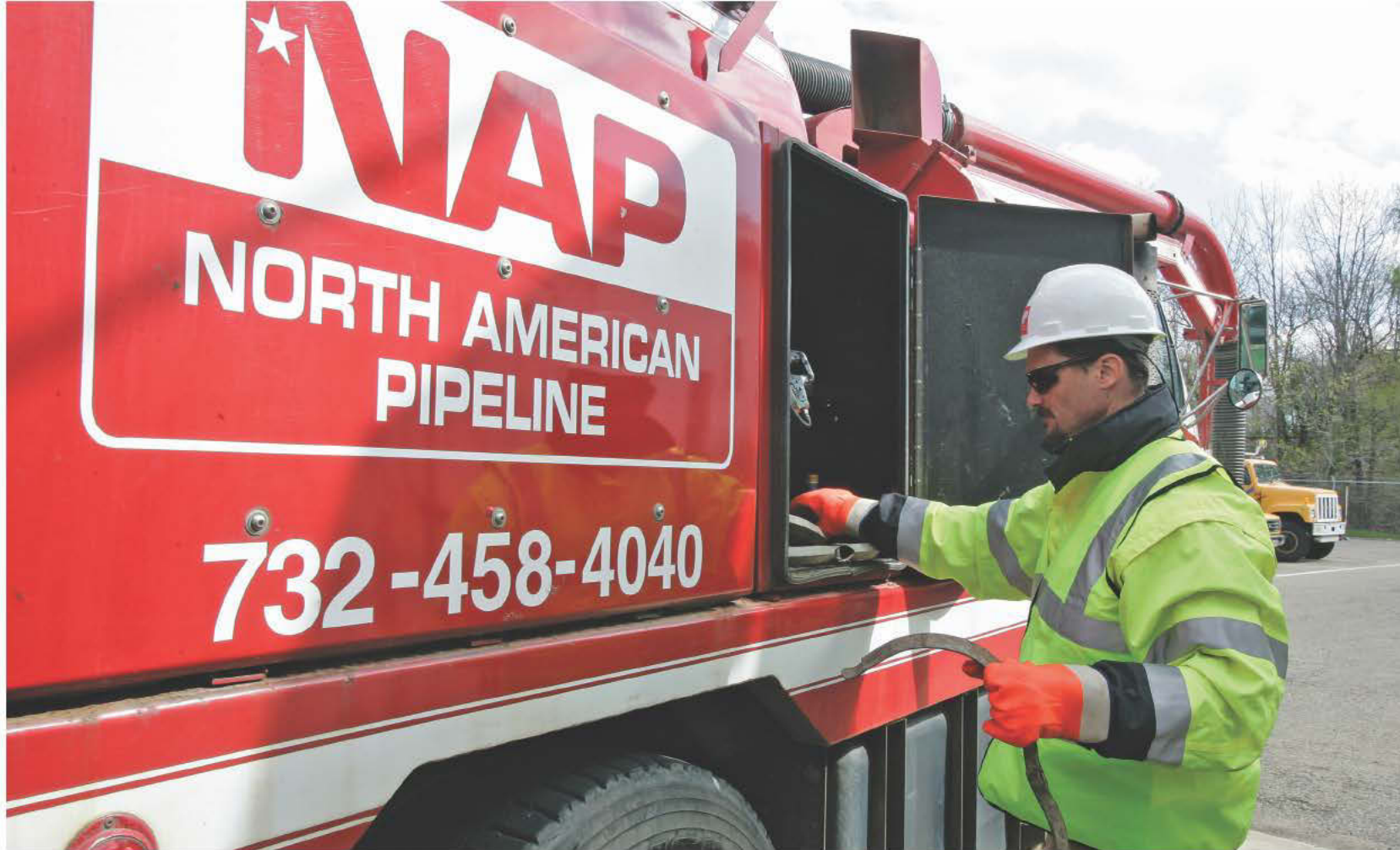
Brad Choppy pulls tools from a storage compartment on a jet-vac truck while working along the Garden State Parkway.
