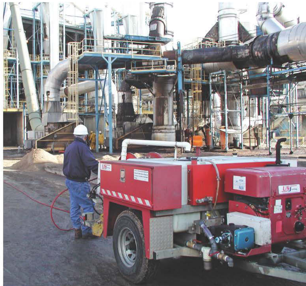
The US Jetting 4018 trailer jetter is used to clean the big stacks at a board factory with 4,000 psi at 18 gpm. (Photos courtesy of US Jetting)
