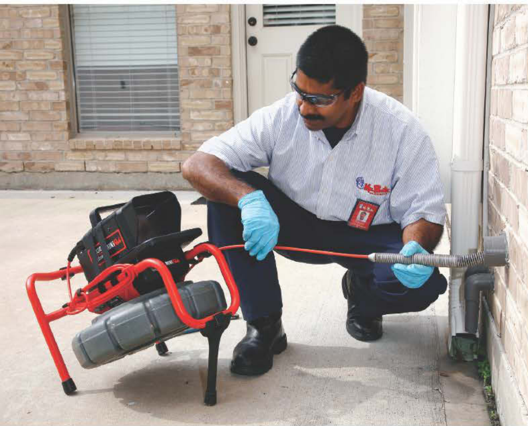
Renny Varghese uses a RIDGID SeeSnake inspection camera to inspect a pipe.
