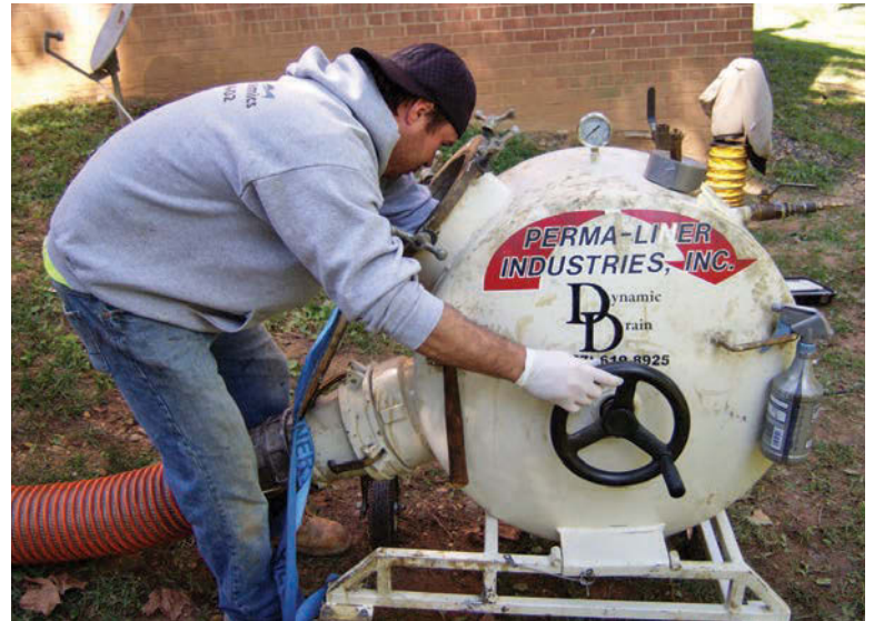
Wes Fogleman of Dynamic Drain Technologies loads the pull tape into the Perma-Liner inverter before loading the liner. (Photo courtesy of Dynamic Drain Technologies)
