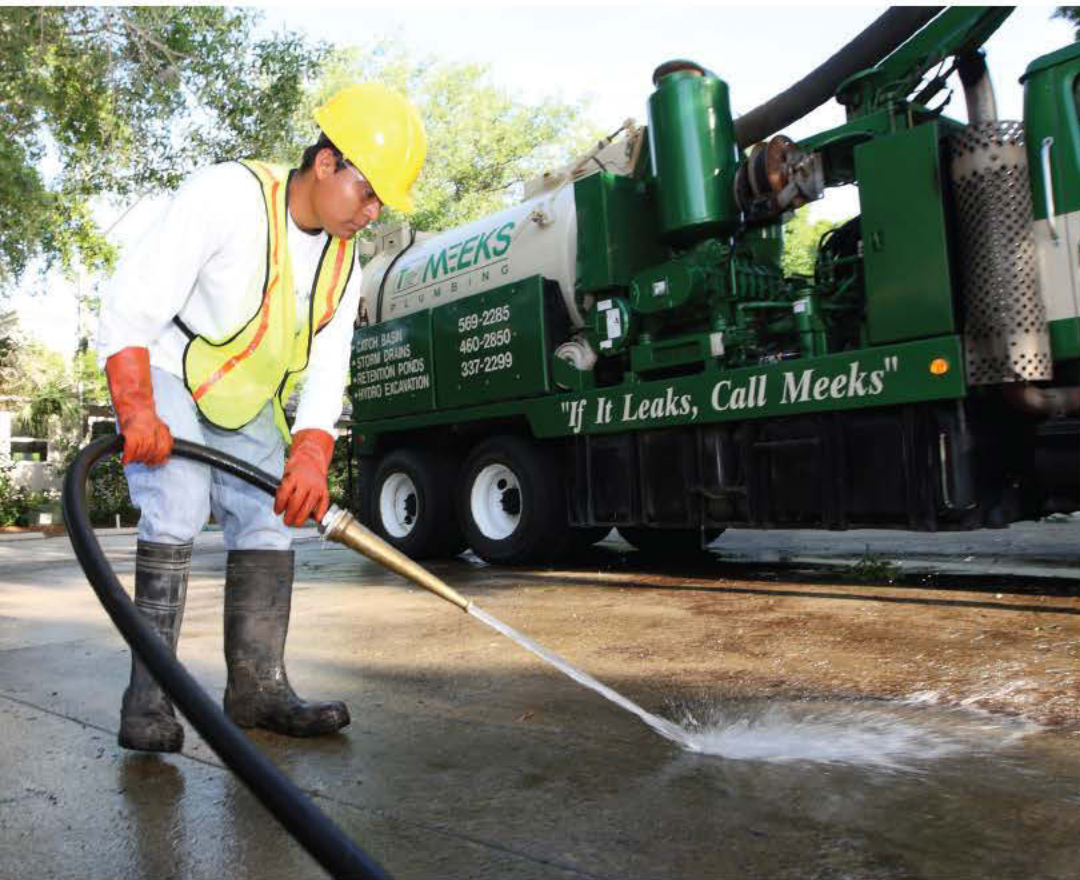
Apprentice plumber Vicente Mendoza hoses off the ground after a hydroexcavation job.
