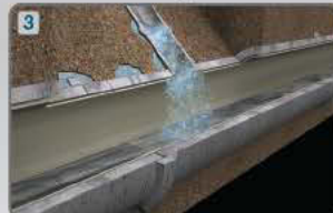
Continues to leak in annular space
