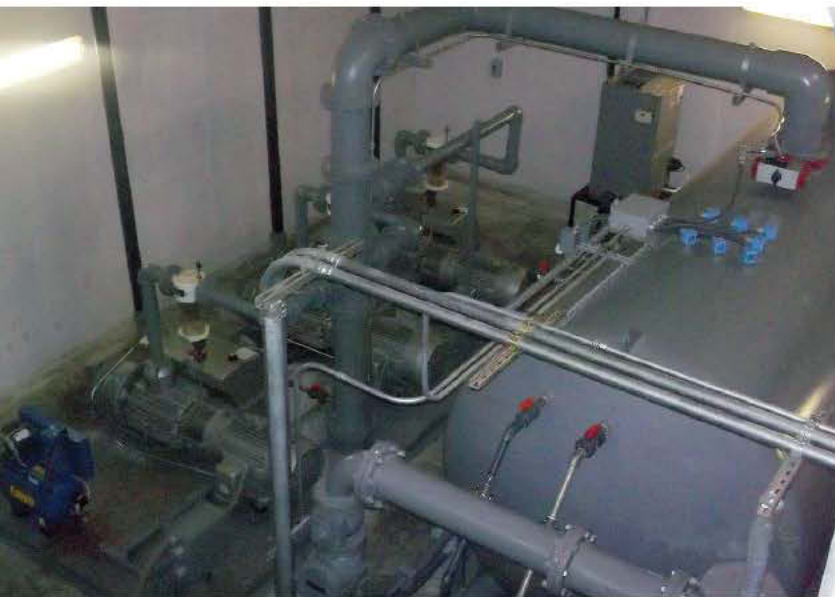
The wastewater is transported directly to the vacuum station, which consists of vacuum pumps, a vacuum reservoir tank, a wastewater collection tank, two wastewater pumps – a lead pump and a lag pump – and electrical controls.
