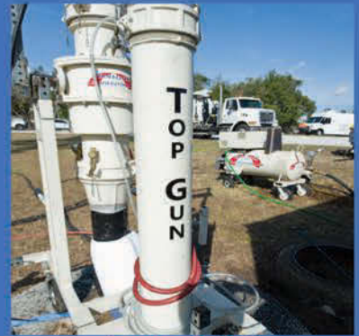
Perma-Main™ Continuous Air Inversion
