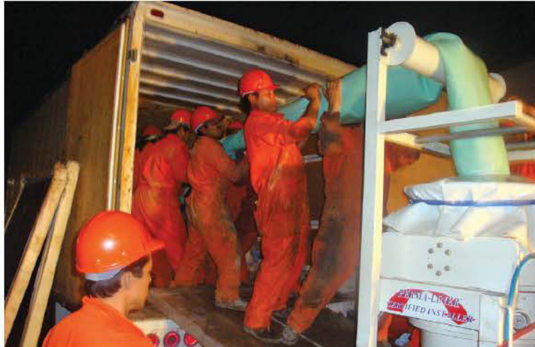
Workers from ACE DuraFlo de Mexico labor to hand-feed the liner onto the tower roller and into the Top Gun diaphragm bladder. (Photo courtesy of ACE DuraFlo de Mexico)
