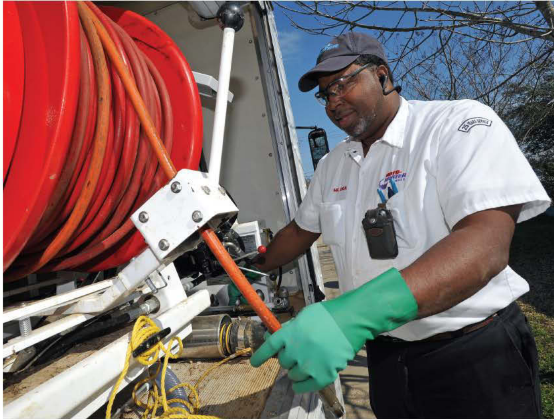
Jackson Roto-Rooter employee Alton Drake sets up the US Jetting equipment that is mounted inside an Isuzu van to waterjet a cleanout at a business in south Jackson.
