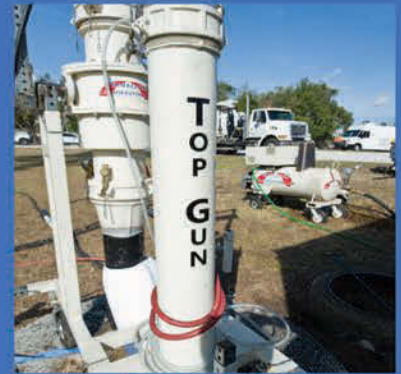
Perma-Main™ Continuous Air Inversion
