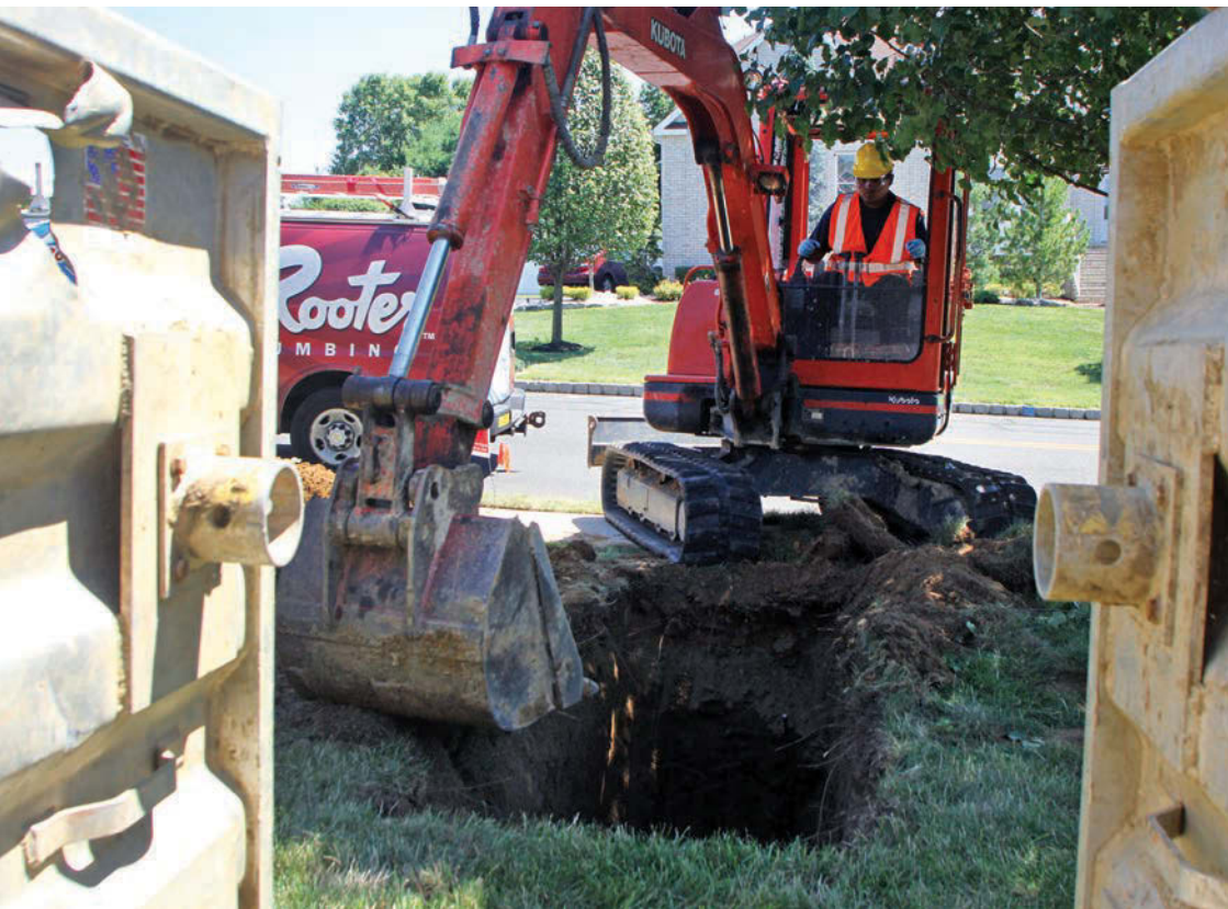
Technician Abaro Garcia uses a Kubota excavator to widen a hole around a broken sewer line.
