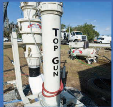
Perma-Main™ Continuous Air Inversion
