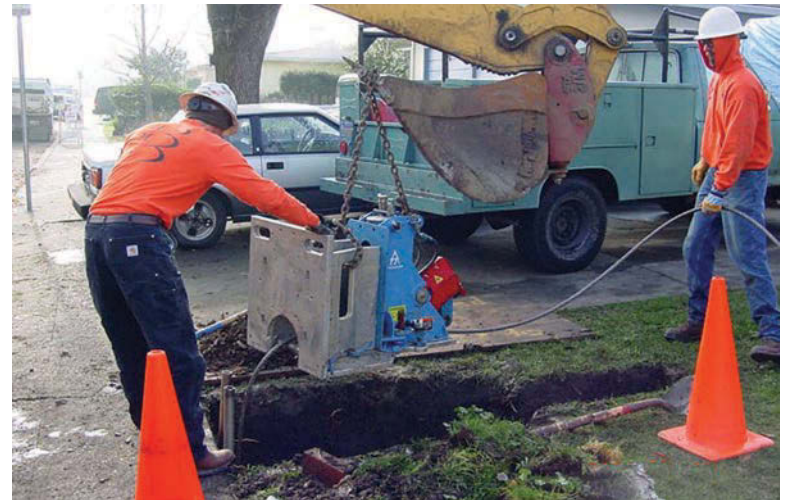
The crew aligns pipe bursting equipment in the extraction pit. (Photo courtesy of IT Technologies, Inc.)
