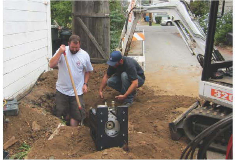
Working in the alley alongside the garage, Rick (left) and Nick Thompson prepare the pulling pit for the PB-40 ram.
