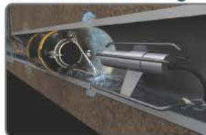
Leaking joint in mainline sewer
