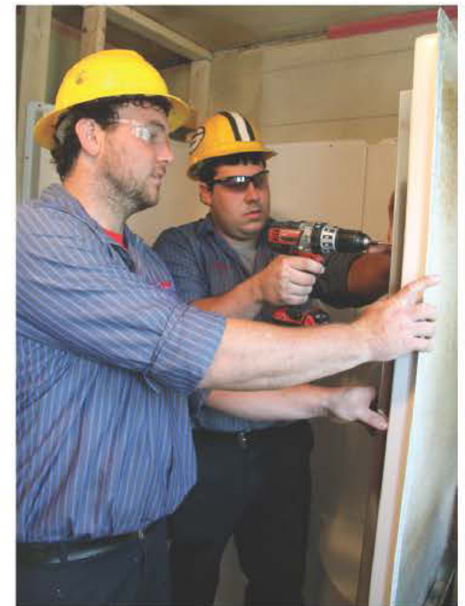
BELOW: Service technicians Jordan Snyder, left, and Parker Smith install an upright shower unit.
