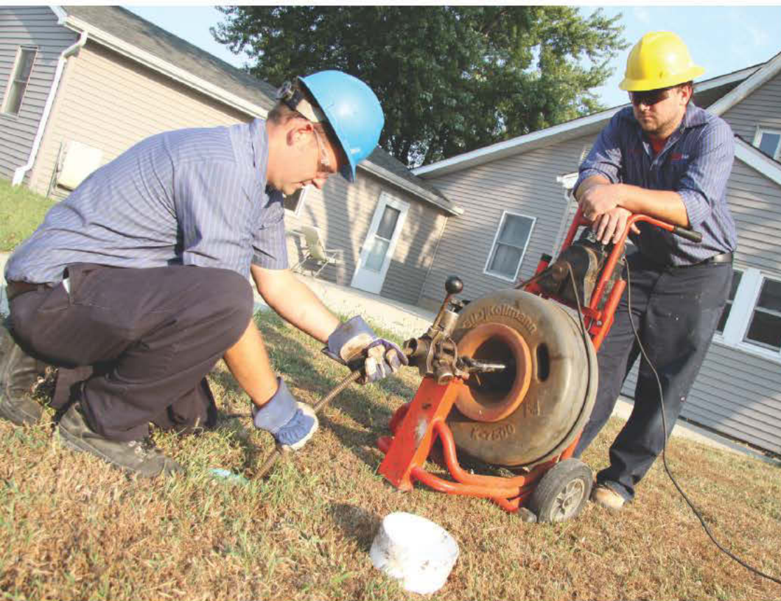
LEFT: Service technician Kurt Ansell, left, gets some assistance from service technician Jordan Snyder while cleaning a sewer lateral using a RIDGID K-7500 mainline cleaner at a residential home in Staunton, Ill.
