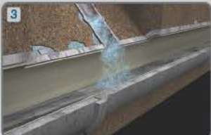
Continues to leak in annular space
