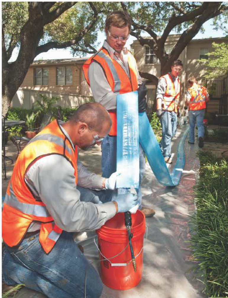
Clayton Vitellaro, Casey Van Cleave and Chad Montgomery prepare the Nu Flow casing.
