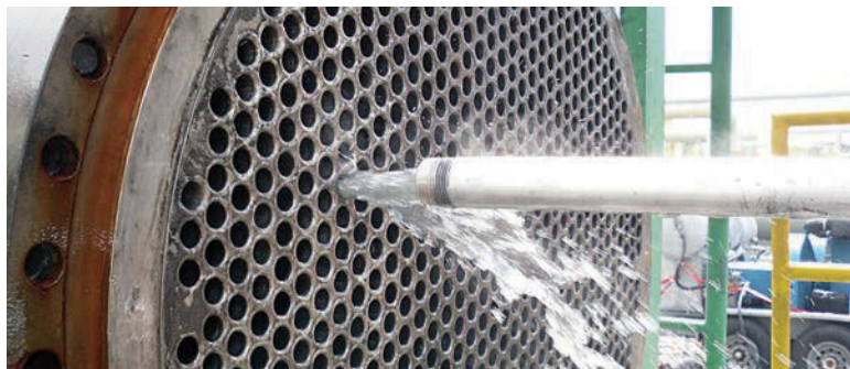
The Armadillo industrial cleaning system jets out a 55-foot-long, 1-inch diameter tube on a heat exchanger at a crude-oil processing facility in Alaska.
