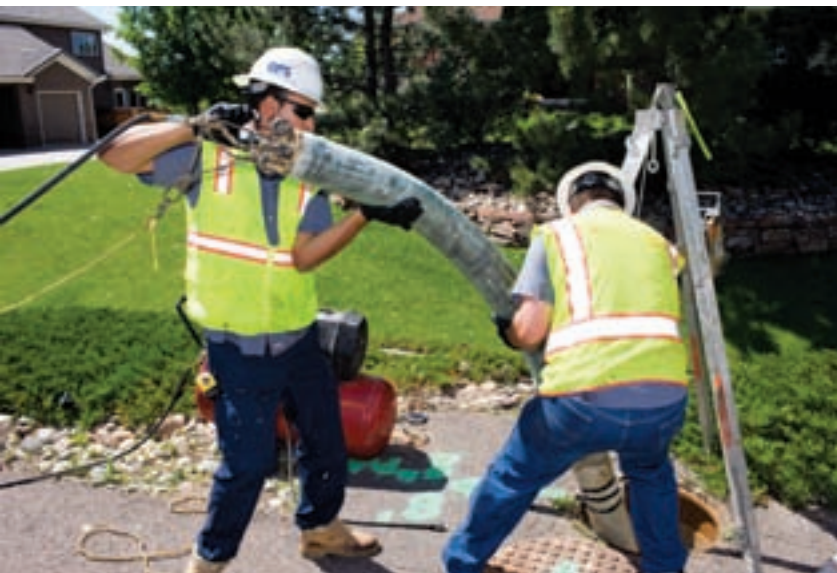
Lead operator Luis Marin, left, and superintendent/project manager Monty Hill get the pipe inserted and ready for CIPP lining repair.
