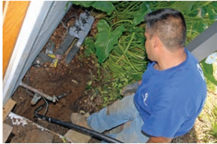
Technician Atanacio Francisco from Quality First Plumbing helps guide the 1-inch HDPE replacement pipe into the pit at the start of the pull. The ACME coupling attaching the pipe to the rear of the bursting head is visible just past the spigot. (Photos courtesy of TRIC Tools)
