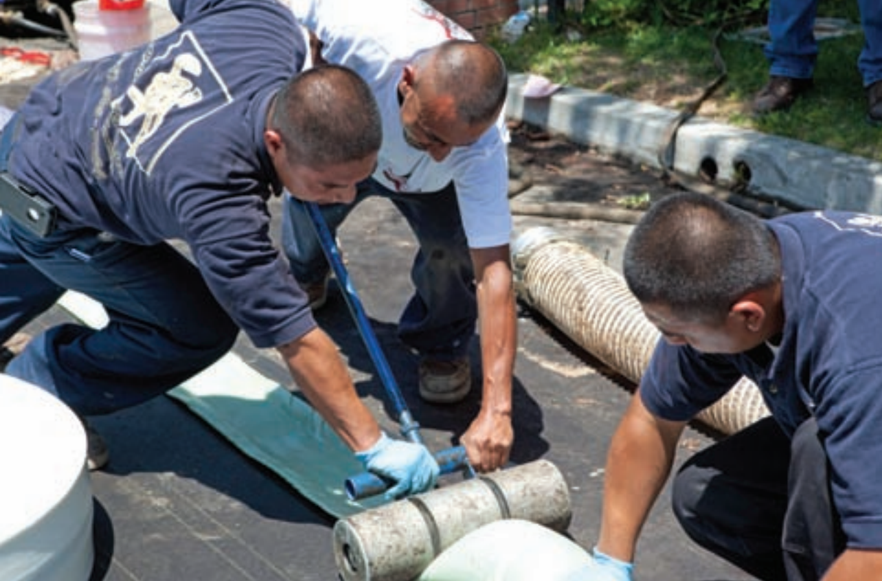
Once the liner is impregnated with the chemicals, it is ready to be deployed. Pipe bursting operator Edwin Azucar (left) and plumber technician Julio Lopez help pipe bursting operator Carlos Aguilar.
