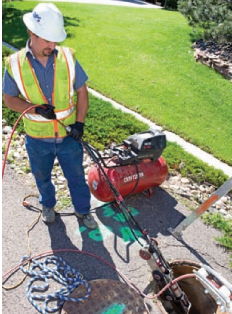
Superintendent Monty Hill lowers the Aries Badger camera into the manhole for inspection.
