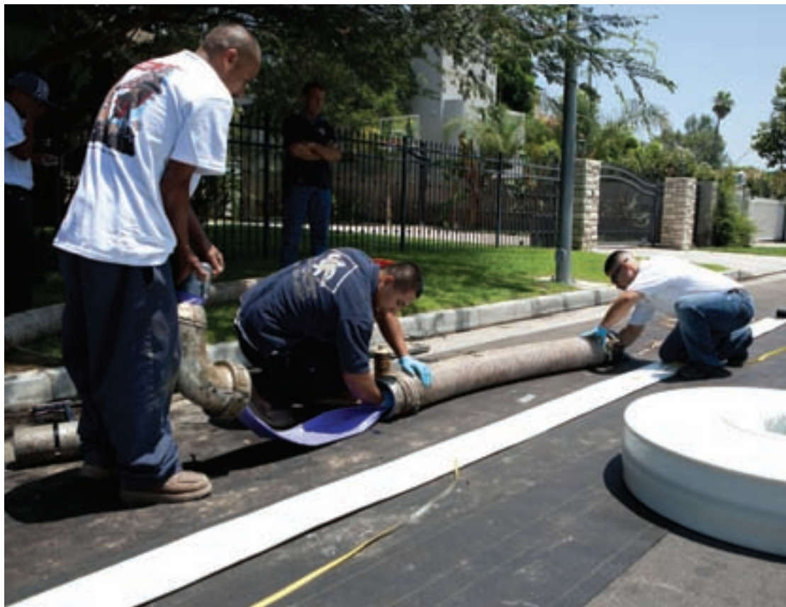
A pipe is readied for lining by Julio Lopez, plumber technician (left); Carlos Aguilar, pipe bursting operator; and Juan Carlos Garcia, owner.
