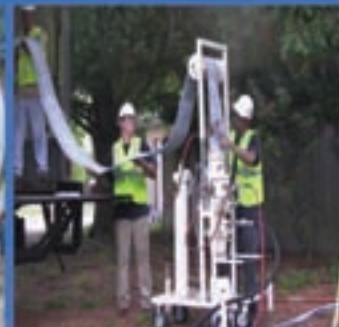
Perma-Main™ Continuous Air Inversion
