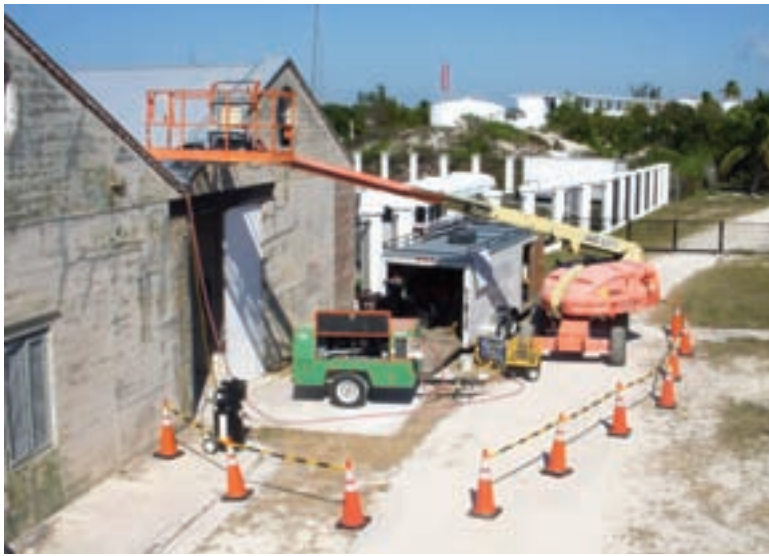
The 20-foot MaxTrailer, telescopic boom lift, air compressors, and generator are barricaded behind cones with safety rails.
