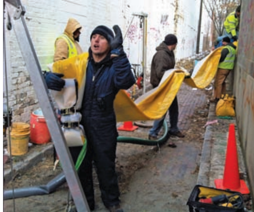
Workers from Flynn Brothers Contracting move a liner to a manhole in an alley. The nose of the liner is folded back over a nylon choker with a cable attachment and secured with two nylon straps. (Photos courtesy of Metropolitan Sewer District of Greater Cincinnati)
