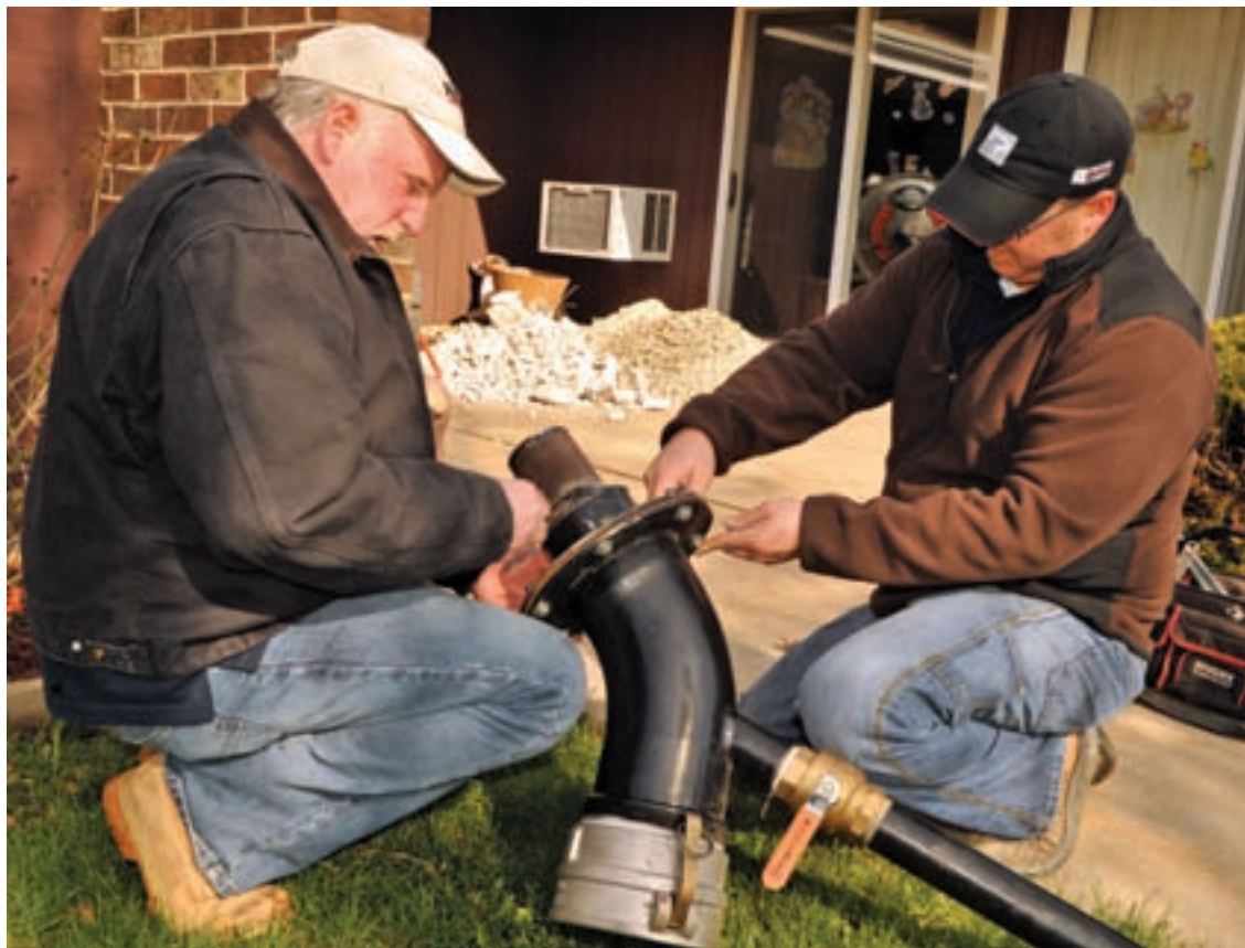
Jeff and Jake Saltzman do preliminary work for a residential pipe lining job.
