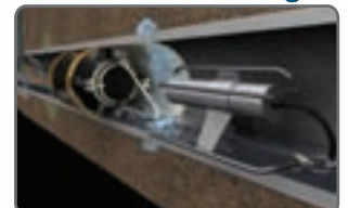
Leaking joint in mainline sewer
