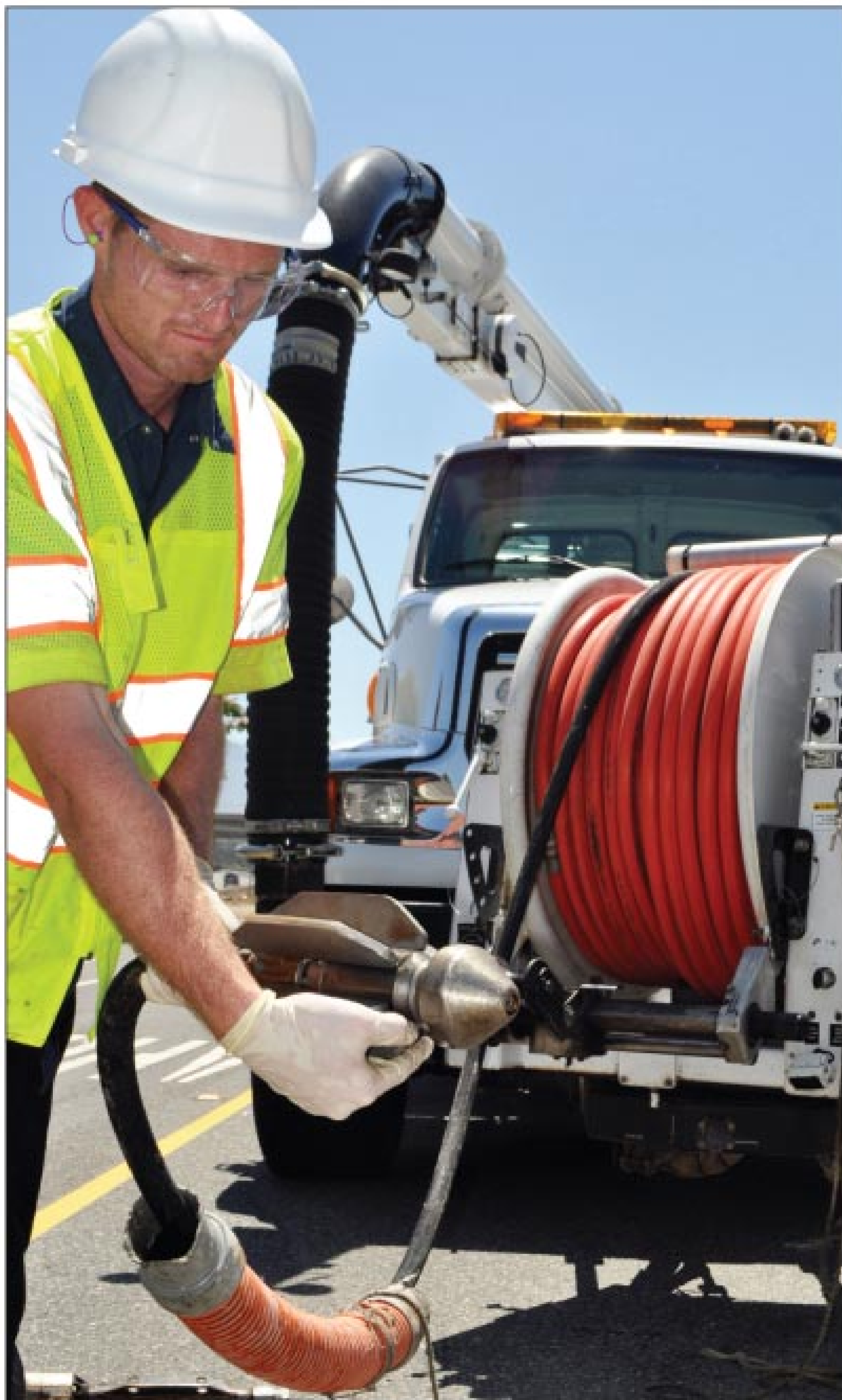
Combination truck operator Austin Welch attaches a nozzle to the jetter hose in preparation for a large-diameter cleaning operation.
