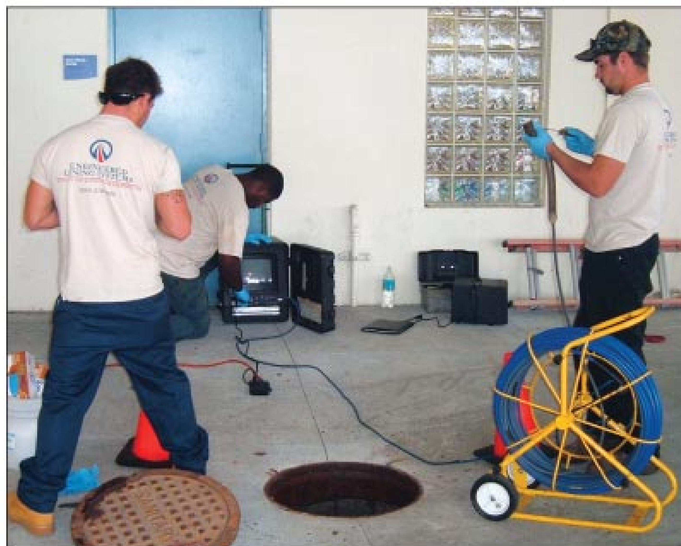
James Macko, Mikal Biegner, and Dennis Gaskins of Engineered Lining Systems set up a camera system from Ratech Electronics to inspect the 6-inch line serving the kitchen.
