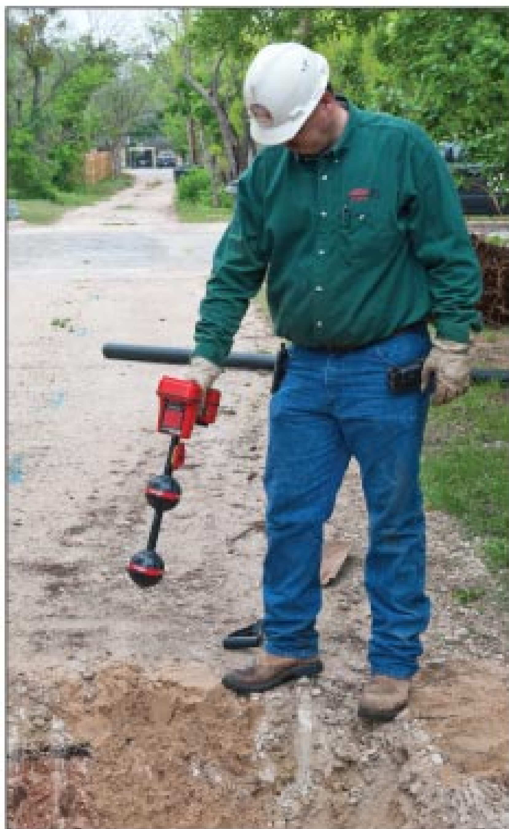
Plumbing technician Mark Hartanft pinpoints a sewer line with the aid of a Scout locator from RIDGID that detects the camera deep in the sewer line.
