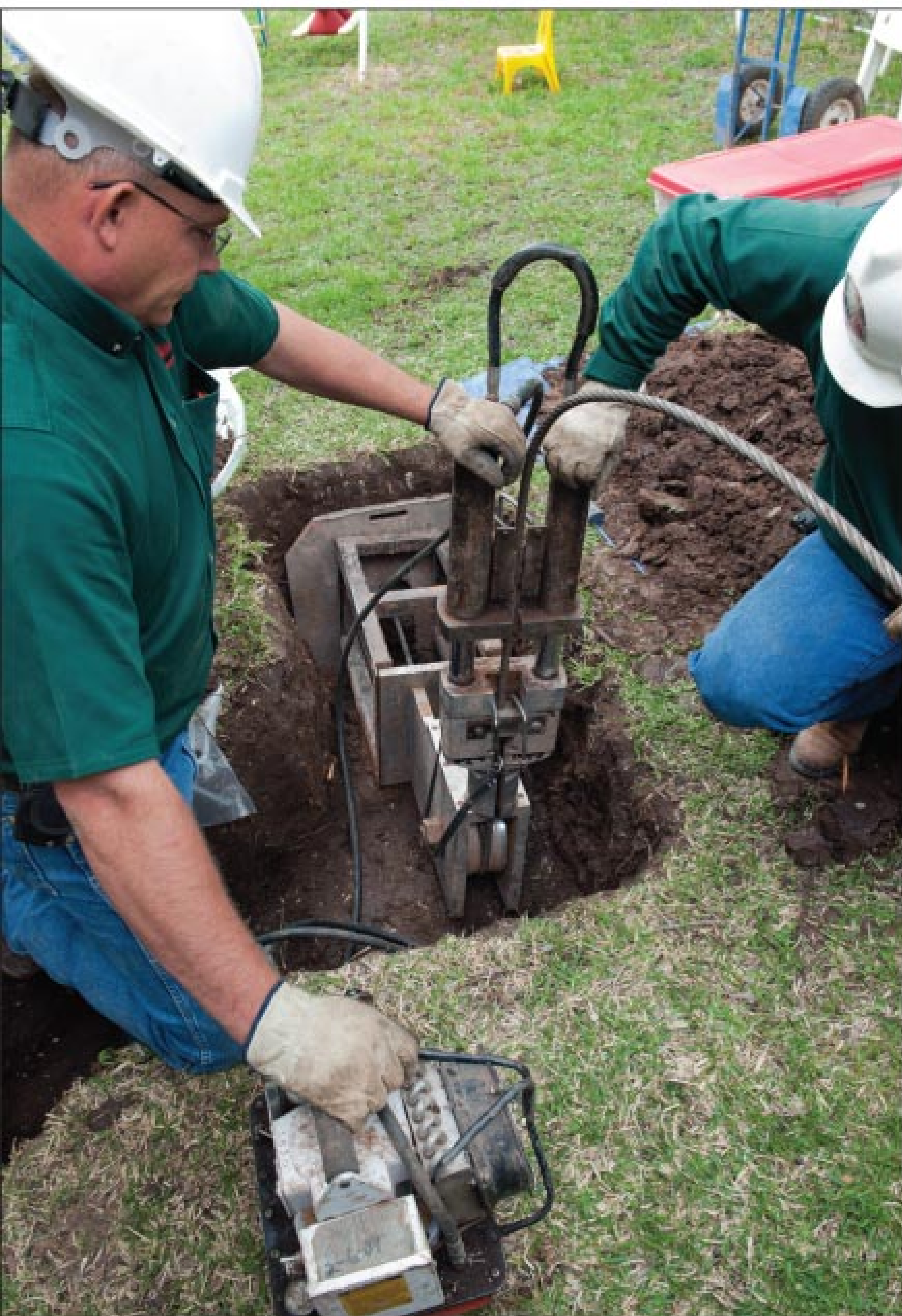
A pipe bursting system from TRIC Tools is a key tool in the kit for Midway Plumbing. Shown placing the bursting unit are apprentice Ronnie Moore and plumbing technician Mark Hartanft.
