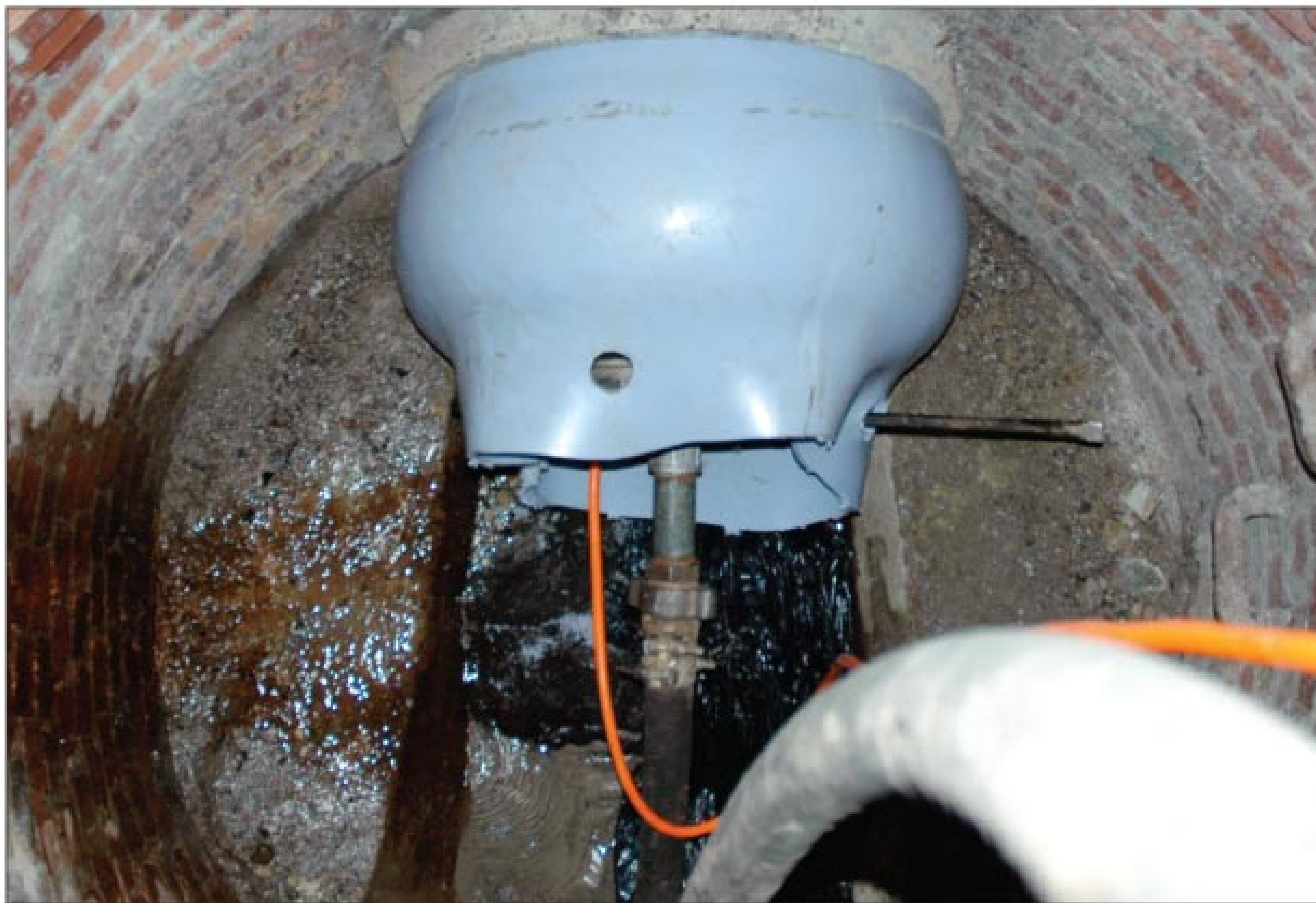
The sewer plug flares out the end of the liner, locking it in place against the manhole and preventing inflow and infiltration.
