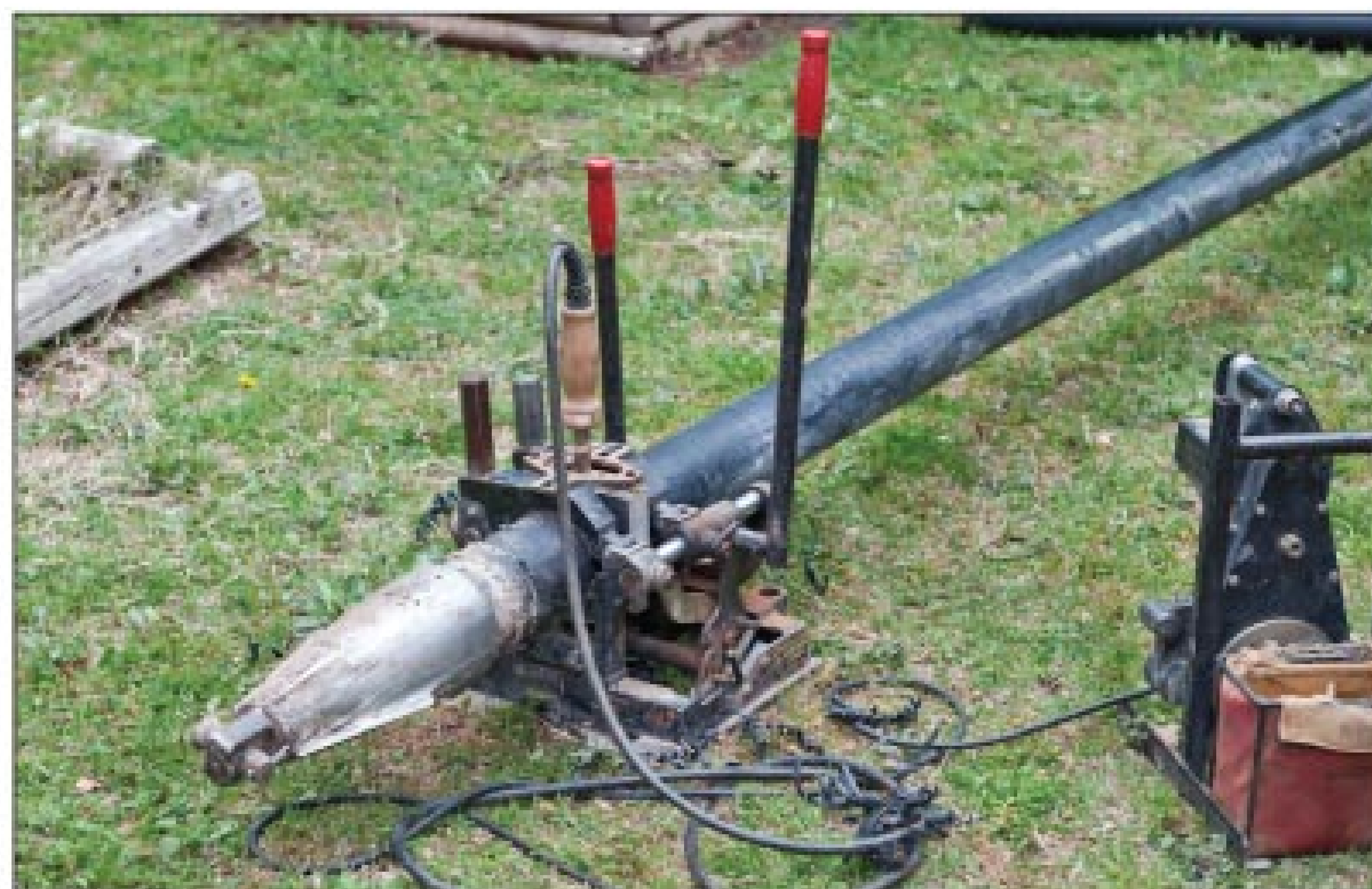
The bursting head pulls fused sections of polyethylene pipe through the old pipe being replaced.
