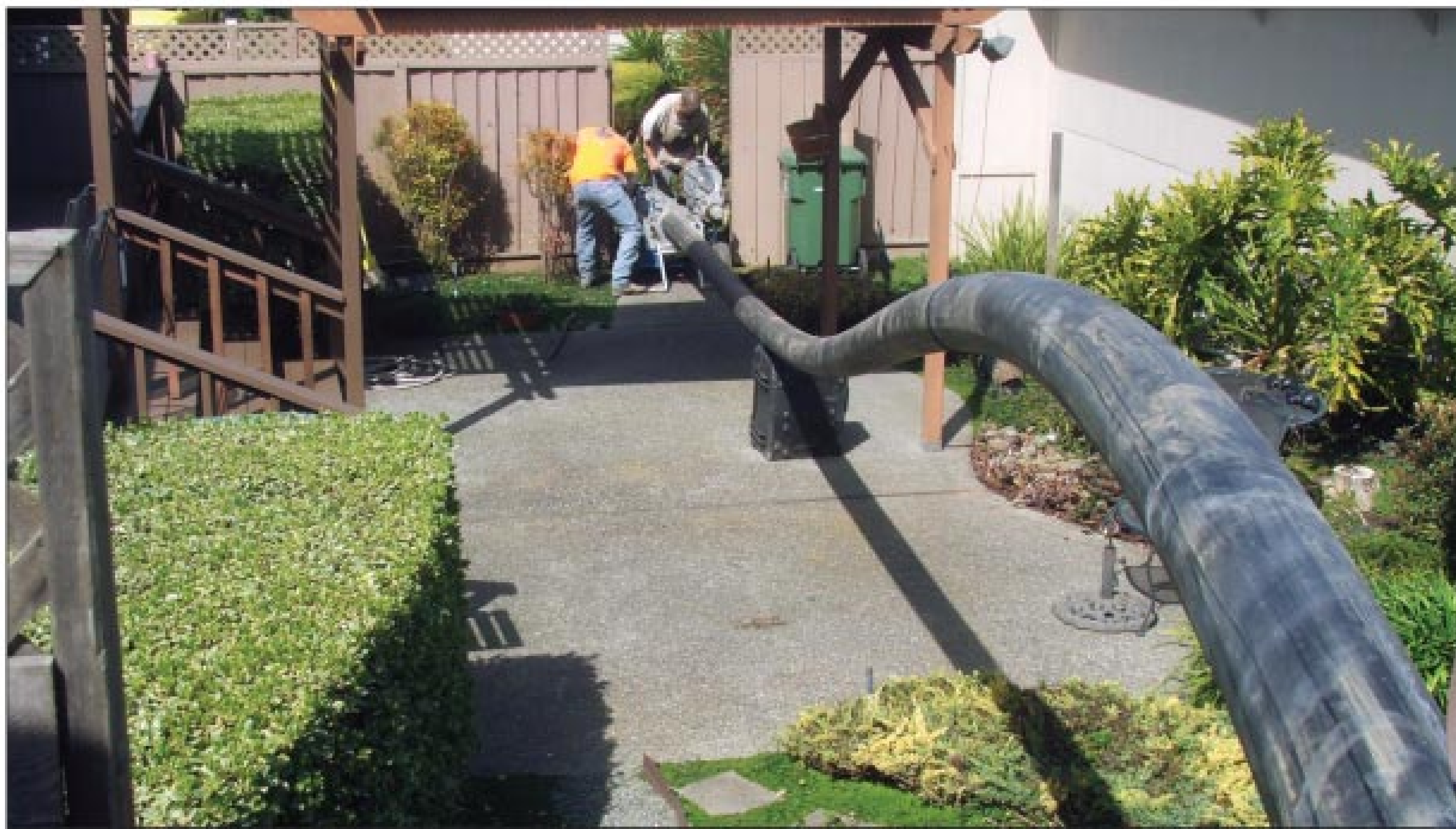
John Mahana and Jim Voudy fuse a 40-foot section of HDPE pipe. A gate in a privacy fence provided the space for the fusion machine.
