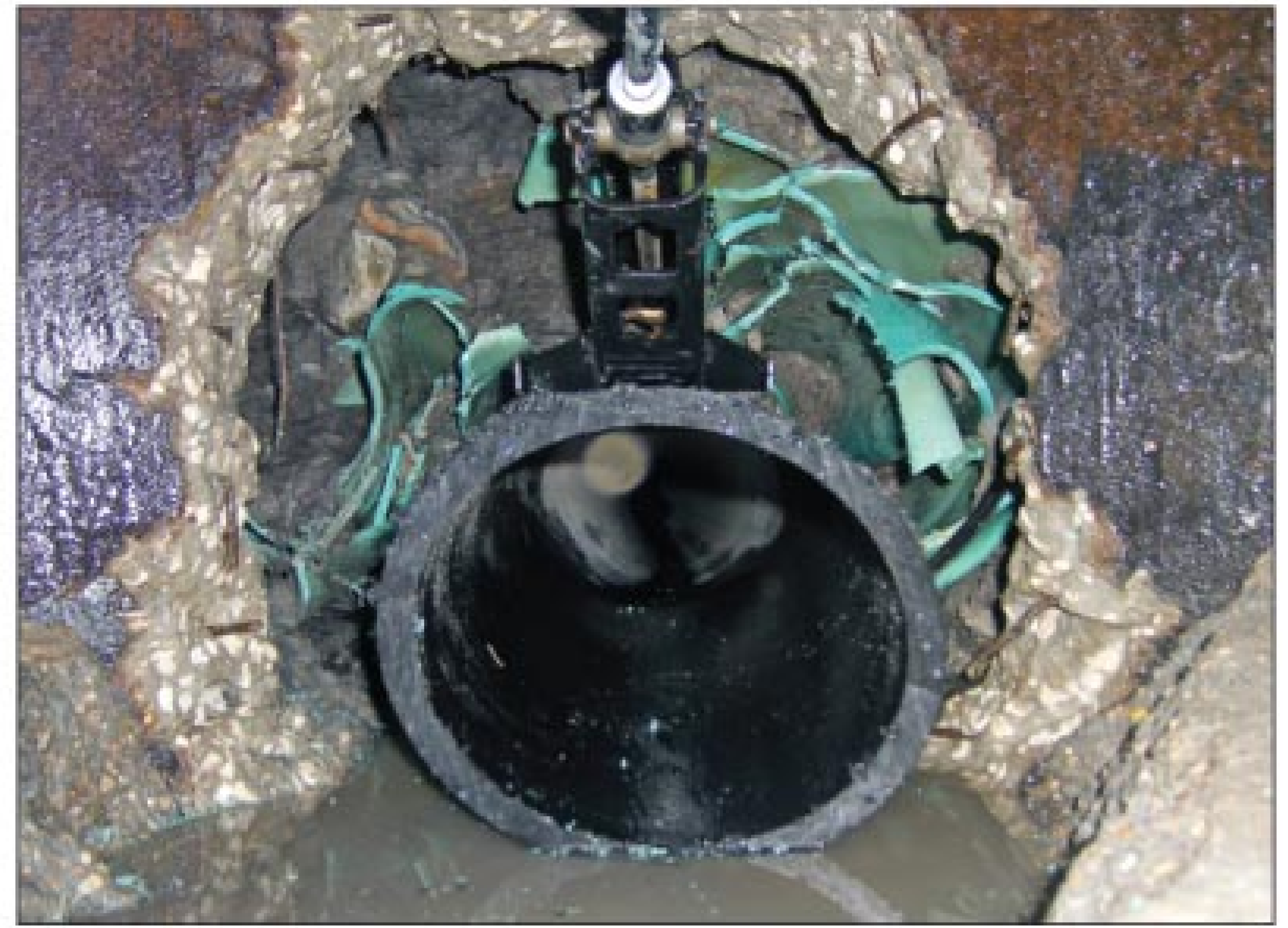
Workers used a scissor jack in an attempt to free the tightly packed telescoping shards of plastic pipe. Backed up water is just beginning to spill out of the black pipe.
