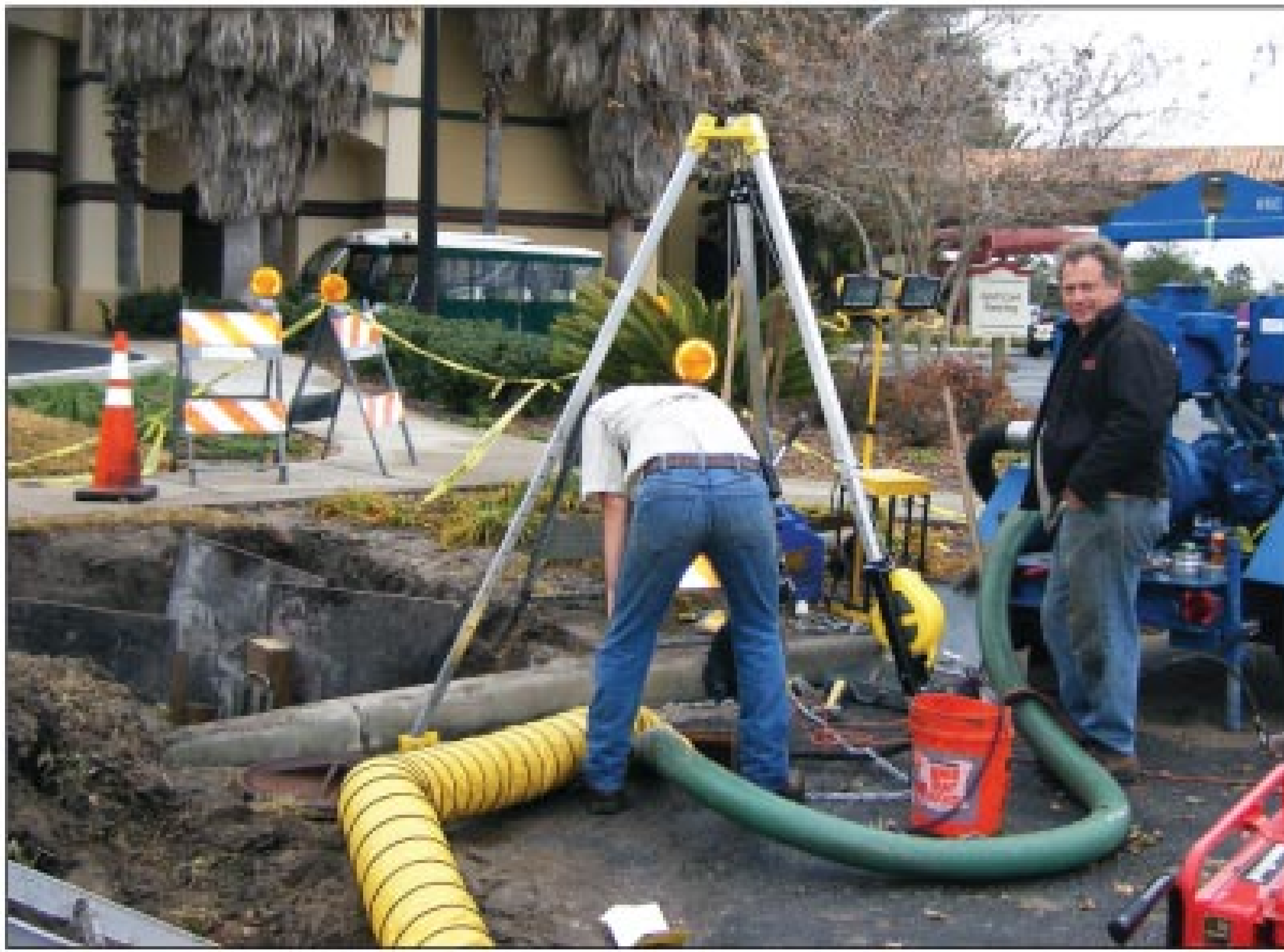
The setup at the center entrance pit included the bursting head, bypass pumps and hoses, and the attendant/entry supervisor observing the man working in the pit.
