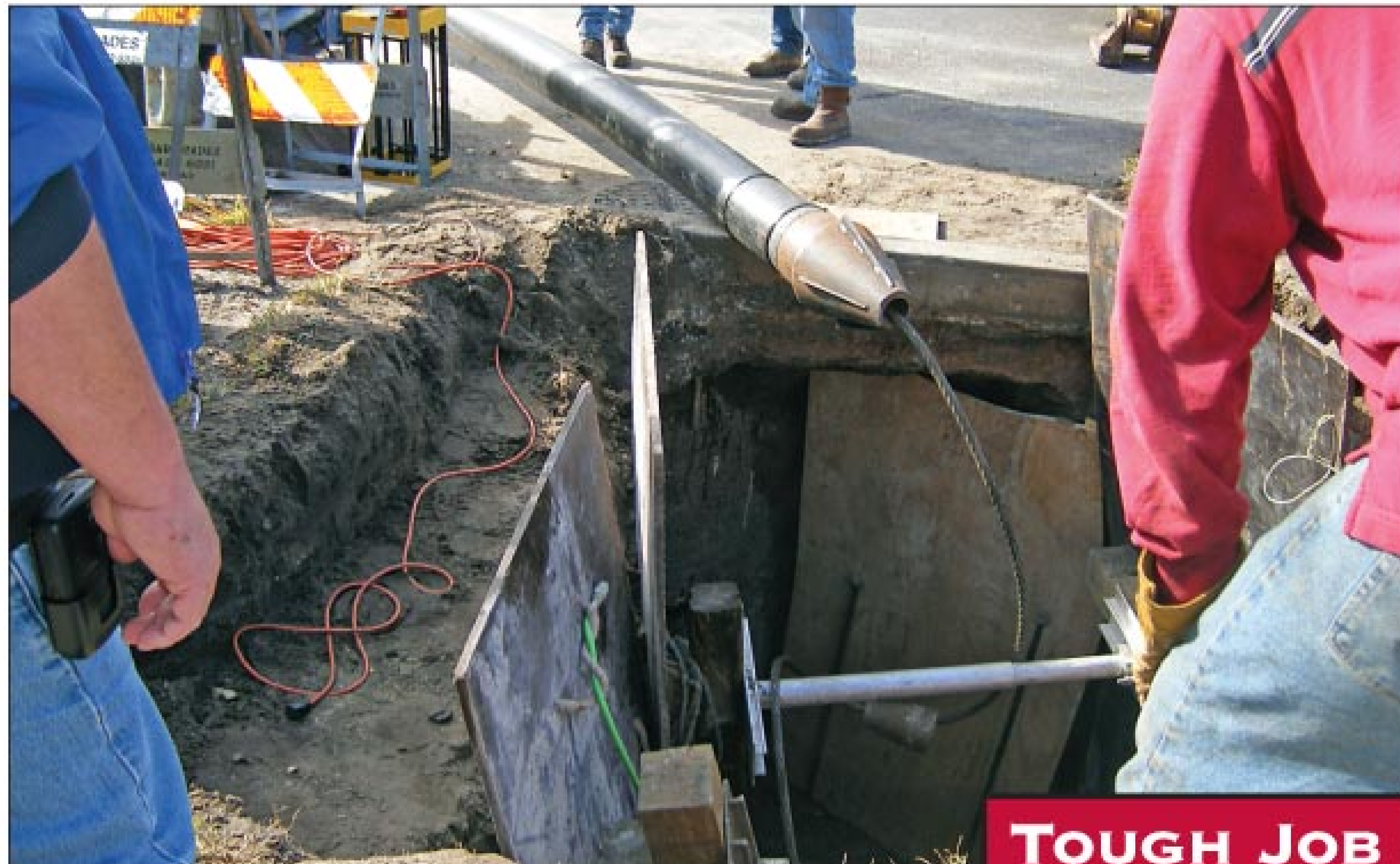
The 8-inch bursting head begins its descent into the entrance pit in the median strip. Note the slitting fins on the head and service collar. (Photos courtesy of Omni Eye Inc.)
