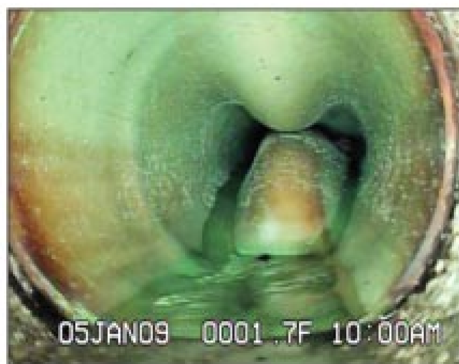
Video capture of the collapsed 8-inch SDR-35 PVC gravity sewer 1.7 feet upstream of the center manhole. (Courtesy of CH2M Hill)
