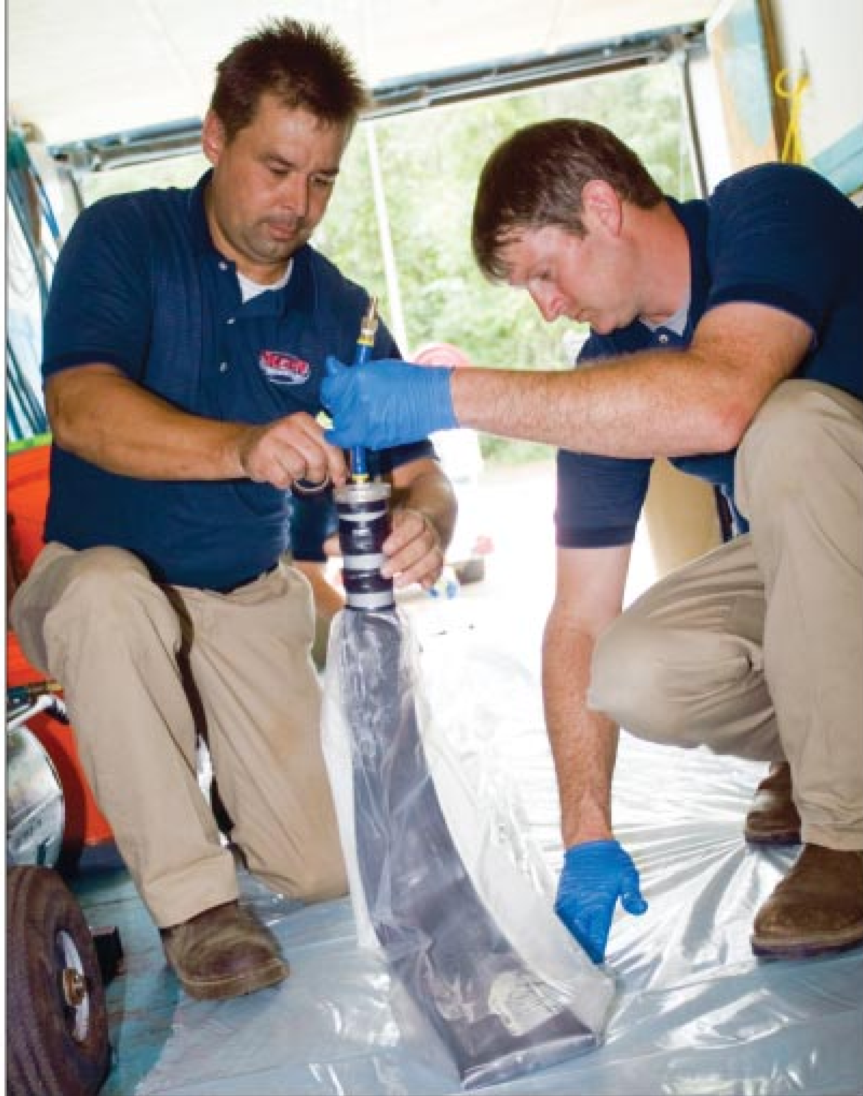
Technicians Frank Romig (left) and Jason Vanlandingham prepare a pipe liner for installation in Skeen Plumbing's 24-foot liner trailer on a work site in Jackson, Miss. (Photography by Ron Blaylock)
