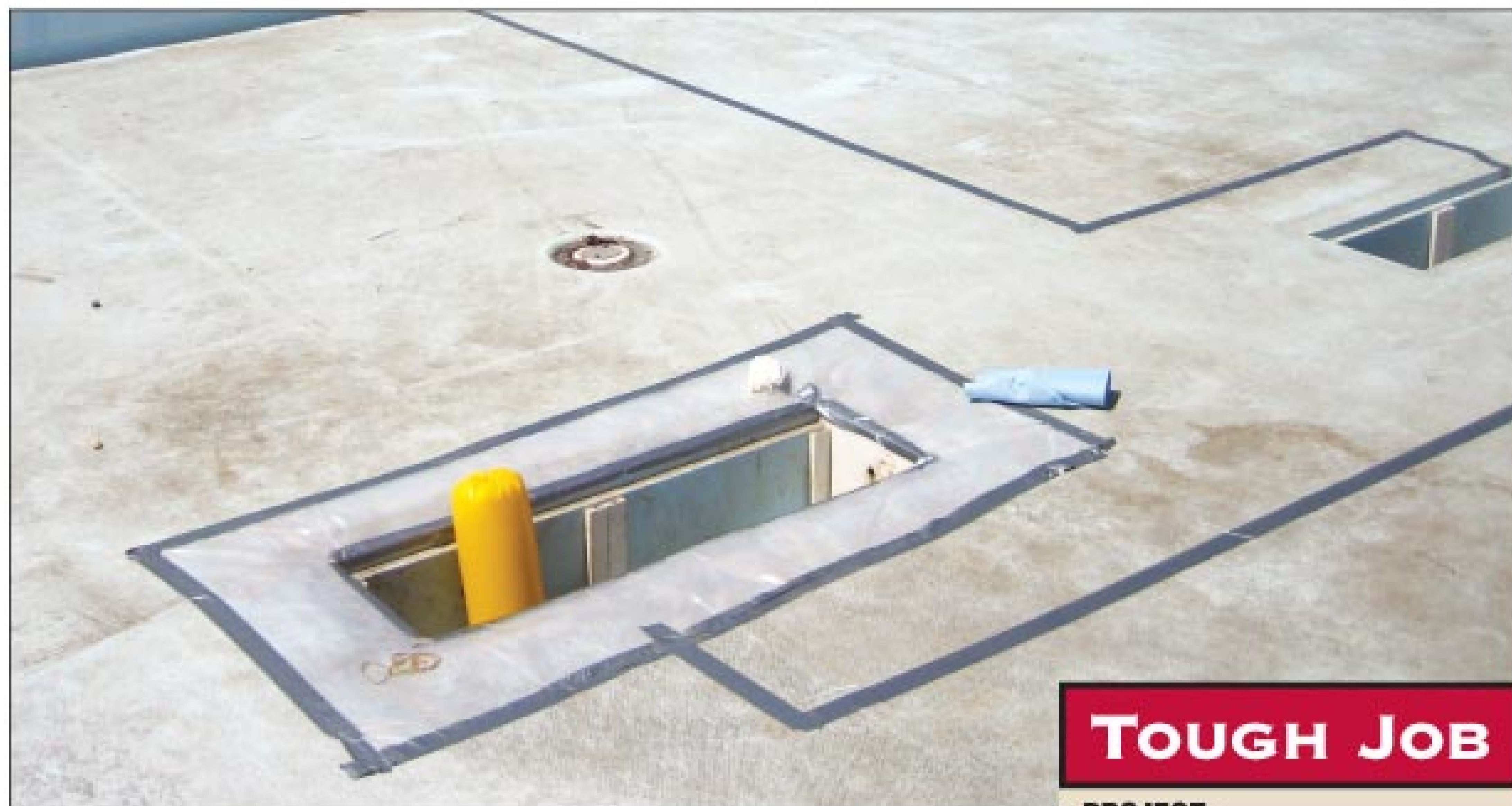
The calibration tube, inflated to 8 psi, rises through the pool drain. The plastic sheet around it is designed to catch any stray drops of resin. The gray duct tape represents the route of the drain line. (Photography by Mary R. Christen)
