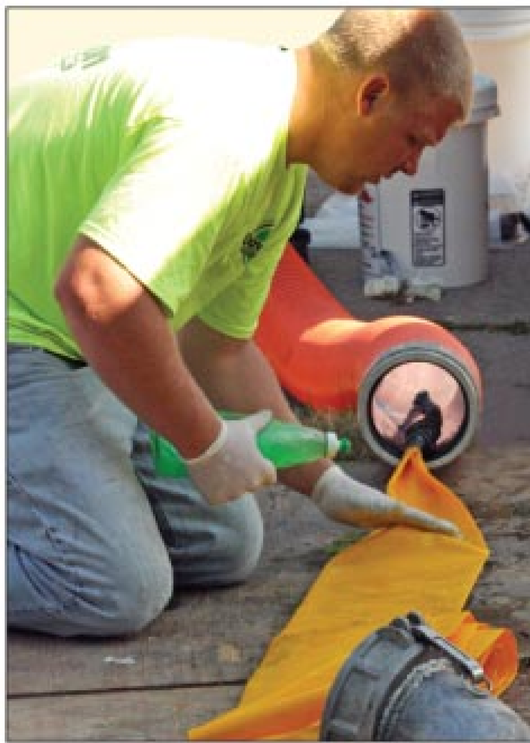
Scott Veal lubricates the calibration tube with a mixture of liquid dishwashing soap and water before shooting it into the liner.
