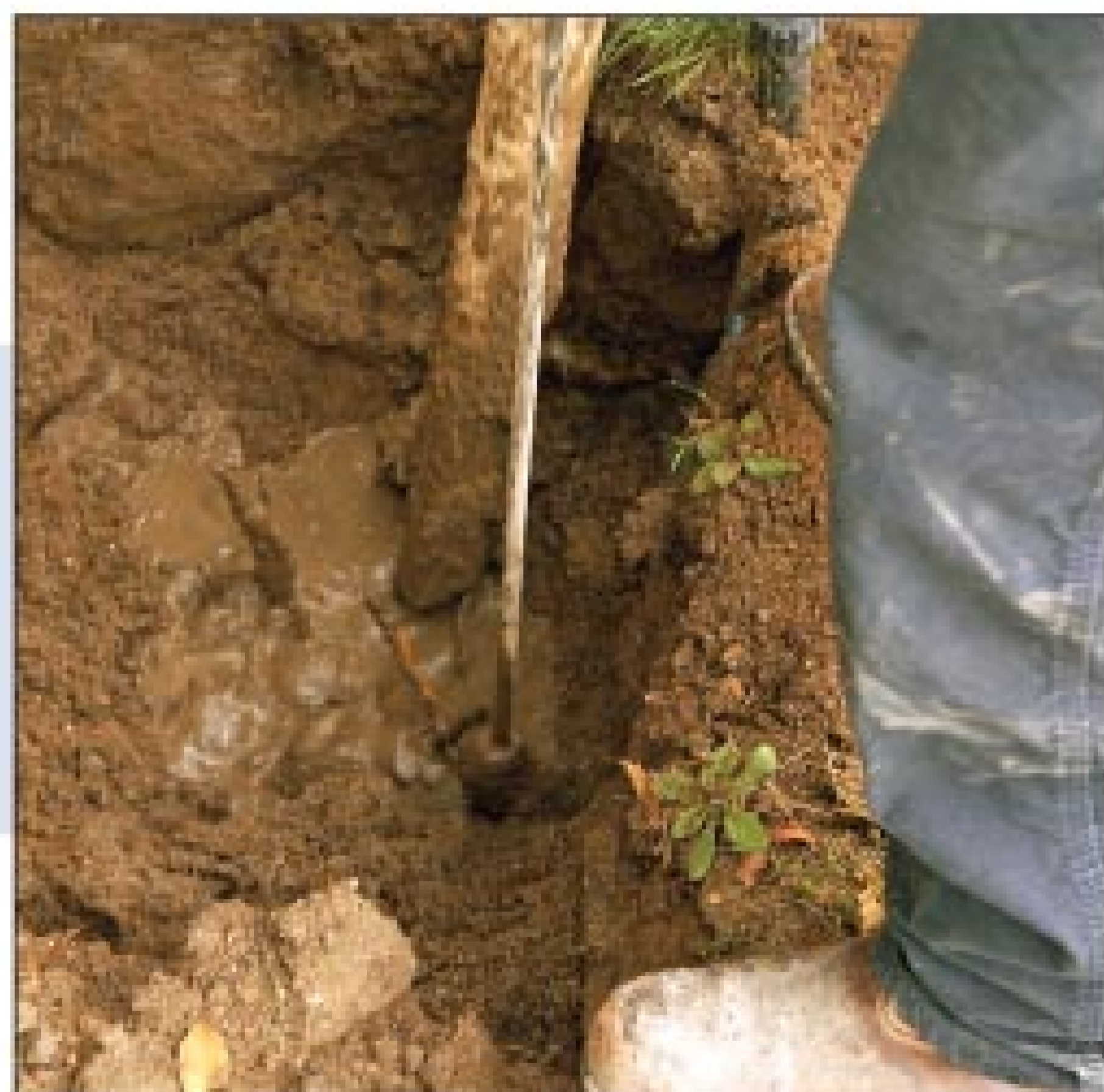
Troy Bunn and Peter Gomalka use a Ring-O-Matic hydroexcavating system to access a broken pipe that caused water to leak into a homeowner's basement. (Photography by Jon Asp)
