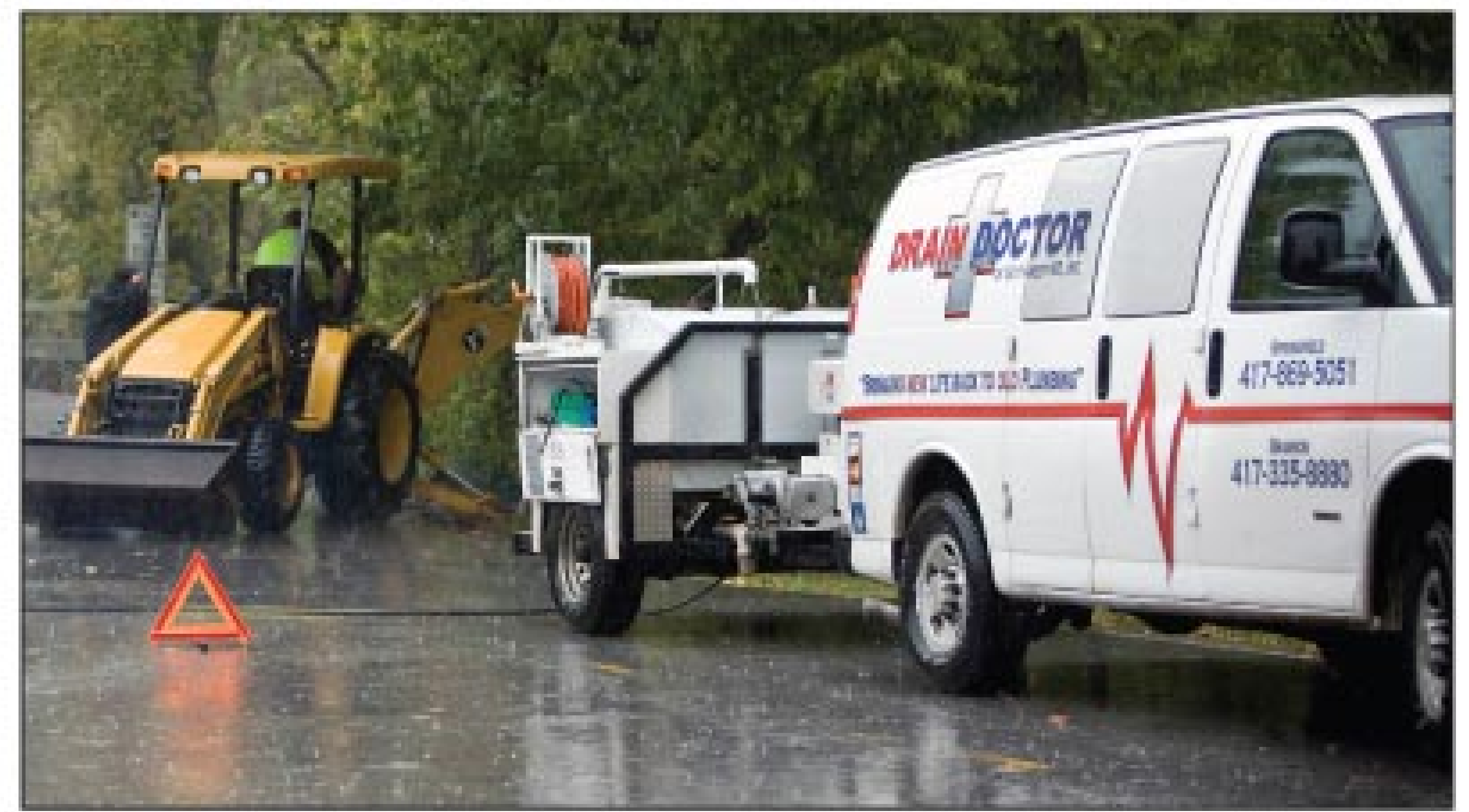
The Drain Doctor van and Model 4018 trailer-mounted waterjetter from US Jetting at the site of a culvert repair.
