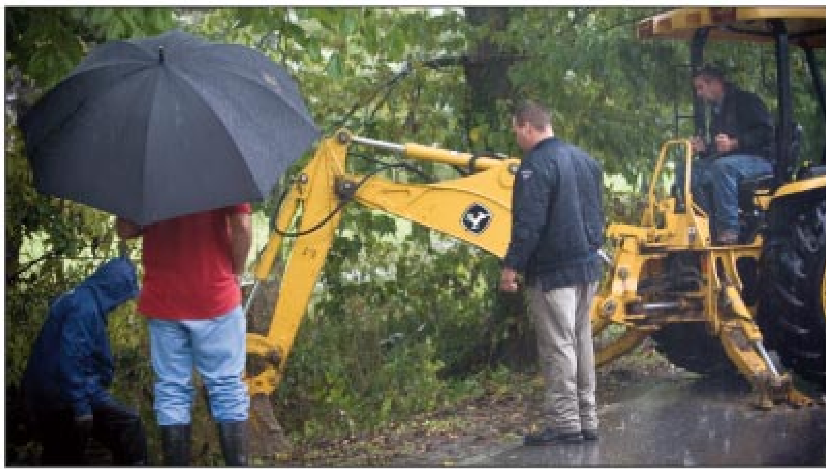
Three companies with different specialties attack a repair job on a damaged stormwater culvert. On the backhoe is Josh Nelson, owner of Nelson Excavating. In the hooded jacket is Tim Smith, owner of S&S Pumping. With the umbrella is Eric Engel, owner of Riverside Inn, and next to the backhoe is Fred Stewart, owner of Drain Doctor.
