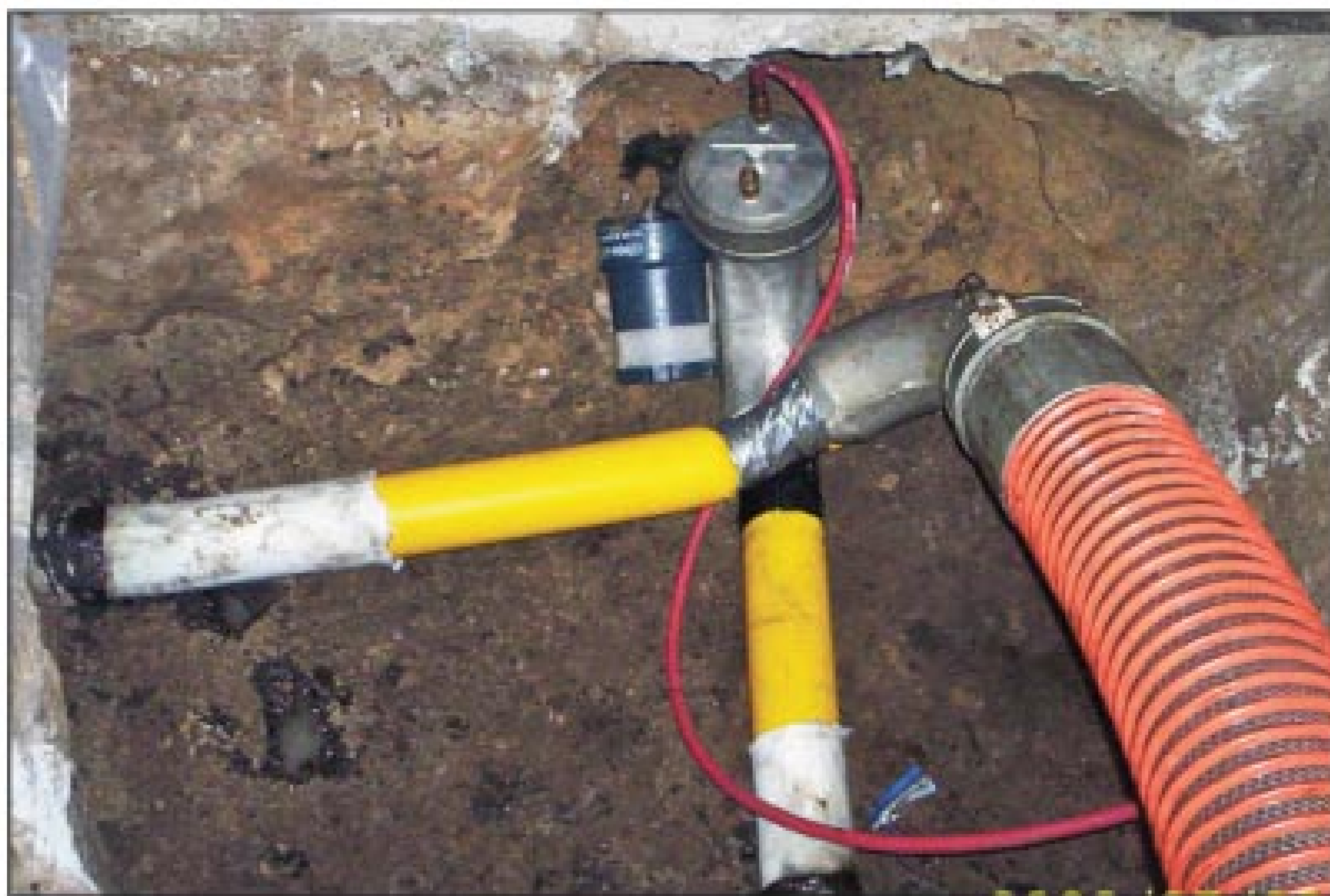
Workers lined in both directions from the access point in the 184-foot-long 4-inch pipe, shooting 101-foot and 83-foot liners.
