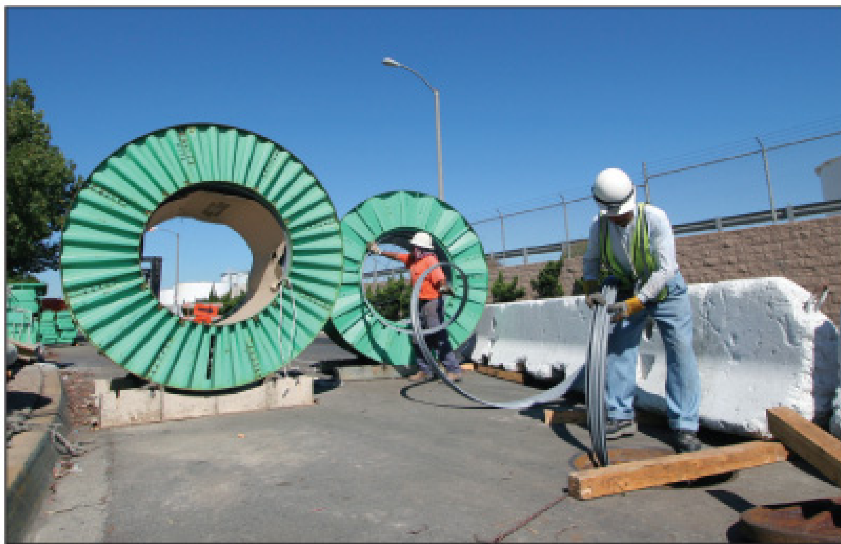
The liner is delivered on rolls and deployed into the manhole to a hydraulic winding machine.
