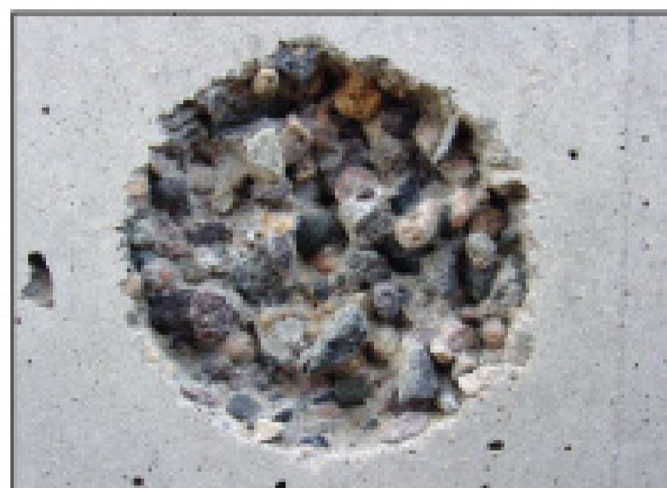
The 40,000-psi/4-gpm waterblast equipment cut a series of impressions in the walls' concrete surfaces.
