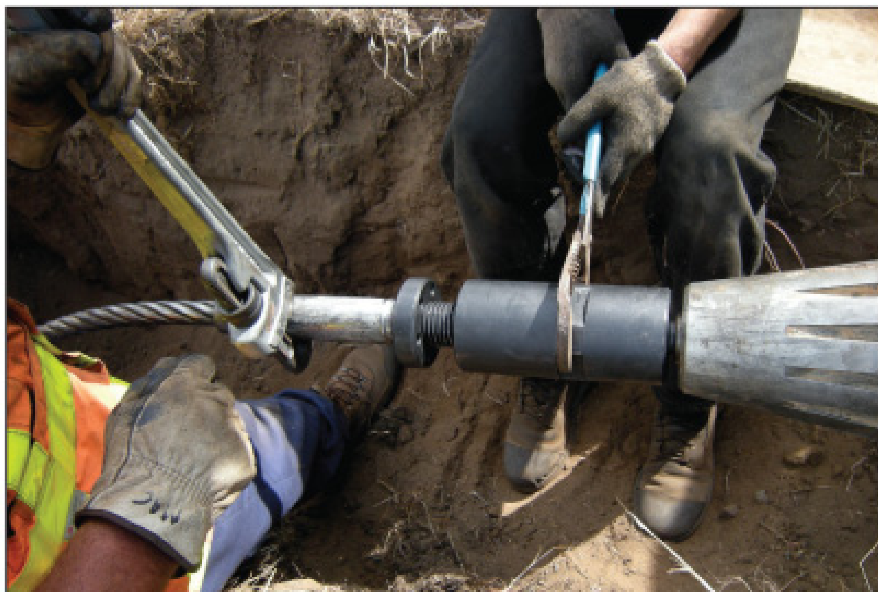
While assistant Ian Hom grasps the treaded stud on the cable with a pipe wrench to prevent it from turning, colleague John Rafferty attaches the cable adapter to the Unified Force head using a channel lock wrench.
