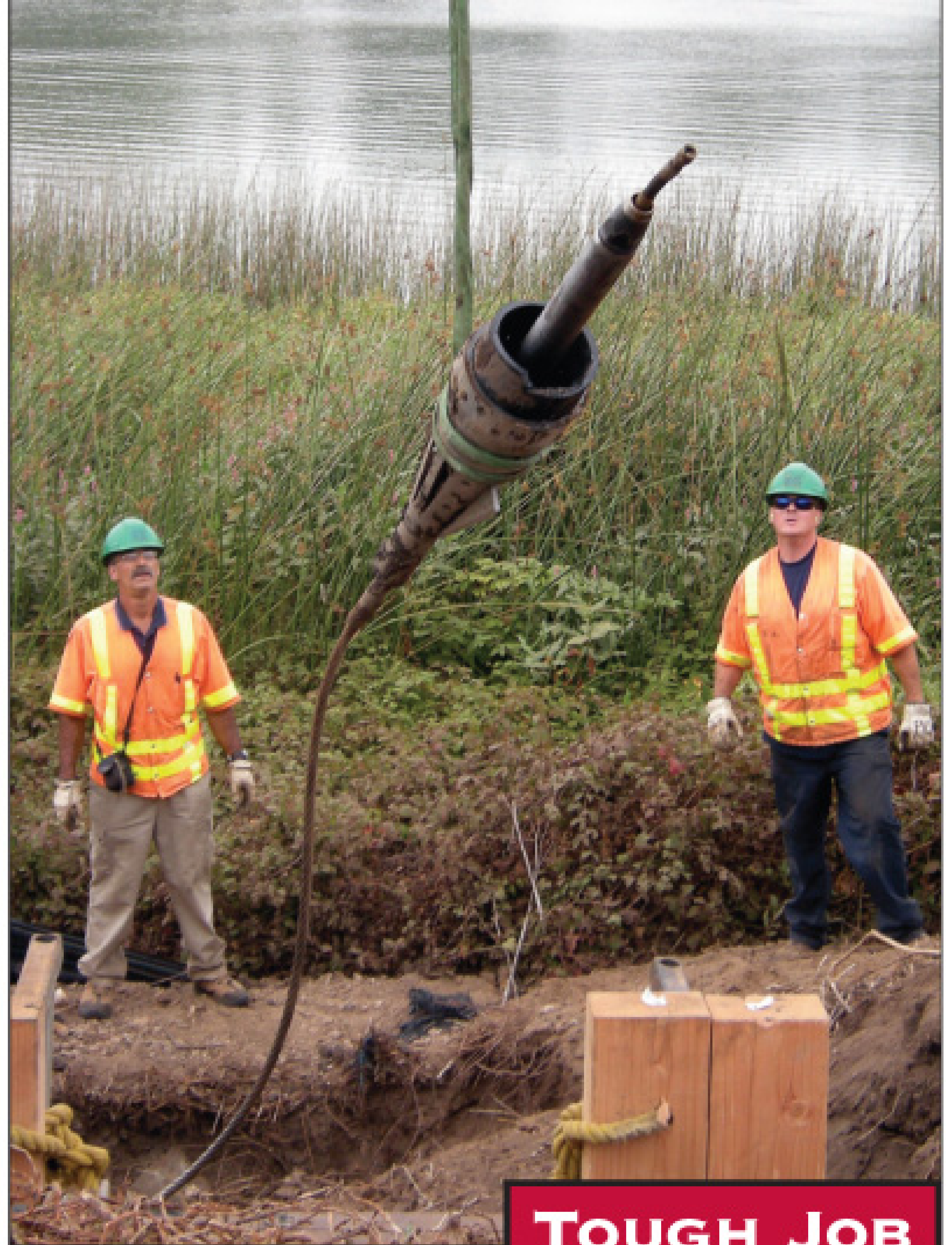
Crew foreman Bob Donati (left) and TRIC Tools assistant Ian Hom watch as a backhoe extracts the fluted head, expansion skirt, and piercing tool from the pulling pit. (Photos courtesy of TRIC Tools Inc.)
