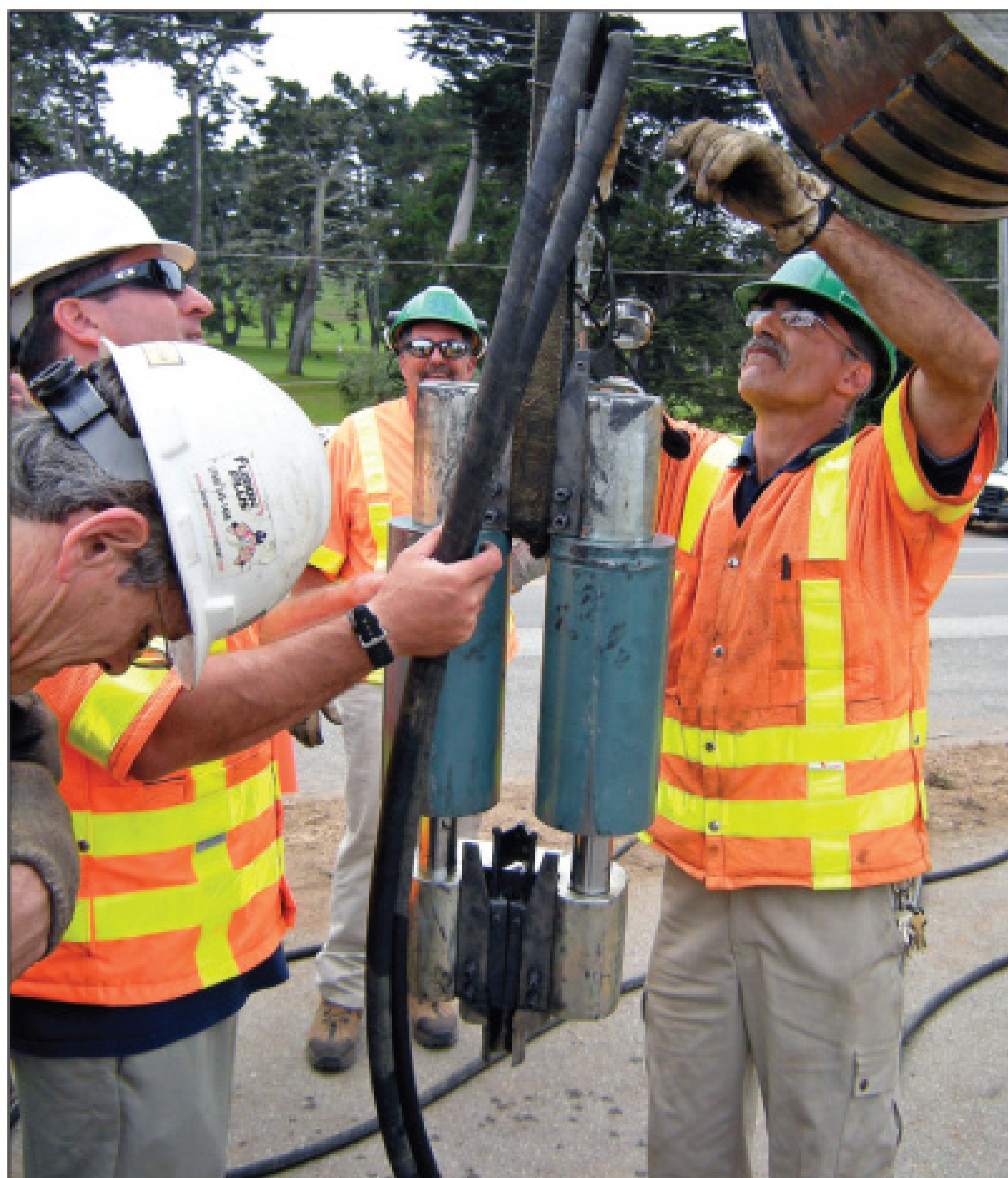
Crew foreman Bob Donati (right) and Tom Piccolotti (left), Daly City wastewater director of operations, attach the ram to the backhoe bucket. TRIC technical field director John Rafferty (foreground) and assistant Ian Hom (background) act as spotters.
