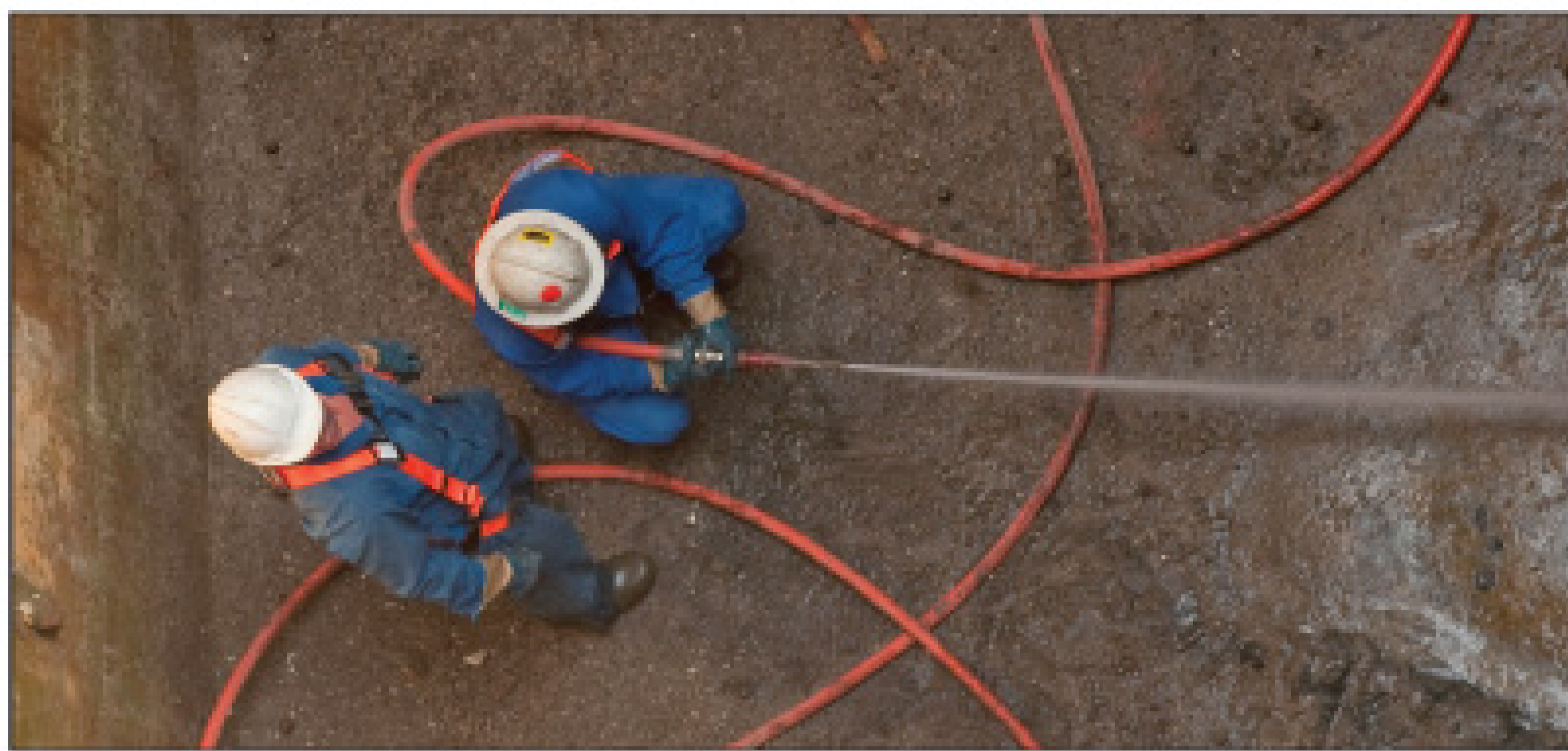
Luke McGill and Josh Weightman clean a settling pit that was used in an old coal-fired power plant.
