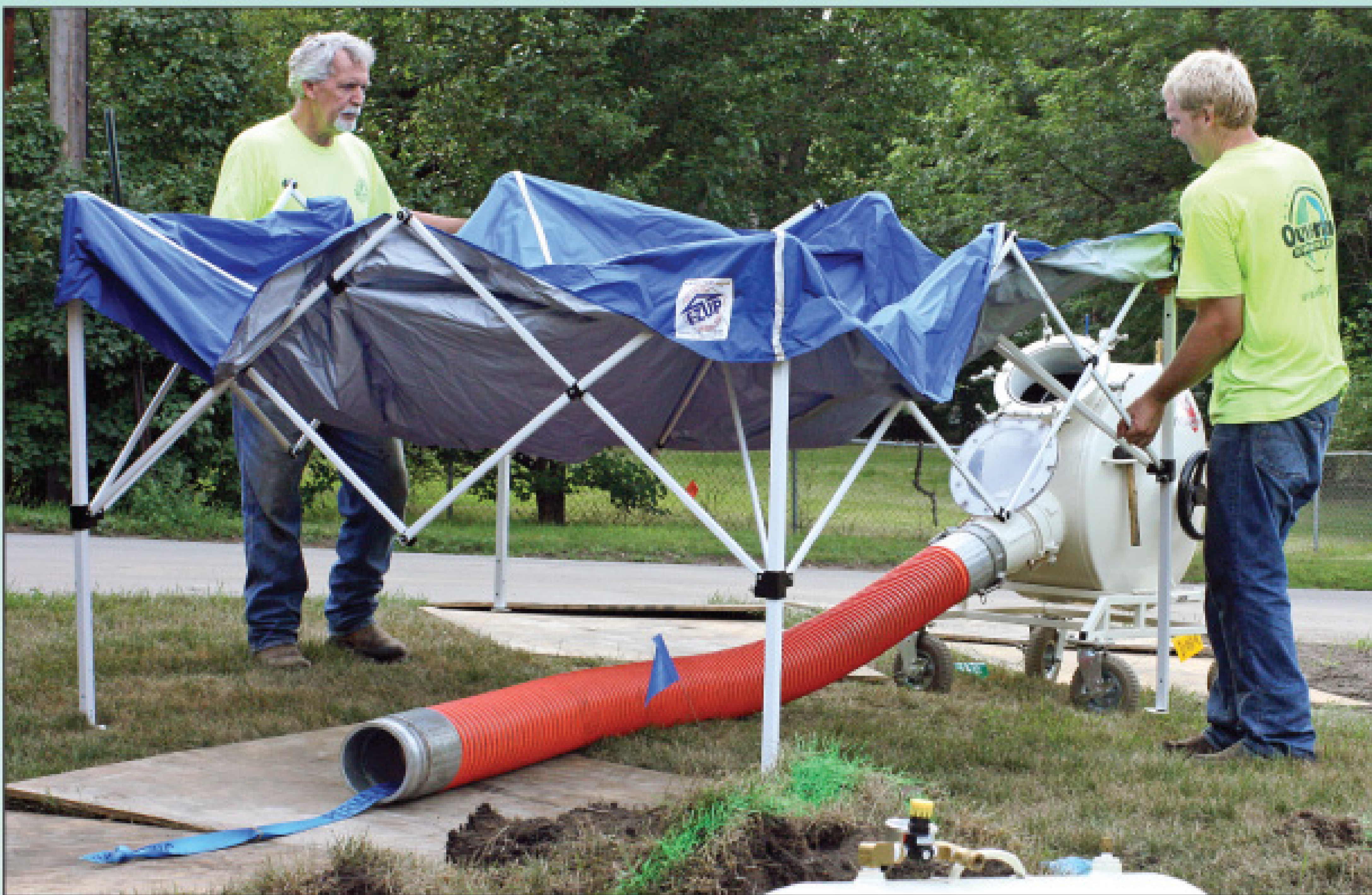
Doug and Troy Ouverson set up a canopy over the standard Perma-Lateral Inverter and delivery hose to protect the material and themselves from the elements.
