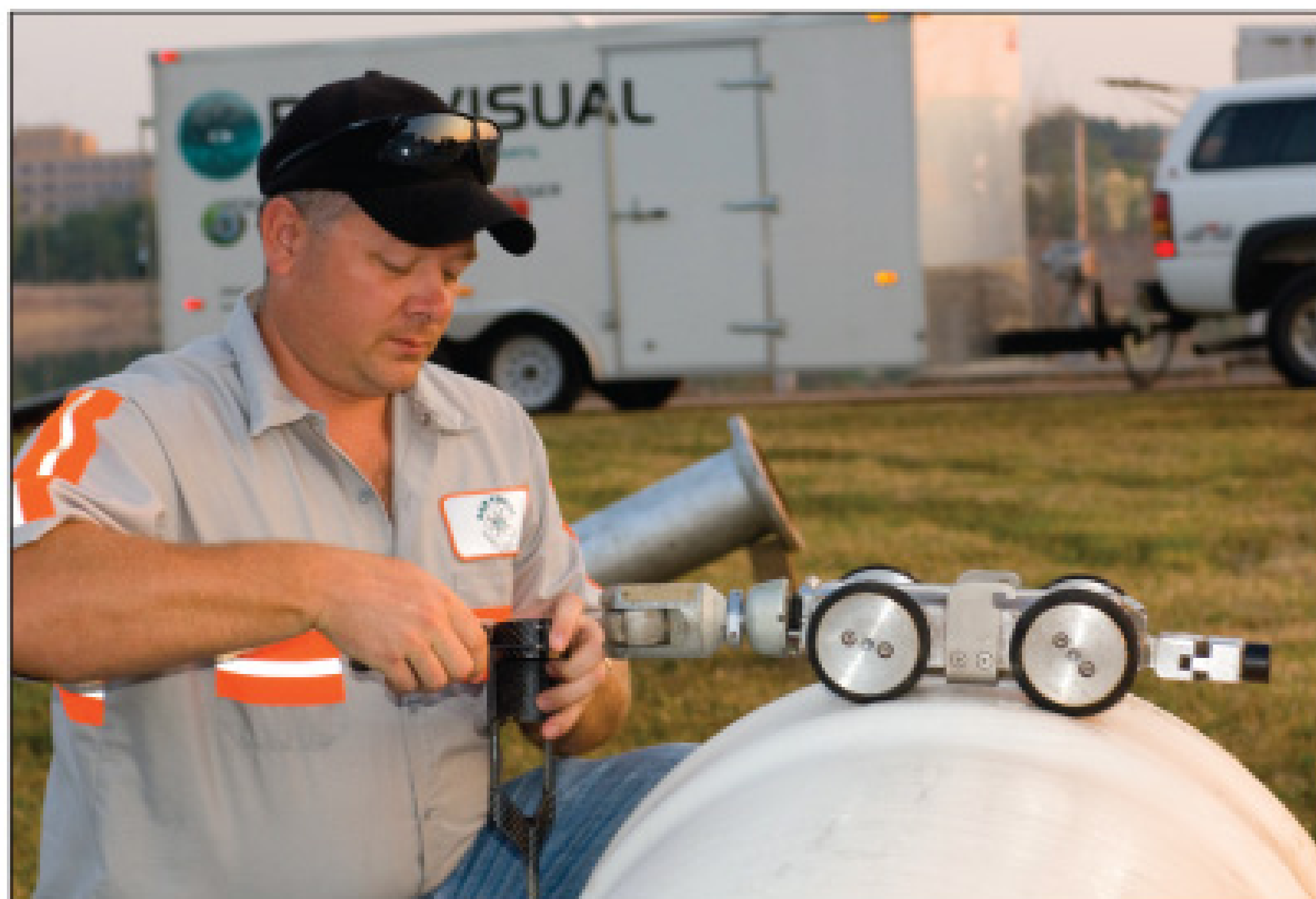
Jeremy Fansler installs a laser profiler on an Orion camera (RapidView) as part of an inspection project.
