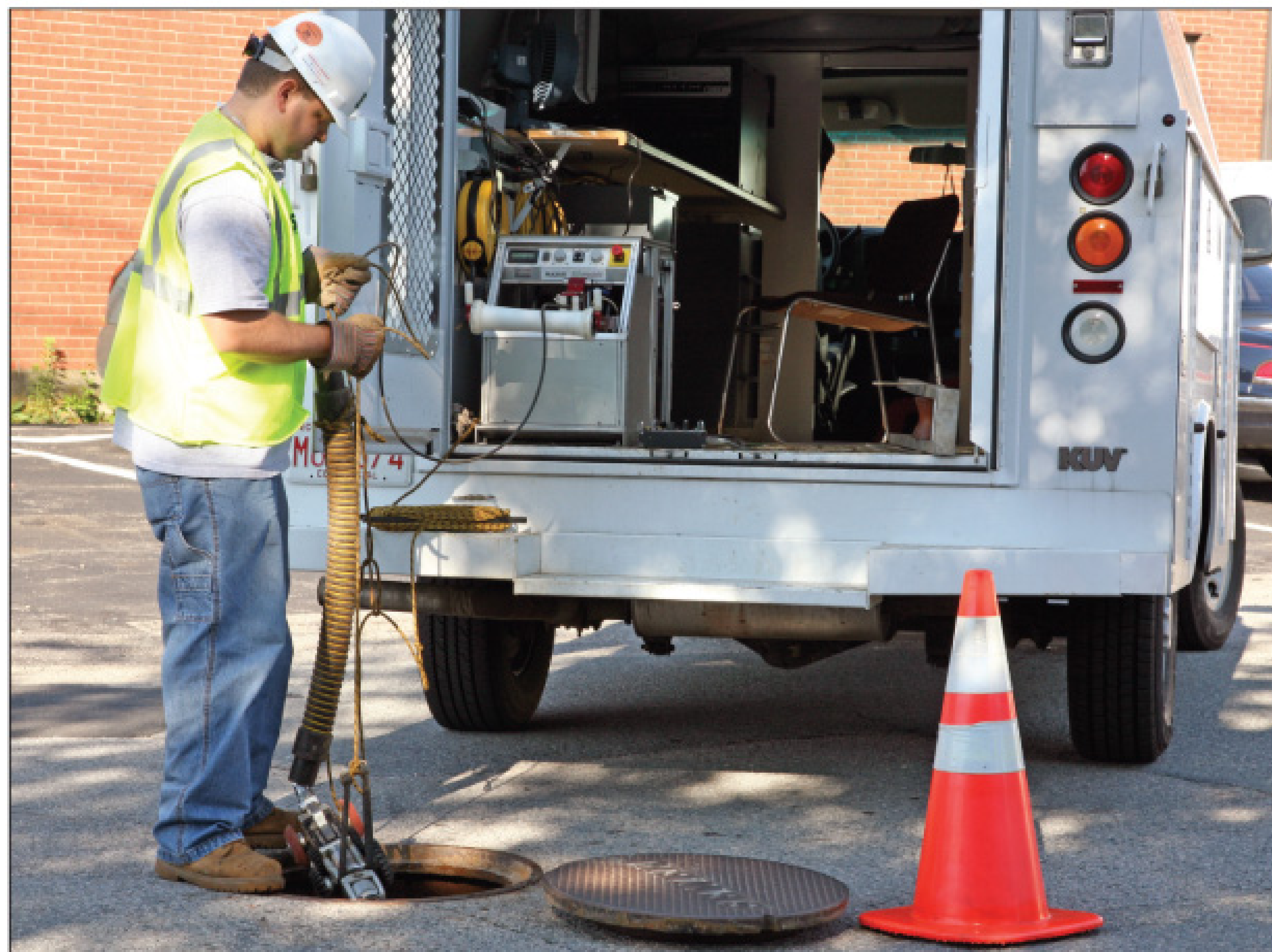
EST's Geoff Beyer deploys a crawler-mounted camera from the back of an inspection van.
