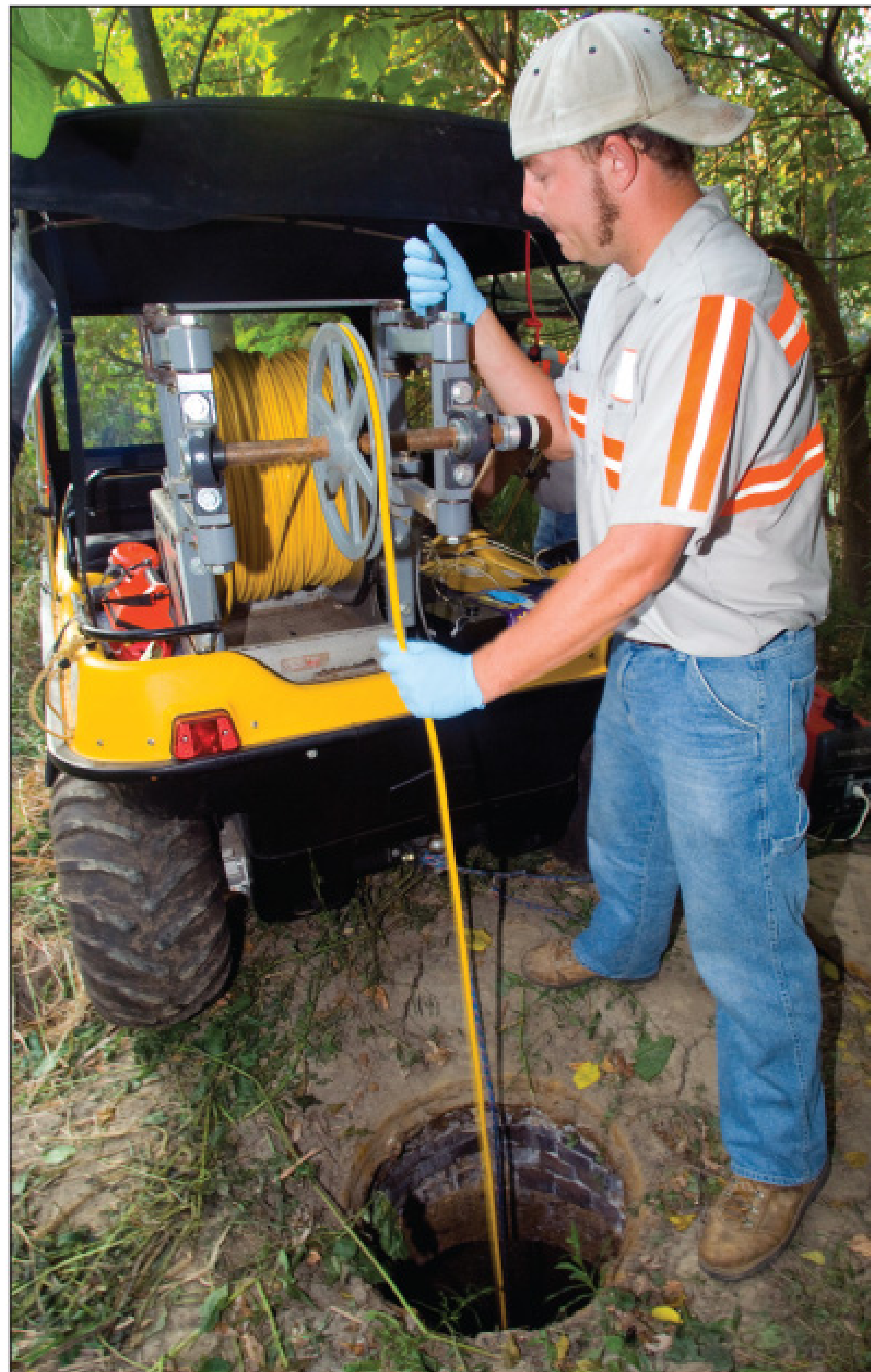
Bryan Benn of R&R Visual guides a sonar cable into a manhole for an inspection. Sonar profiling is among the advanced technologies the company uses to give customers complete data on their underground infrastructure.
