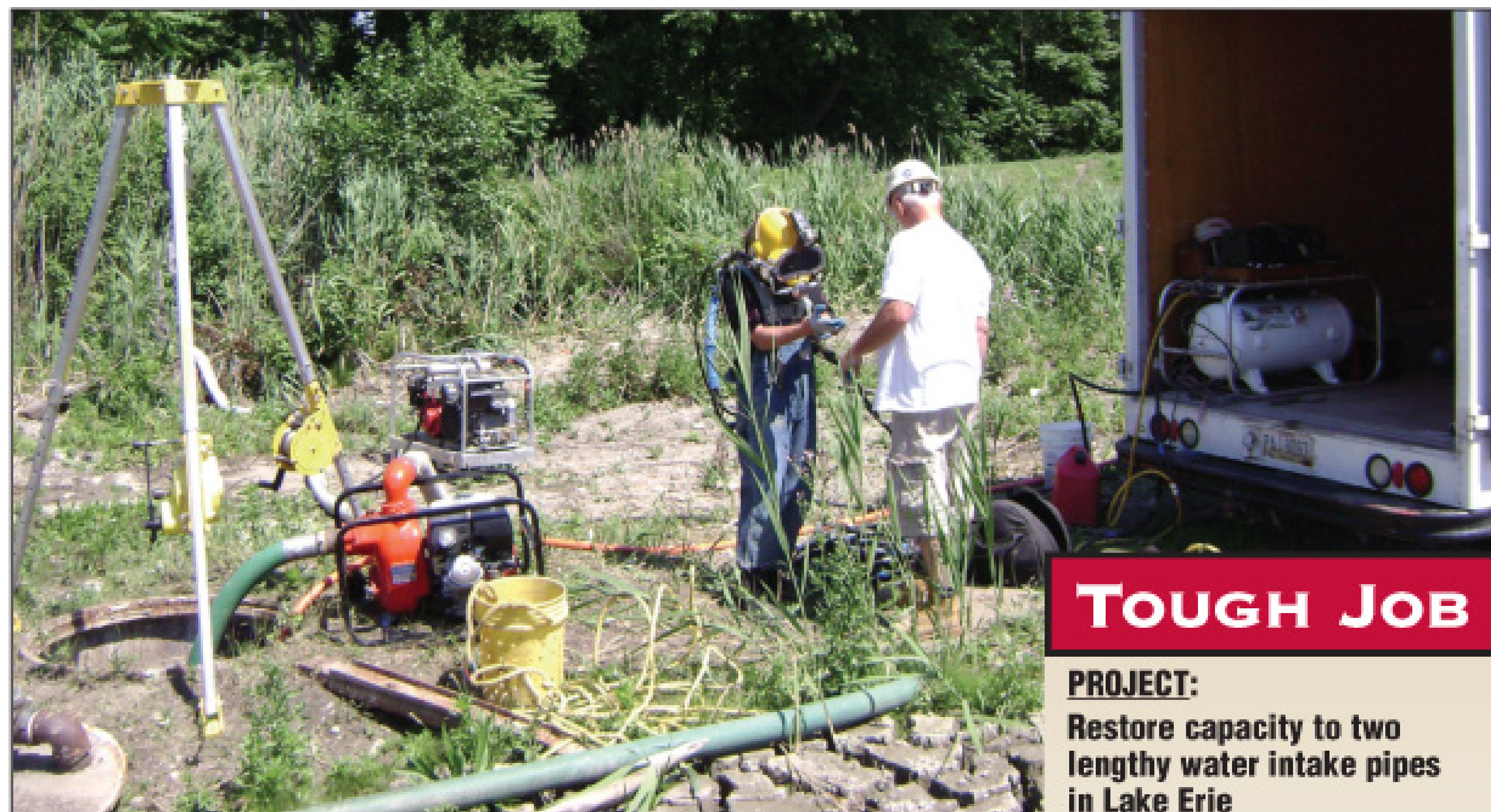
Lake Erie Diving's commercial diver Mike Murphy prepares to place cleaning equipment in a 3,000-foot-long, 30-inch intake pipe. (Photos courtesy of Pat Murphy, Lake Erie Diving Inc.)
