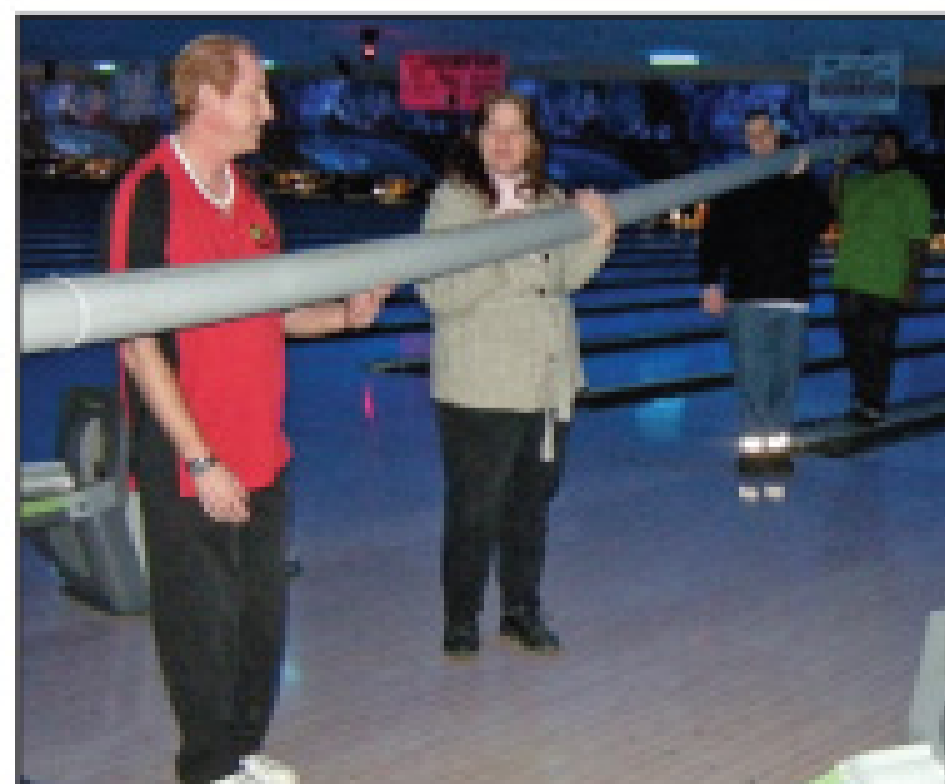
Diablo Lanes employees guide the fused pipe across the floor while the other half of the bowling alley remains in use.
