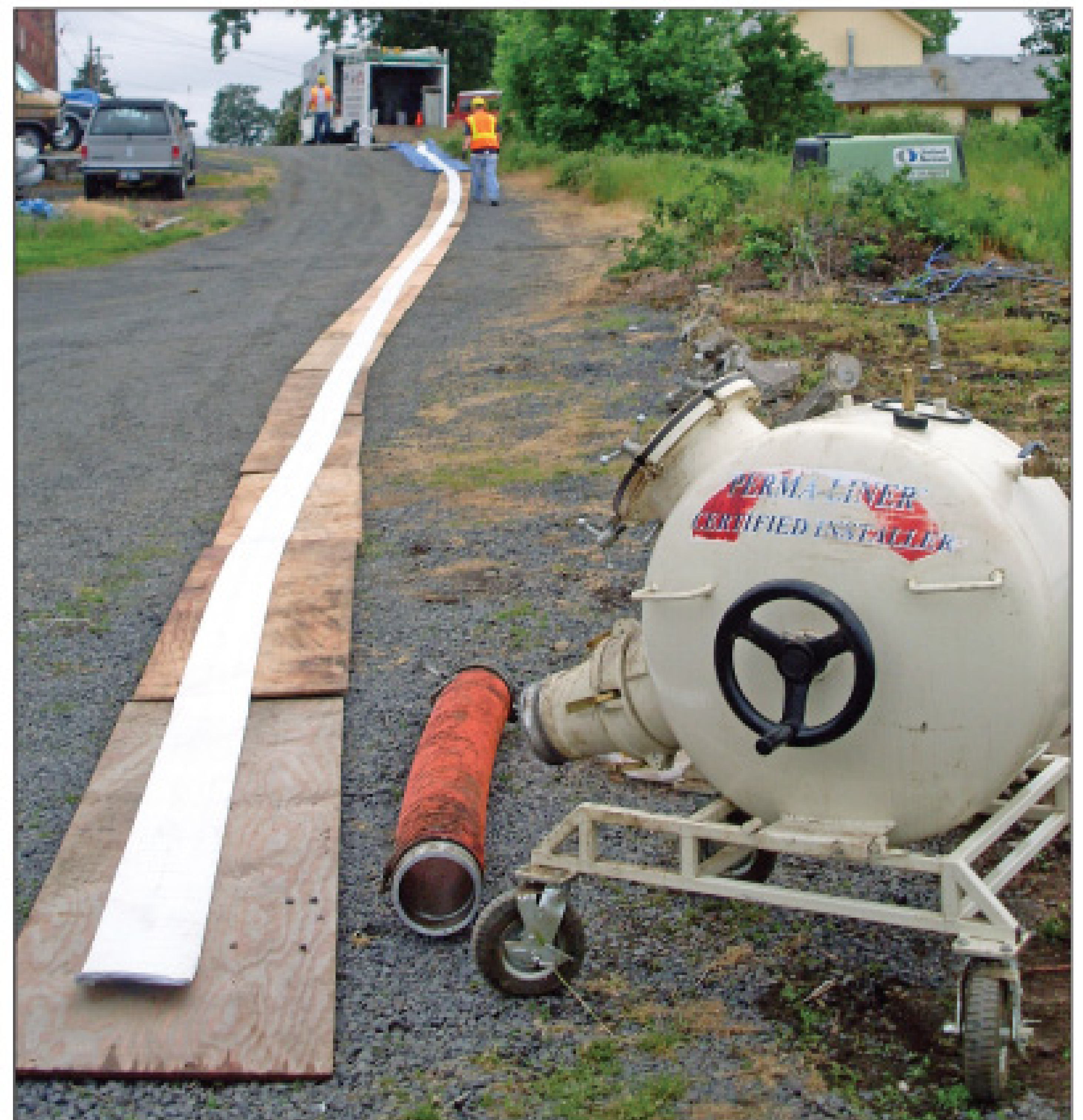
An inversion canister is shown at the end of the liner, ready to be installed.
