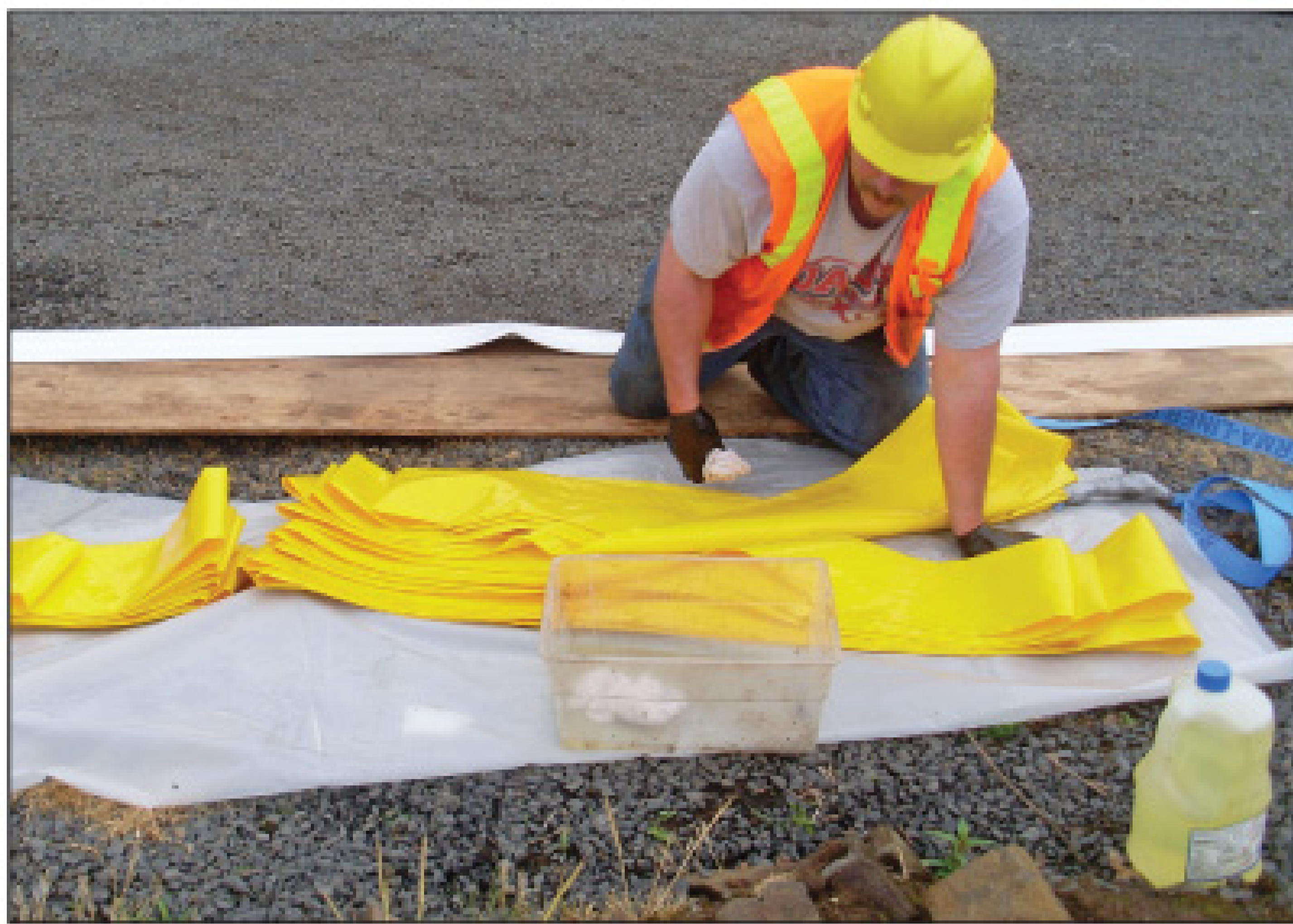
Lining installer Steve Neal slicks the calibration tube with environmentally friendly vegetable oil to help it slide in and out of the liner when it is inverted.
