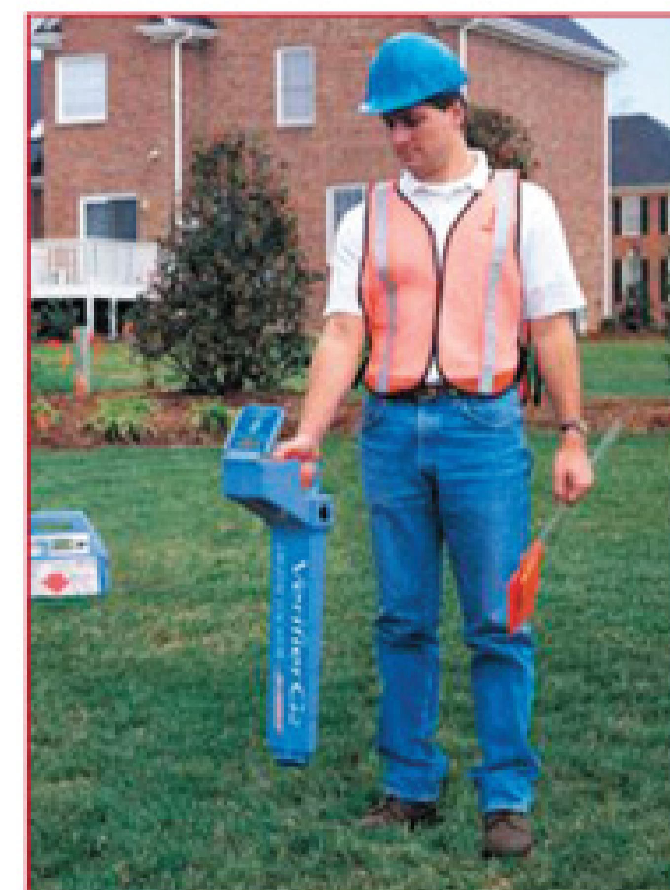
A worker uses a locator to find telecommunication lines in a residential area.
