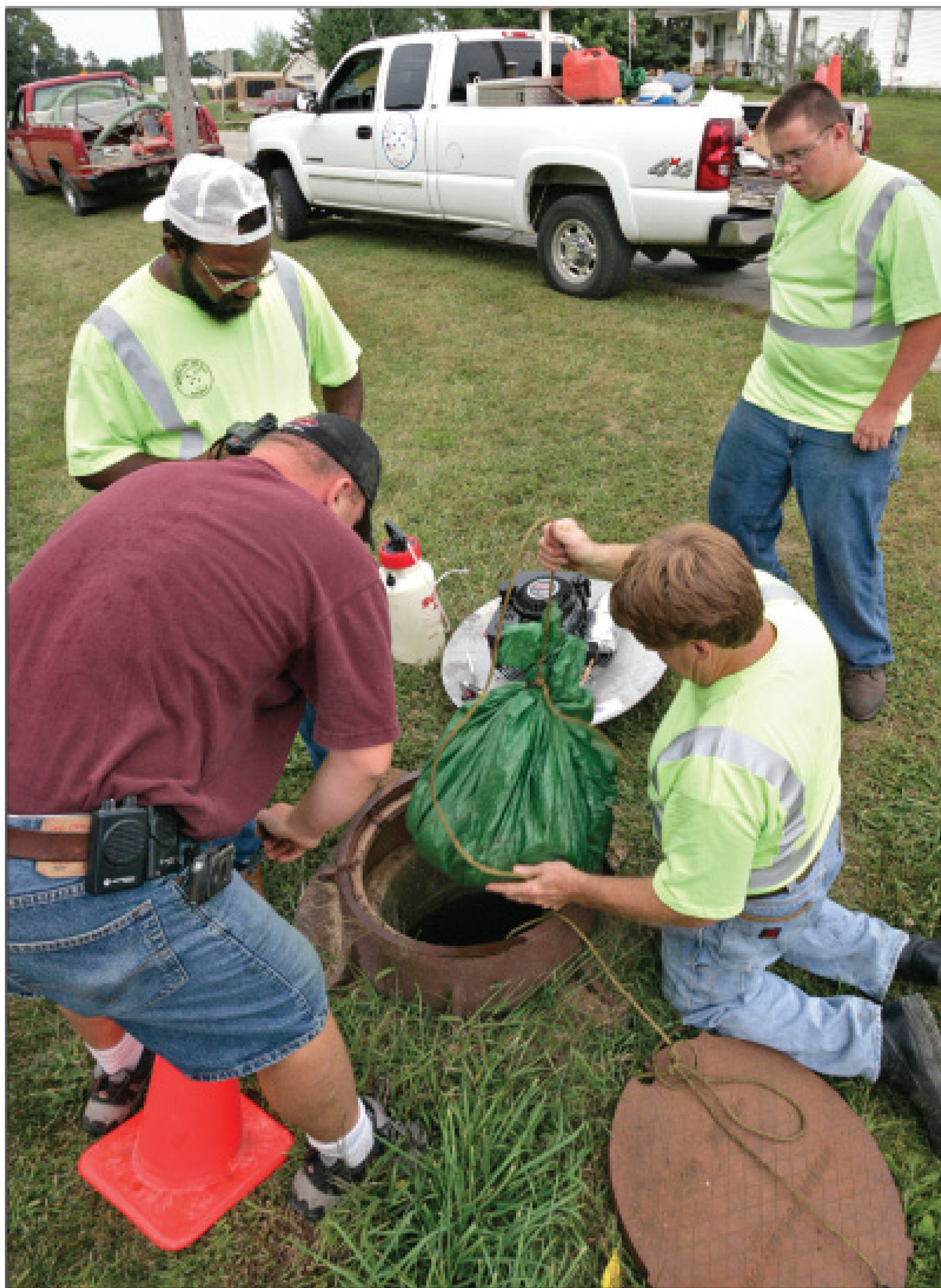
Harlan Sargeant drops a plug into a sanitary sewer manhole before smoke-testing sanitary sewer lines.
