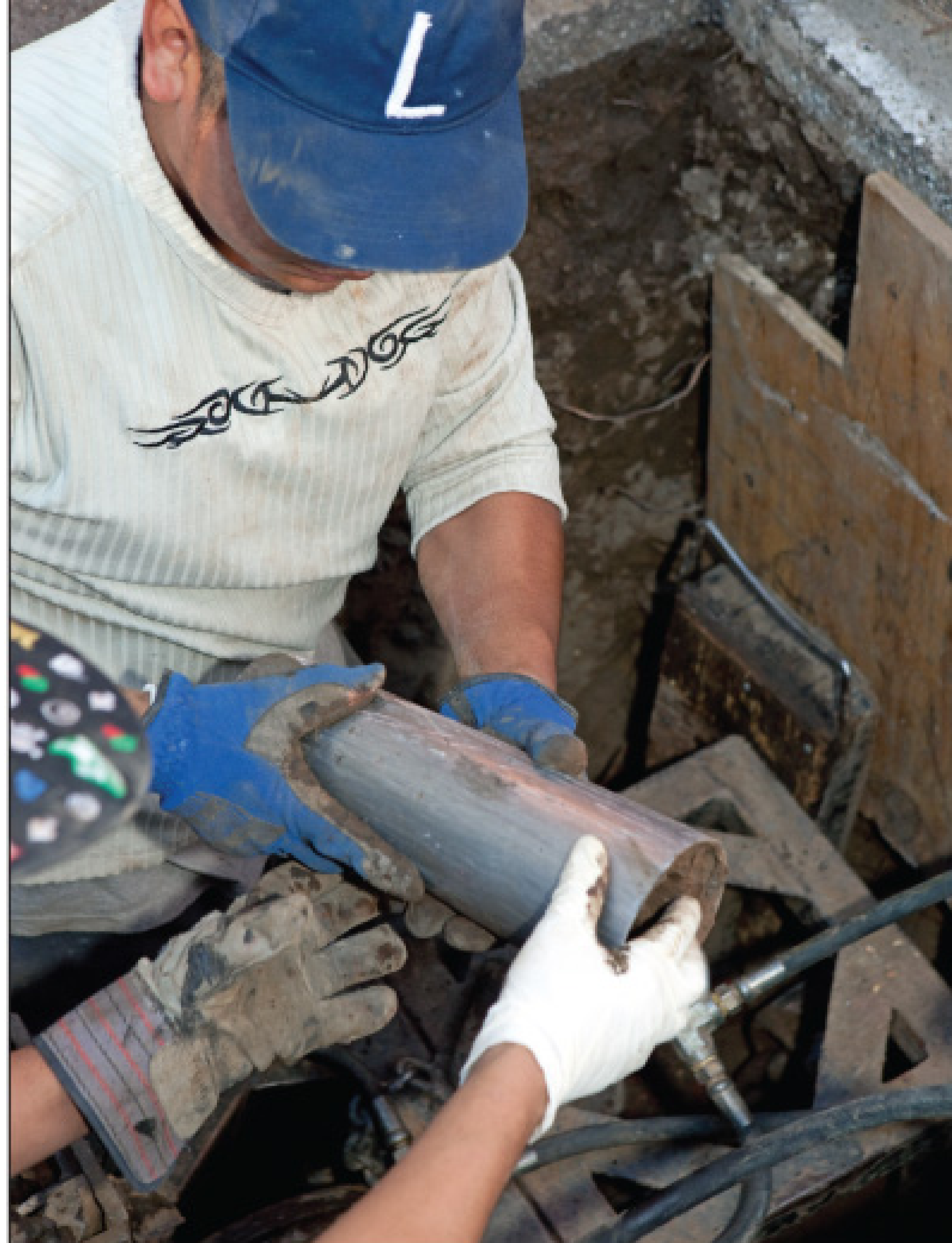
Breaking cones on the bursting unit are used to shatter the existing clay pipe.
