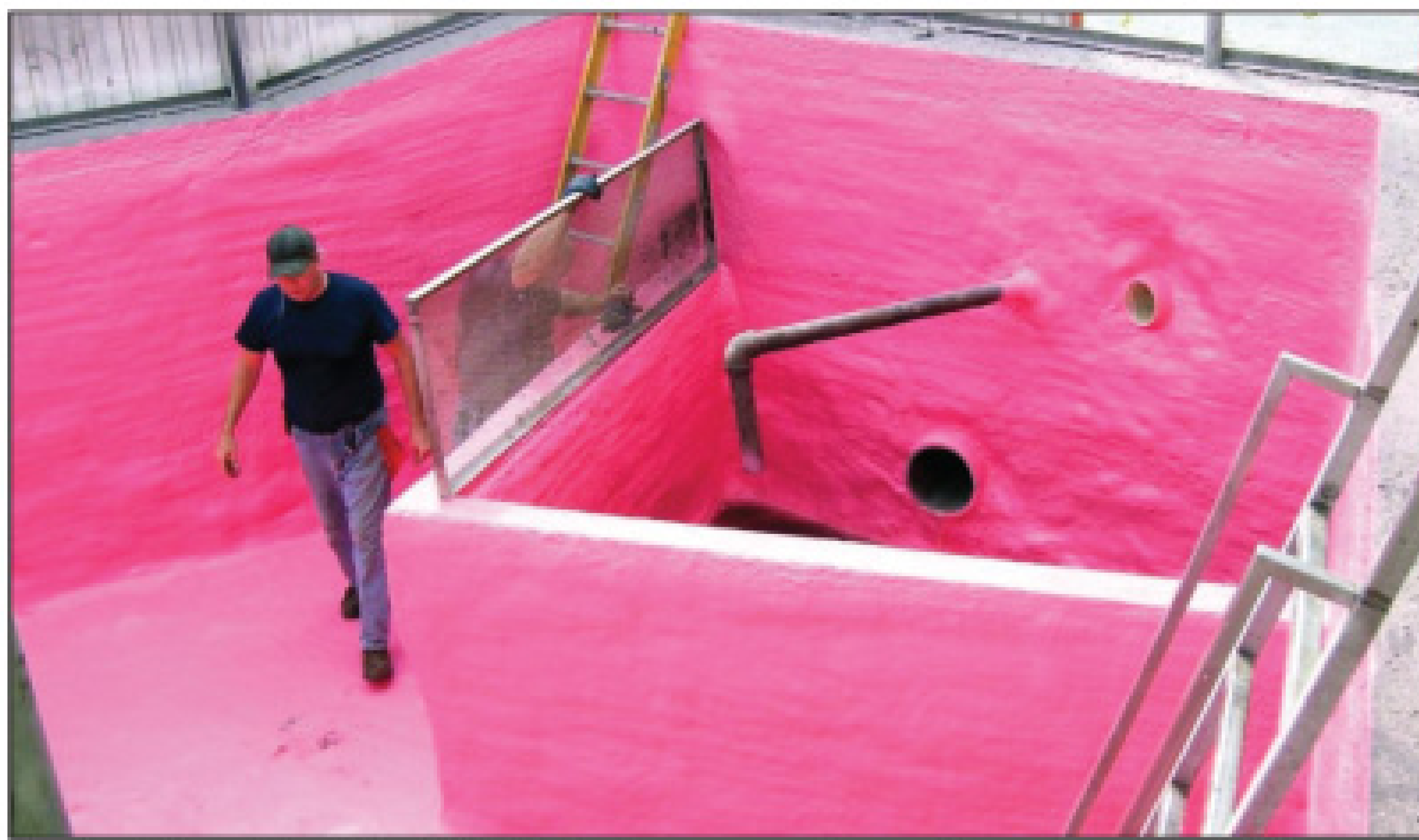
The first layer of the SpectraShield system was a primer designed specifically for saturated concrete.
