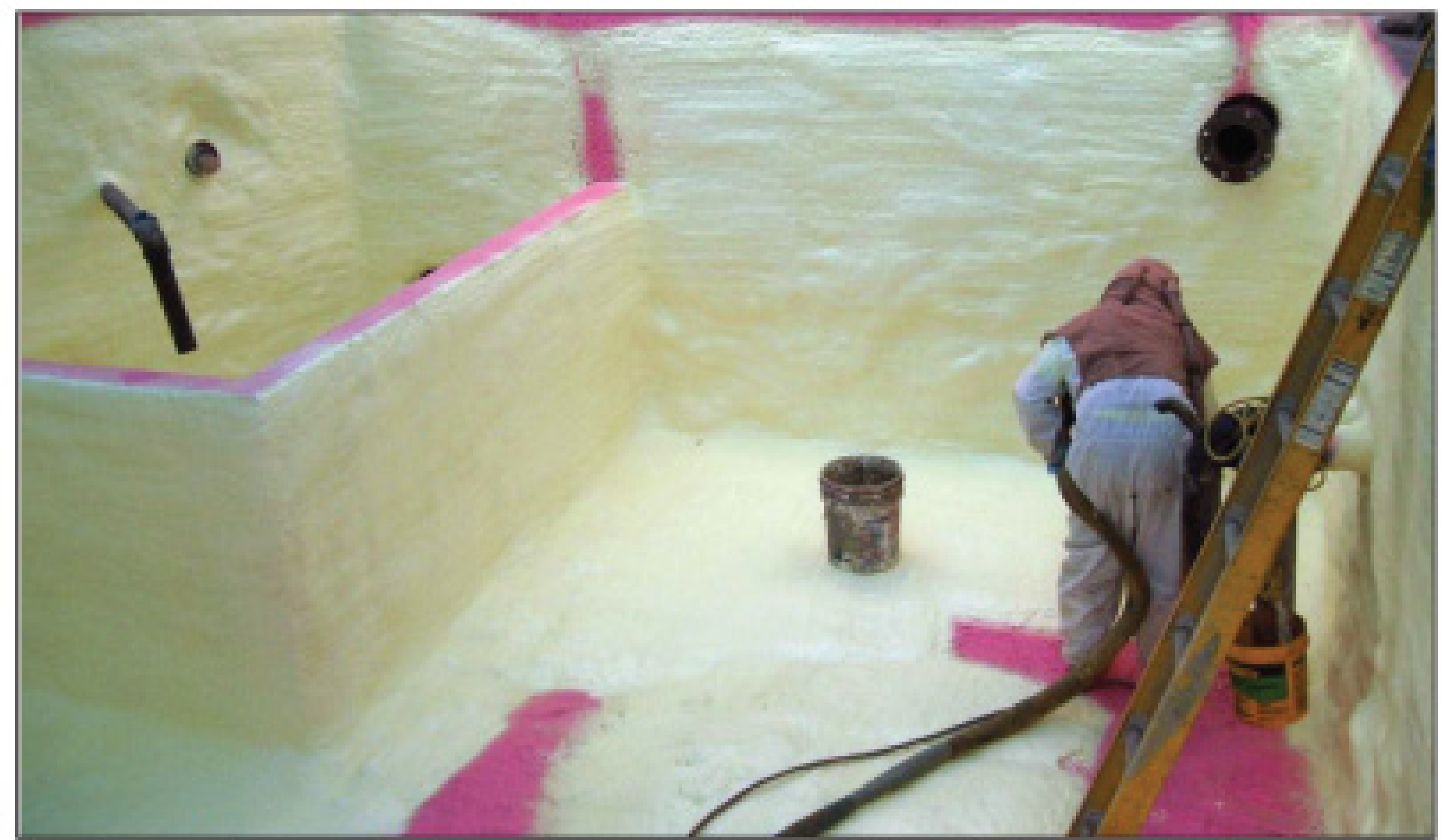
Two layers of sprayed-on foam sealers finished the tank restoration job. Matias Garcia Jr. applies a layer of polyurethane foam over the pink primer in the outside tank.
