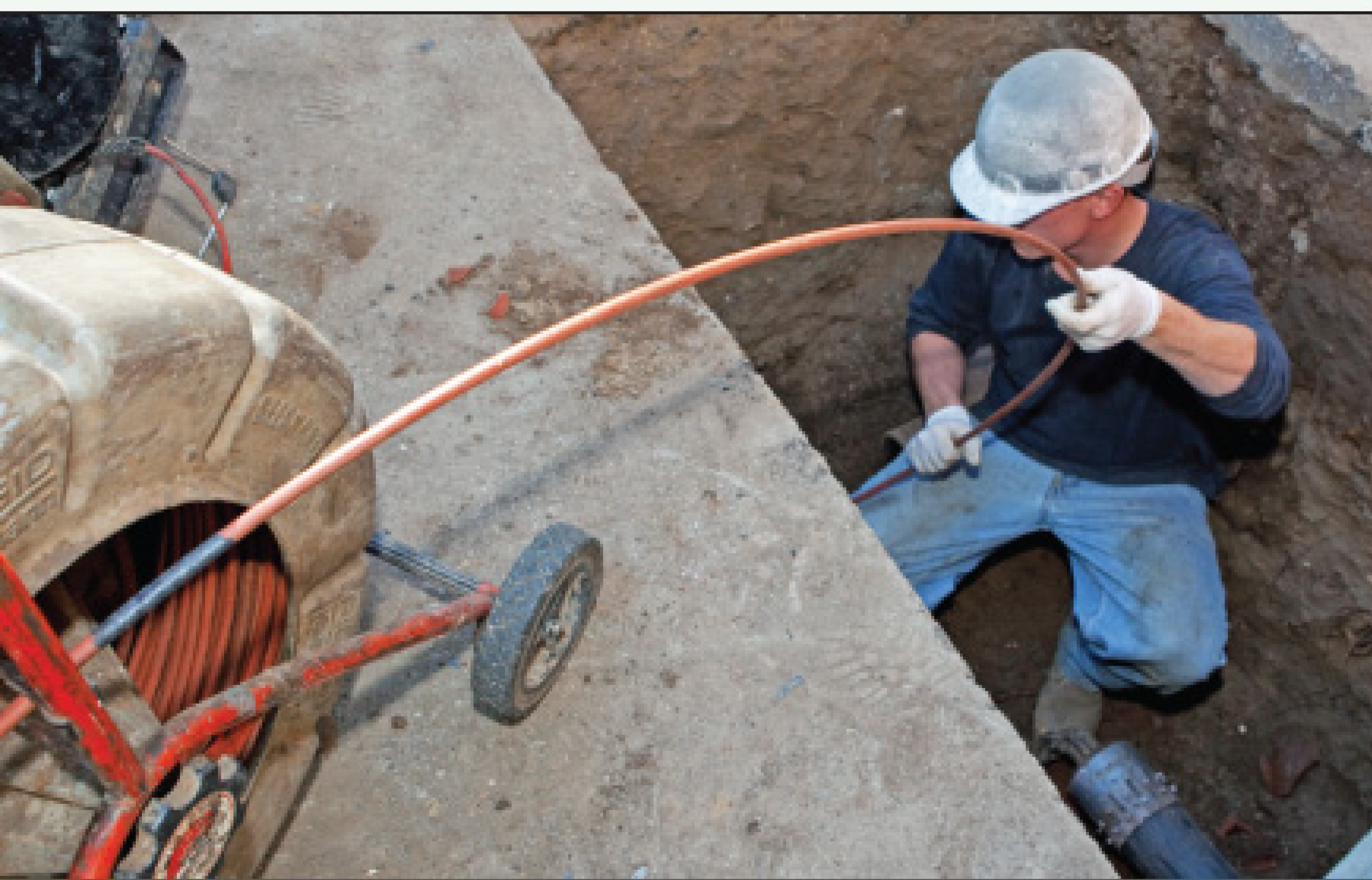
Top photo, Mark Tomlinson and Alex Marchuk of Sewer Line Video Inspection make sure the pipe, pulled from the other side by a Pipe Genie bursting unit, goes in without incident. Lower photo, Marchuk runs a SeeSnake inspection camera from RIDGID into a pipe. (Photography by Patrick Botz-Forbes)
