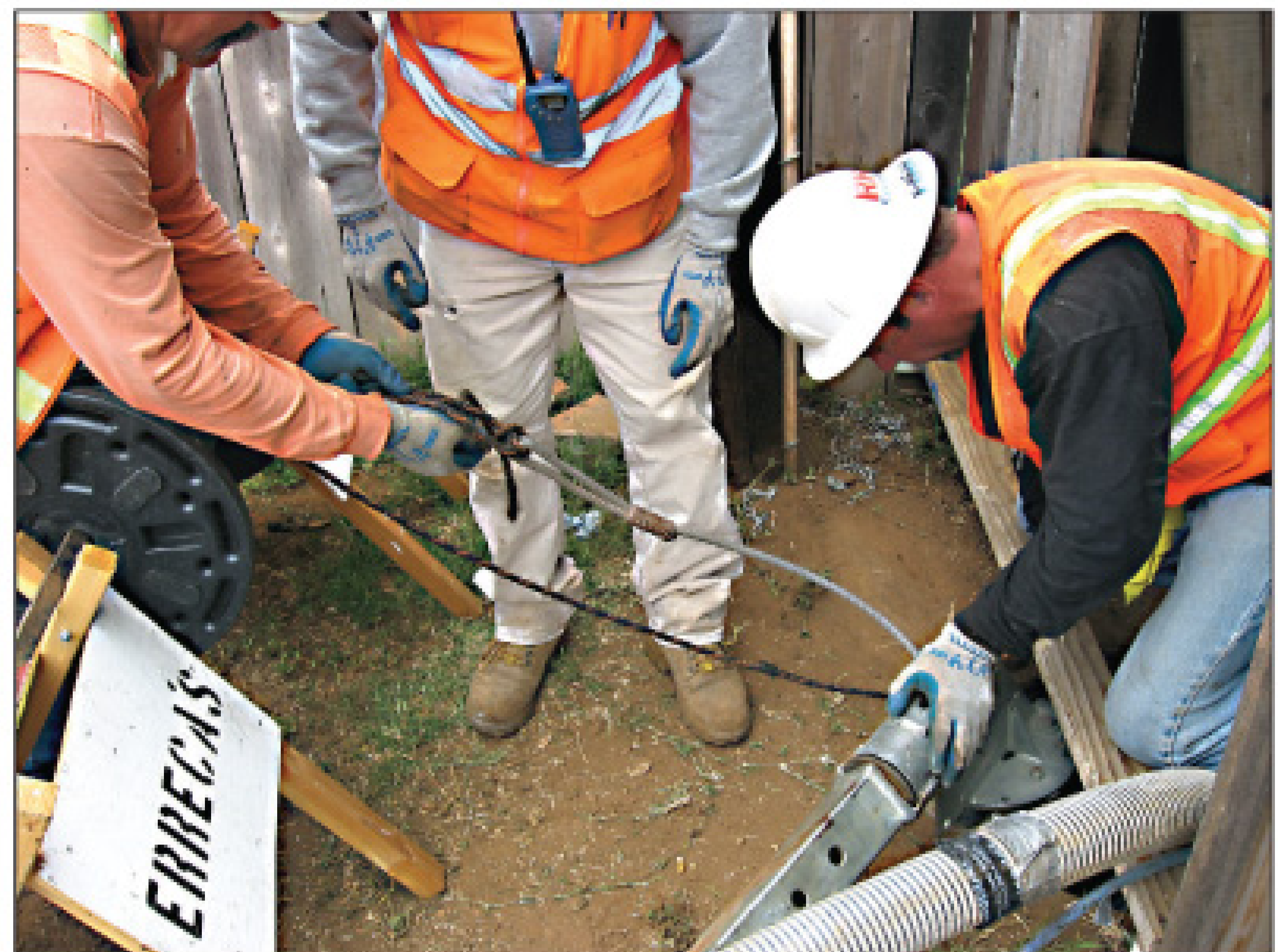
Workers from Erreca's Inc. in Lakeside, Calif., lower the ultraviolet light chain. The sewer rehabilitation system was light enough for them to carry into residential back yards and urban canyons.
