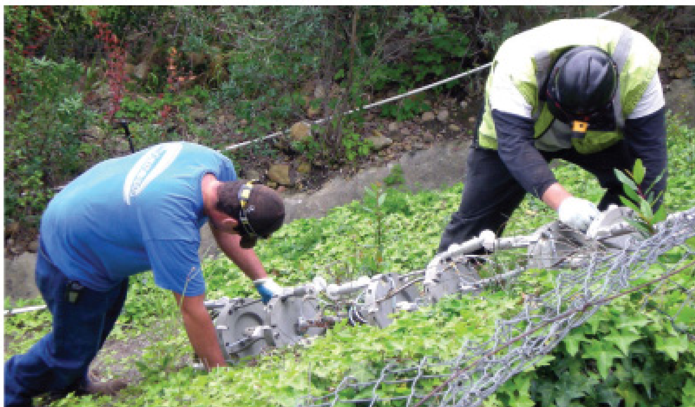
Superintendent Chris Holden (left) and foreman Roy Gallegos maneuver the light chain over a chain-link fence and down a 45-degree slope to a downstream manhole in a canyon. The 275-foot-long, 36-inch pipe to be lined sloped 40 degrees between the upstream and downstream manholes.
