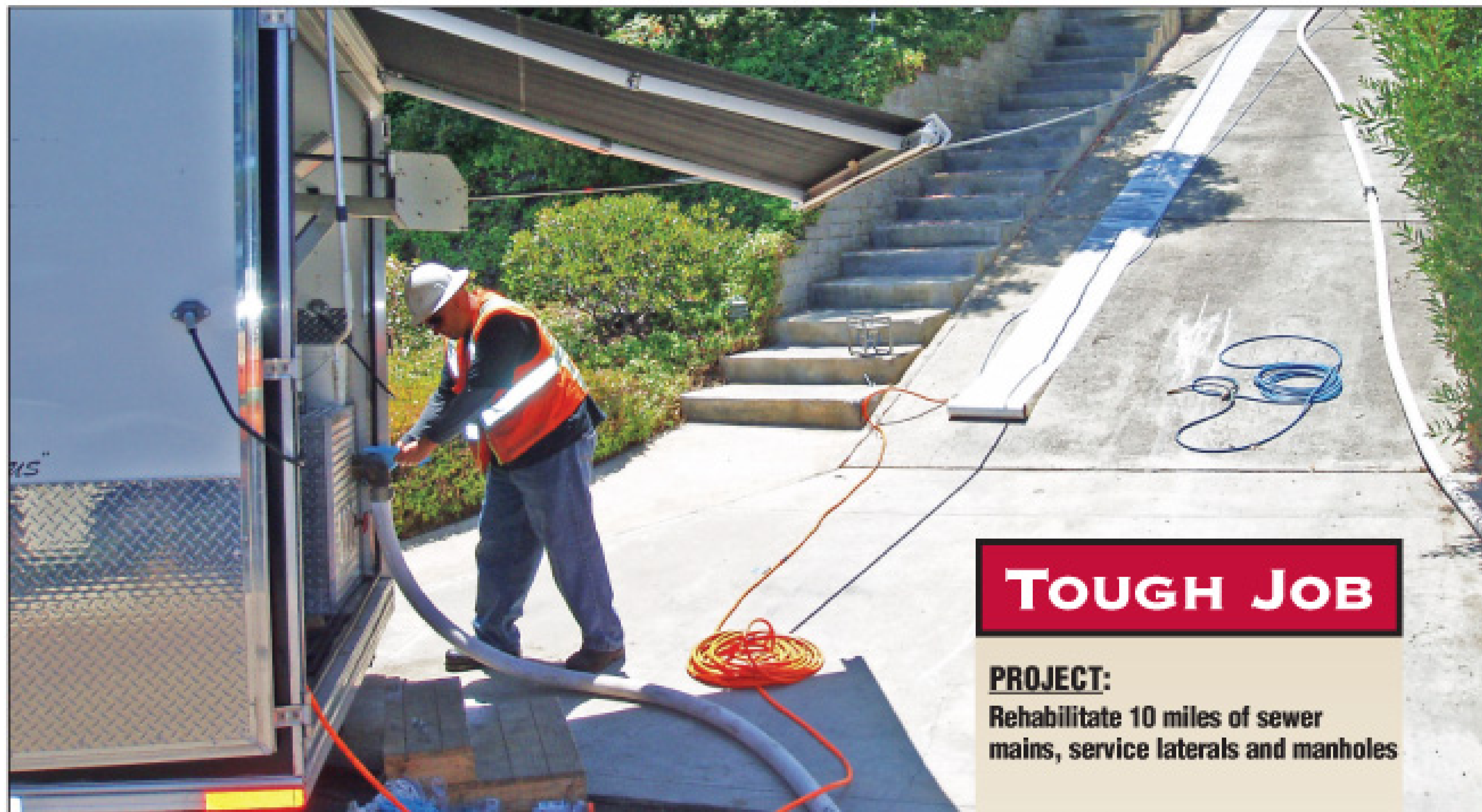
William Barreda prepares to run cables and hoses 120 feet from the street to a backyard manhole. The plastic foil that protects the liner extends up the middle of the driveway. (Photos courtesy of International Pipe Lining Technologies)
