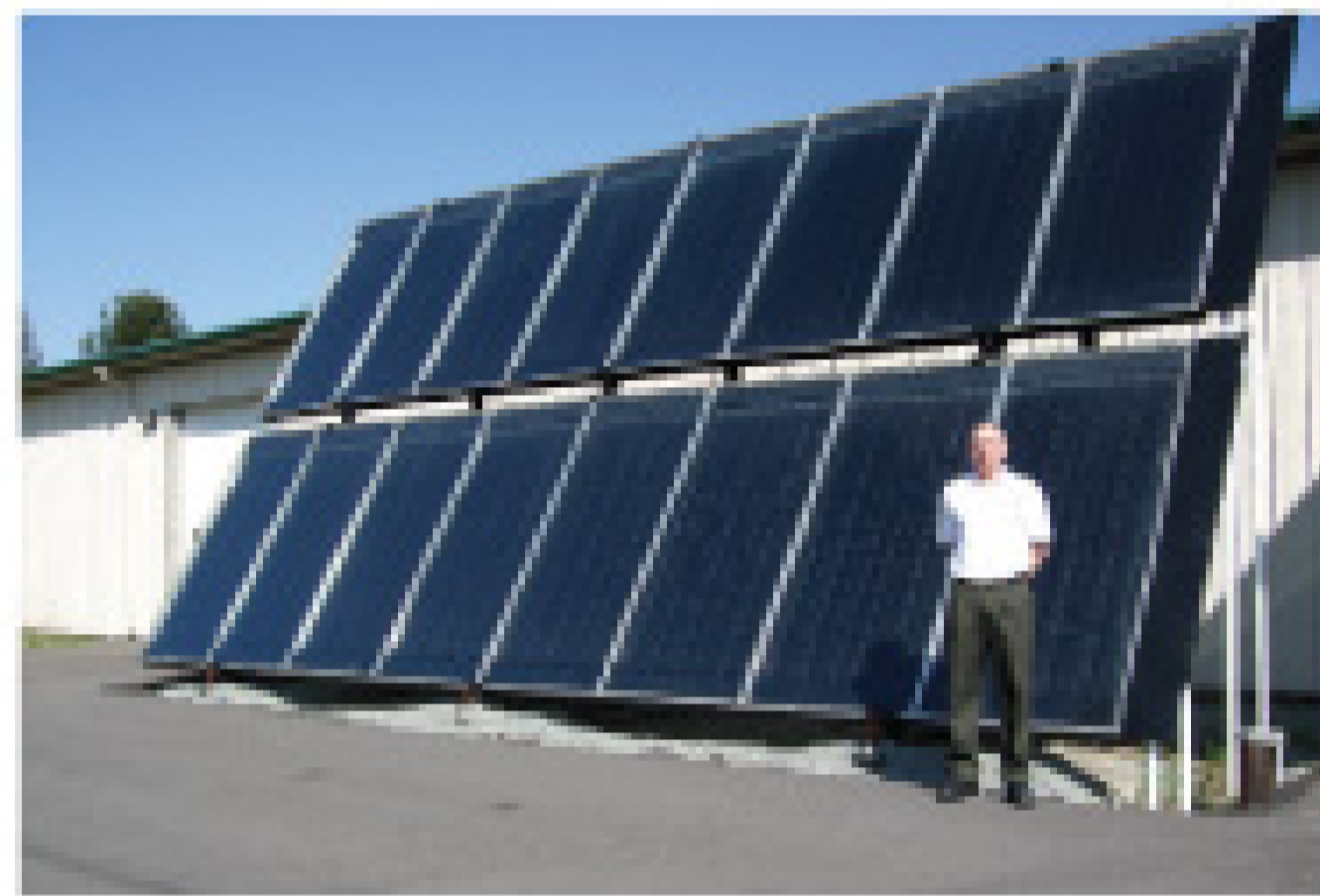
Jerard Nighorn, vice president of sales, stands next to the solar heat panels installed at the Lenzyme facility.
