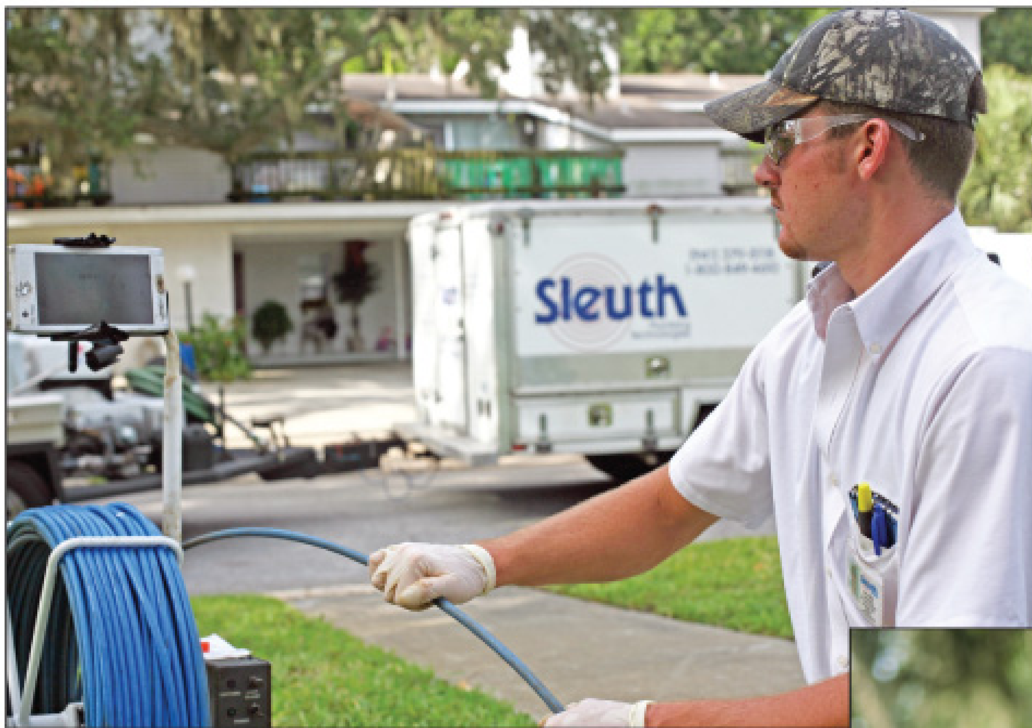
Josh Miller checks the video display as he drops a camera into a 6-inch cleanout at a housing complex.
