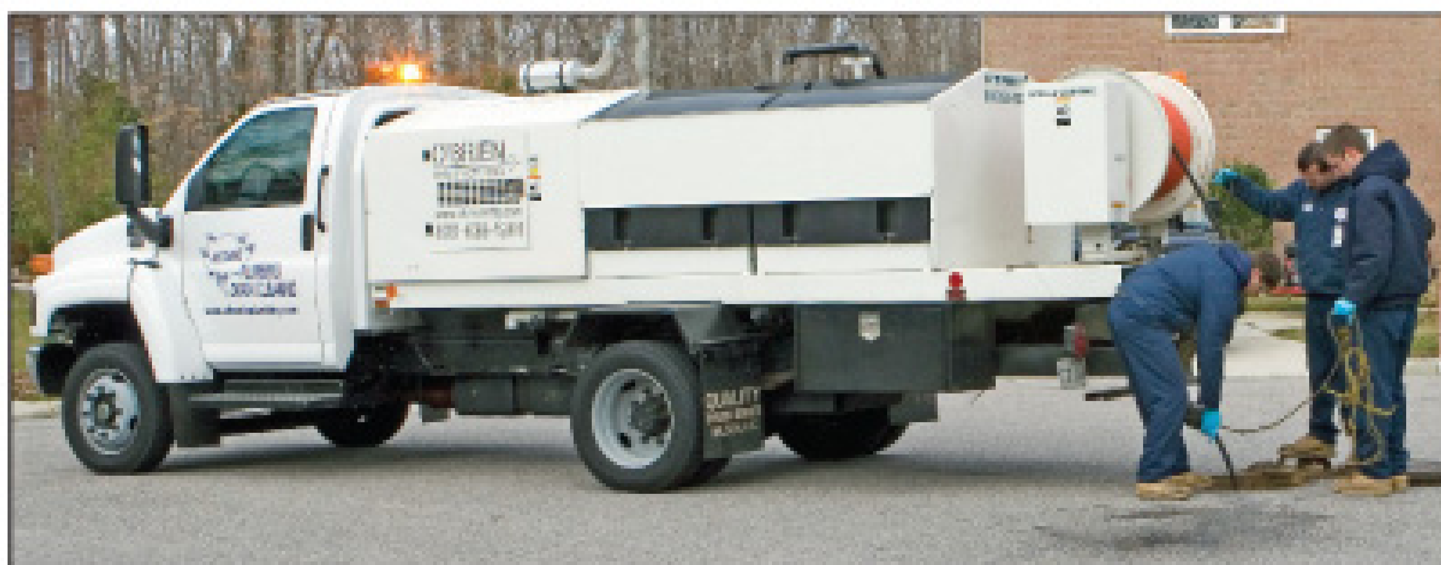
Keane, McCants and Landry jet a mainline sewer using a truck-mounted jetter.
