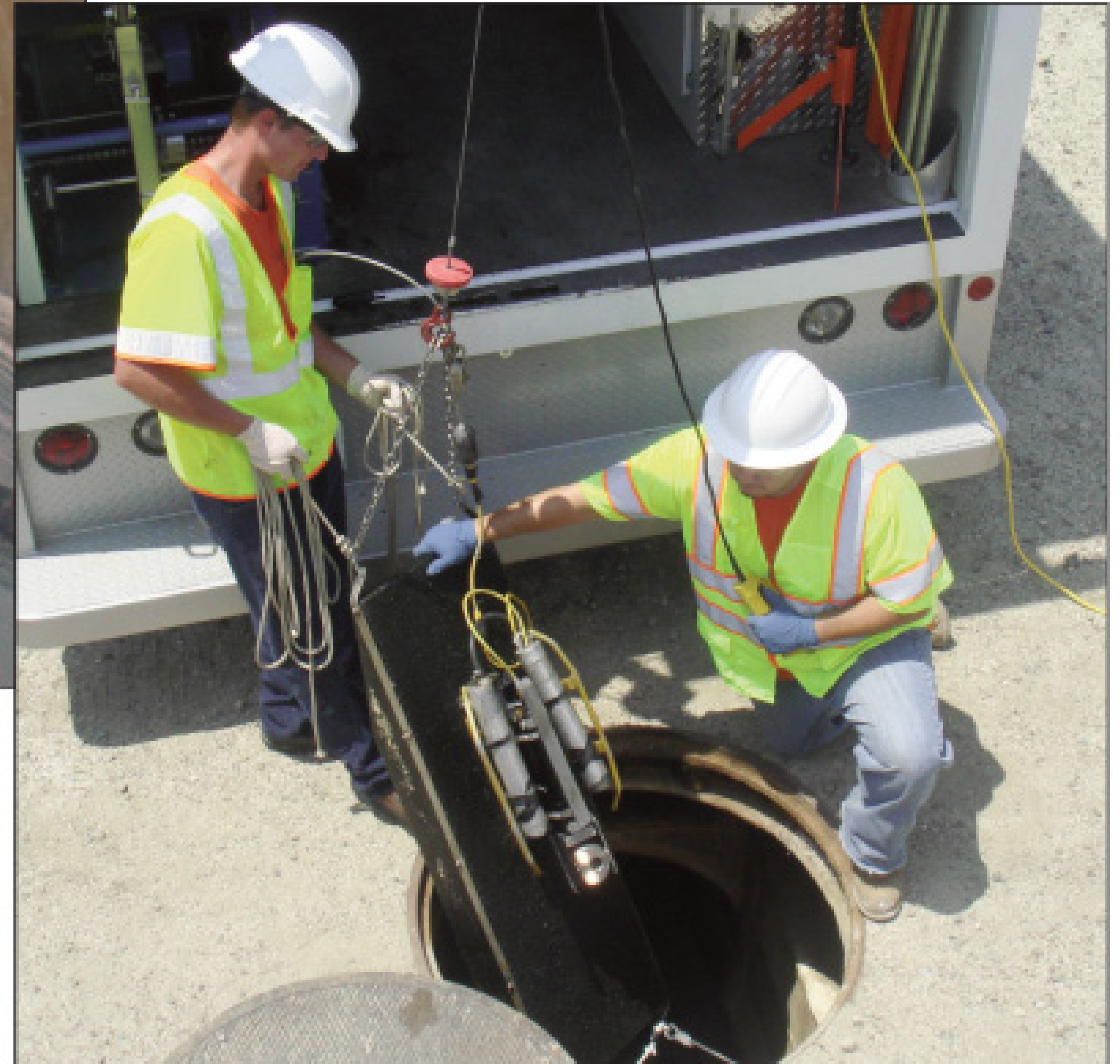
Below: A camera float rig is shown ready for deployment. Floats can be tethered from the upstream manhole only or from both ends.
