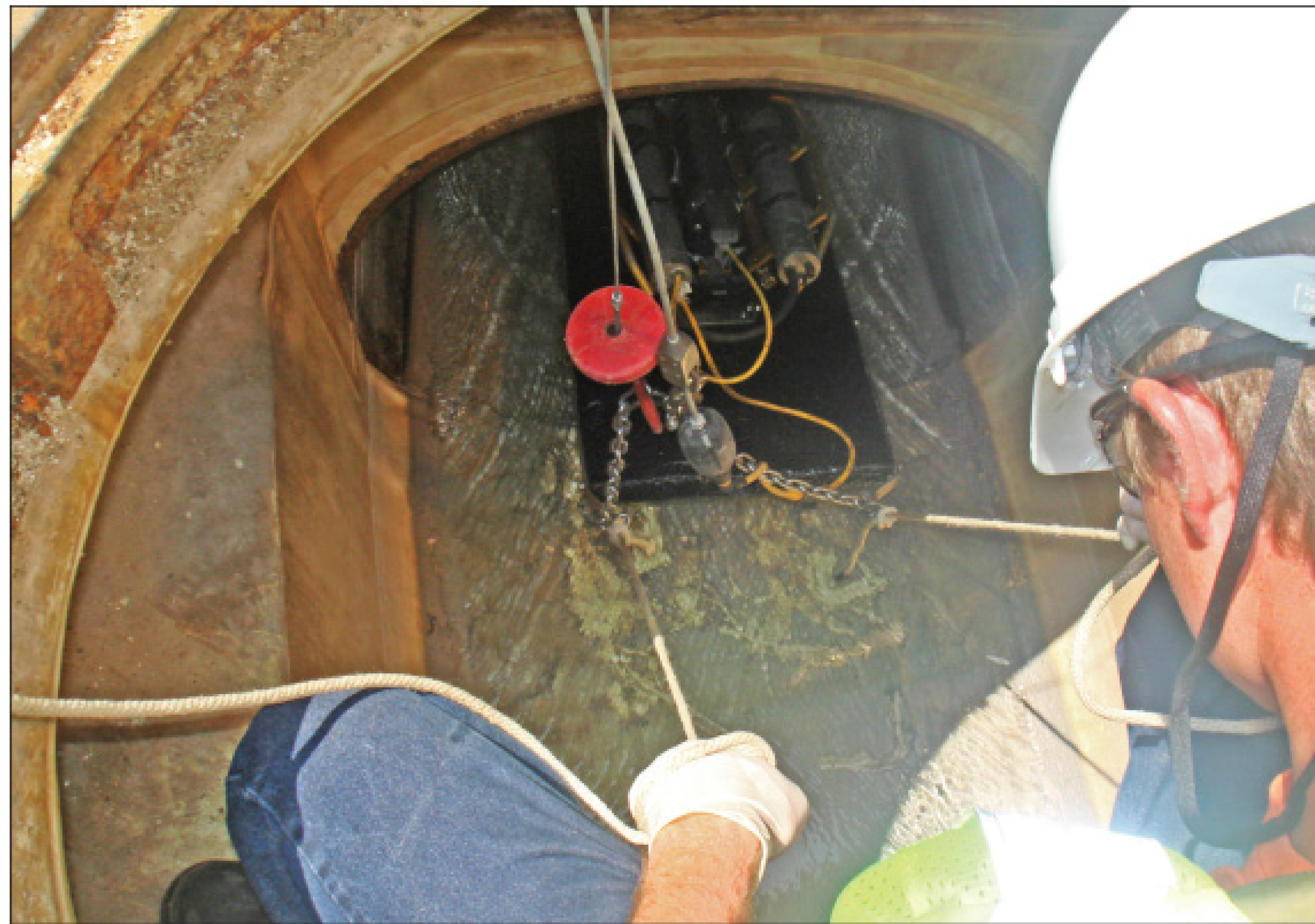
An inspection technician lowers a camera on a float rig into a mainline sewer. (Photography by Jim Aanderud)
