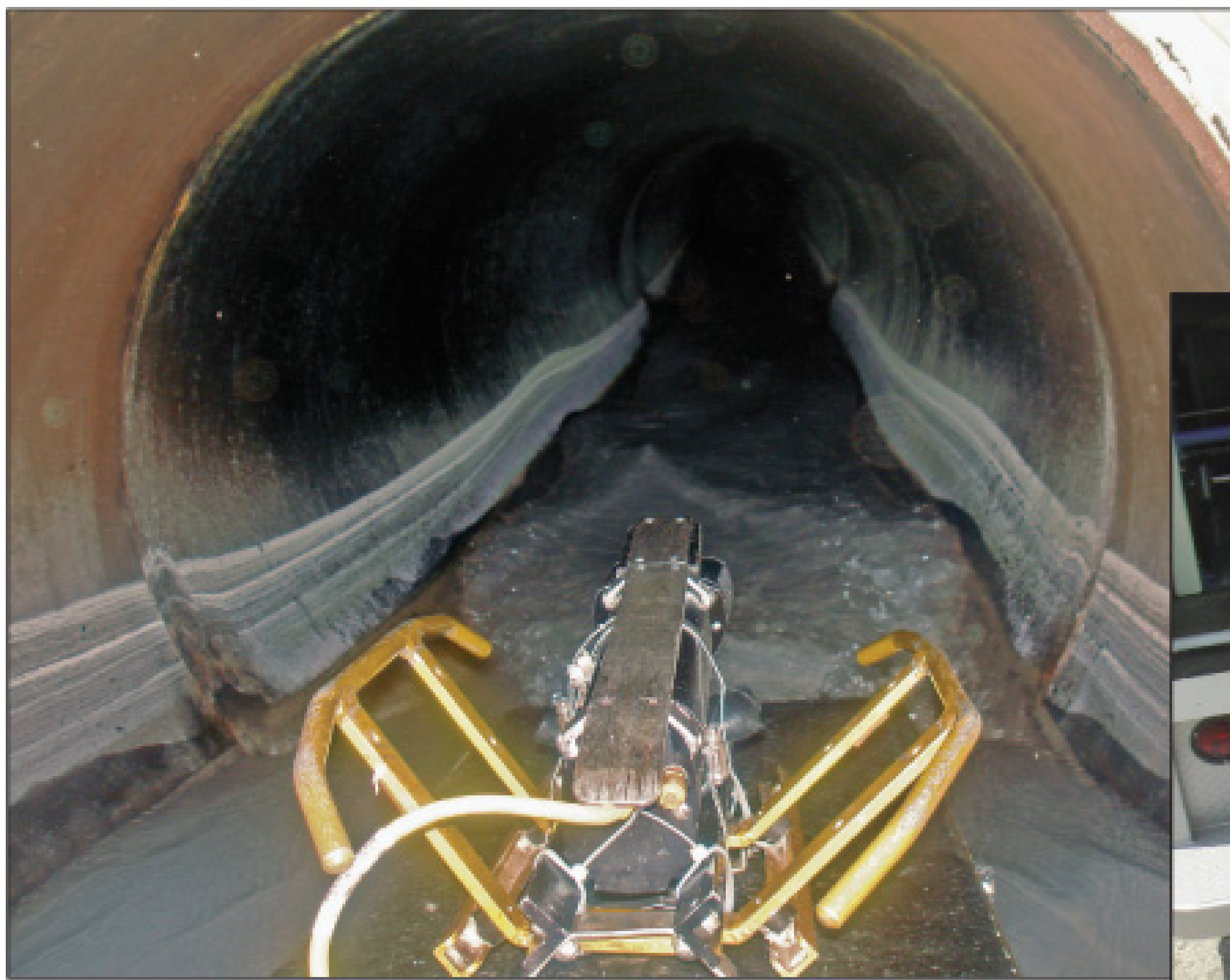
Left: A camera on a float proceeds down a mainline under heavy flow. Floats enable high-quality inspections under conditions where a traditional camera crawler cannot be used.
