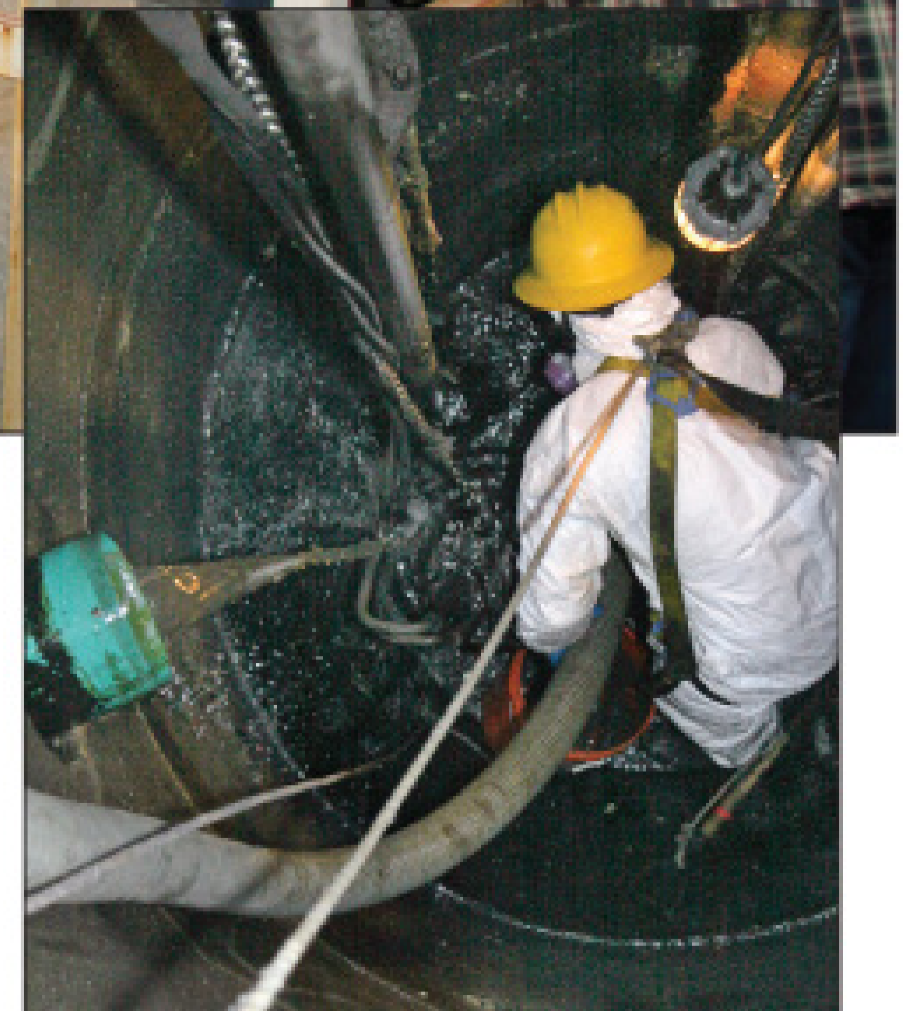
Hunter Smigelski of Sturgeon Creek Enterprises LLC, a subcontractor of L.W. Morgridge, is lowered by a crane and supported by a lifeline during a confined-space entry, picking up rocks and debris from a hospital's sewage ejector station.
