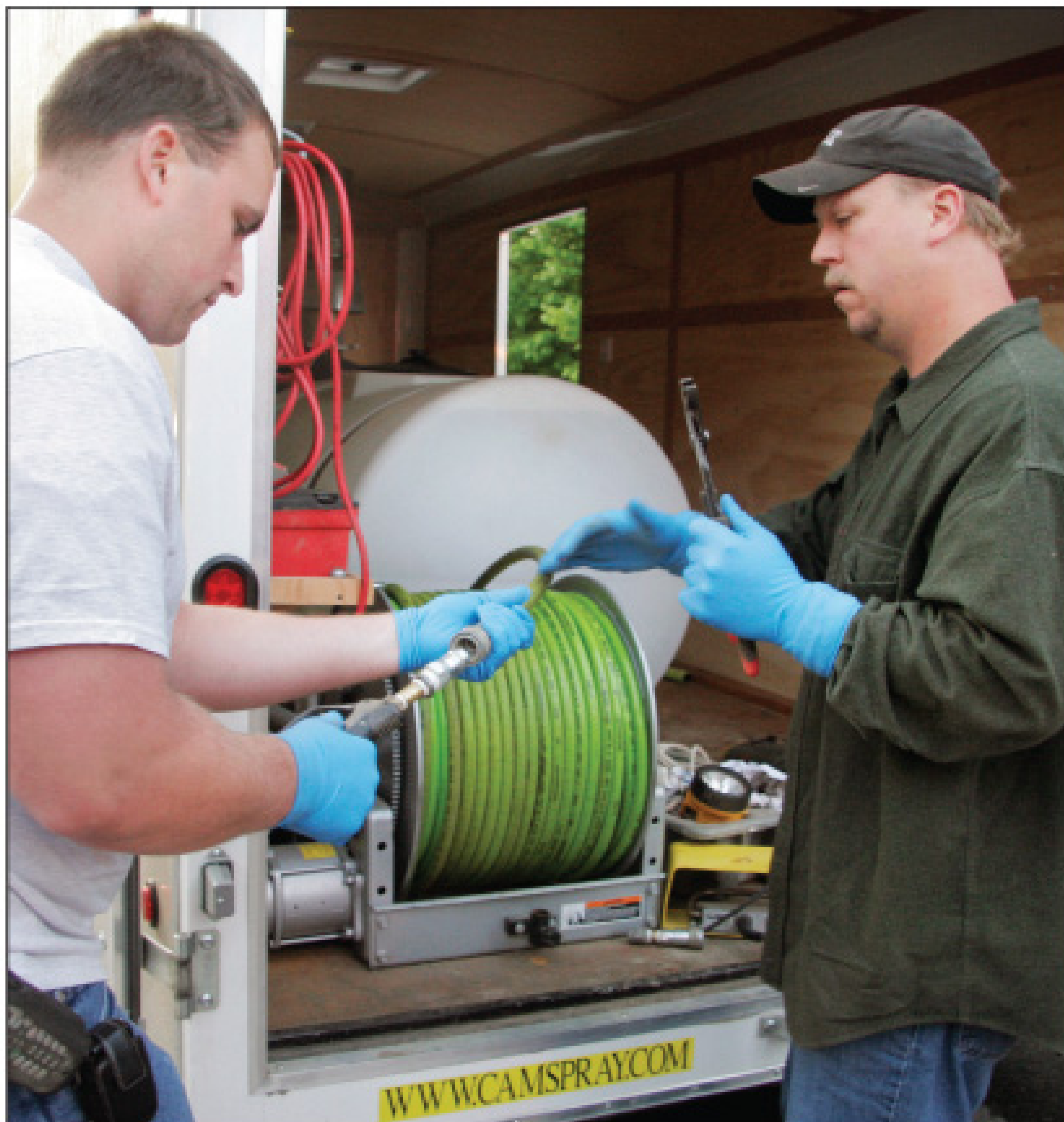
Matt Lizotte, left, and John Adams of L.W. Morgridge attach the jetting wand to the hose on a Cam Spray jetter in preparation for a cleaning job.
