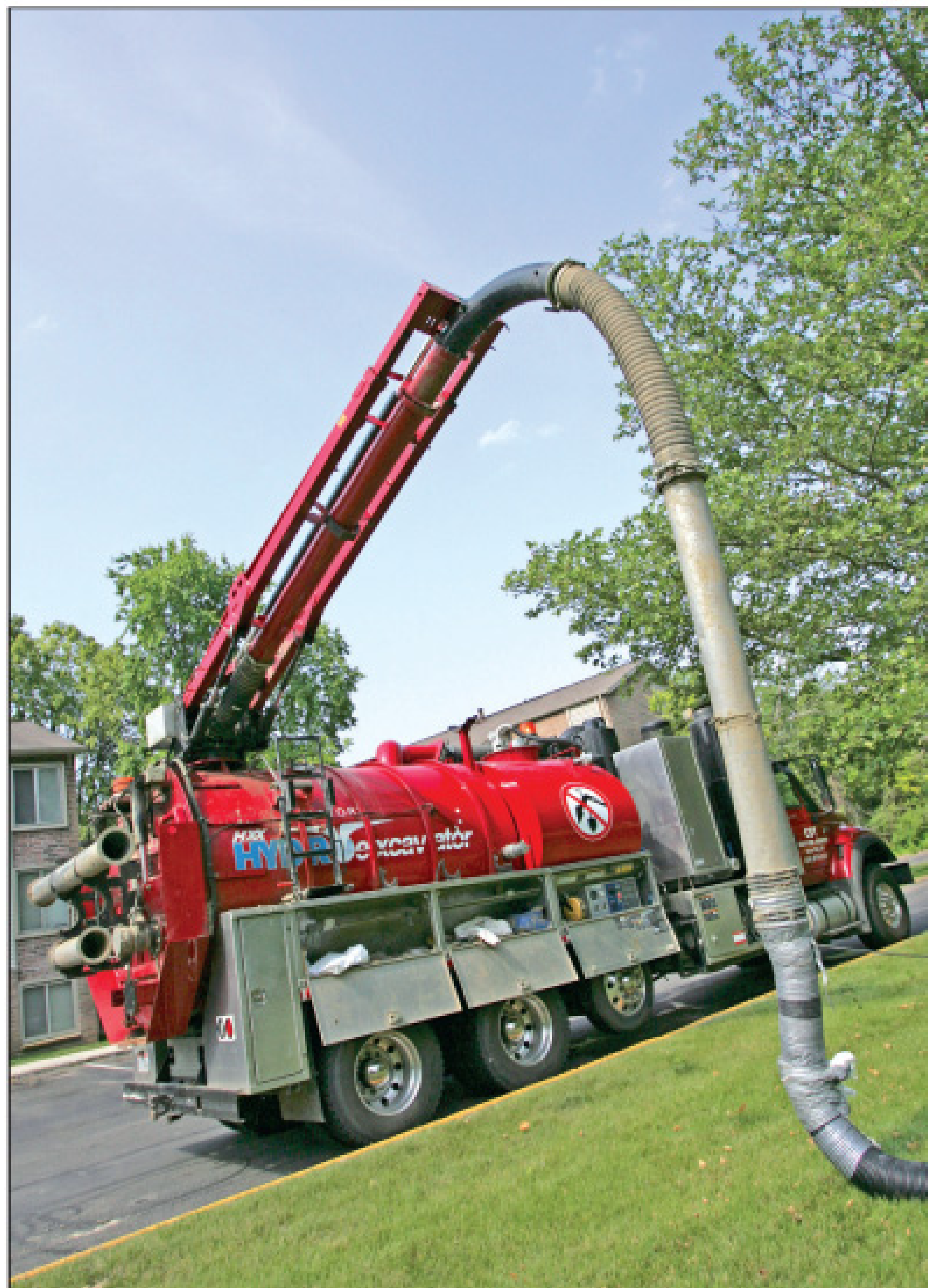
The company's Vactor hydroexcavator at work on a jobsite. A crew of three worked on exposing electric and petroleum lines outside an apartment complex.
