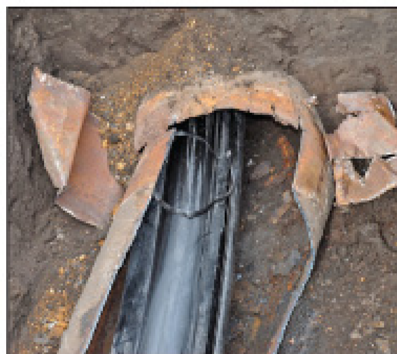
The 10-inch PE pipe negotiates a fabricated bend in the larger steel pipe.
