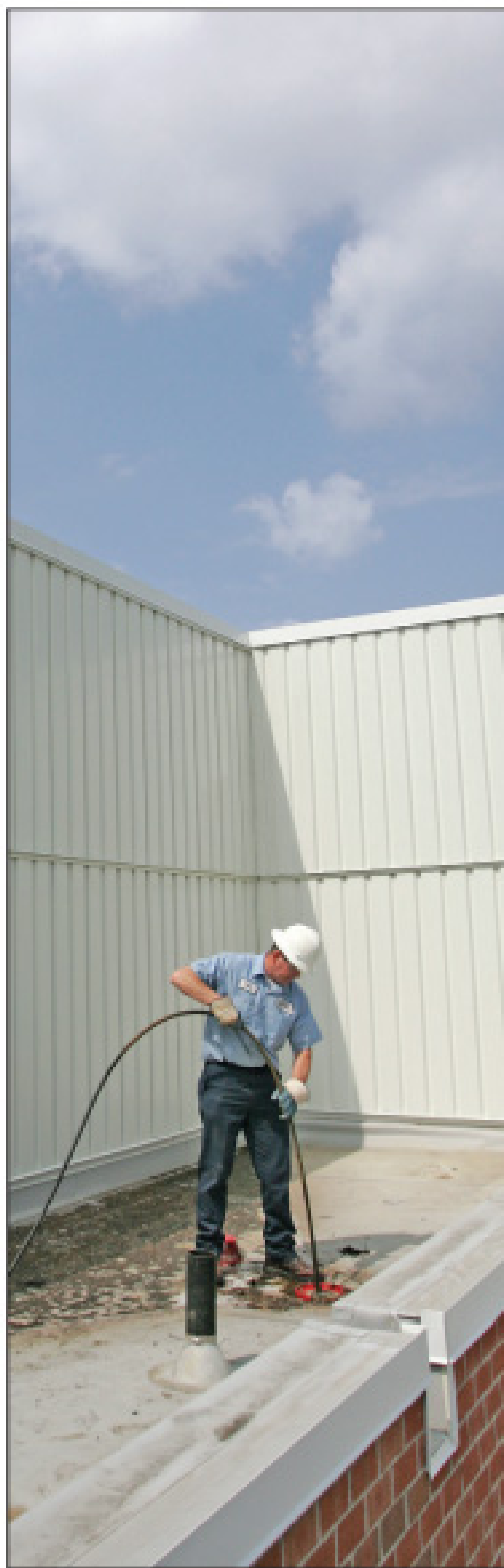
Chuck Lang Jr. uses a jetter to unclog drains at a middle school in Columbus.
