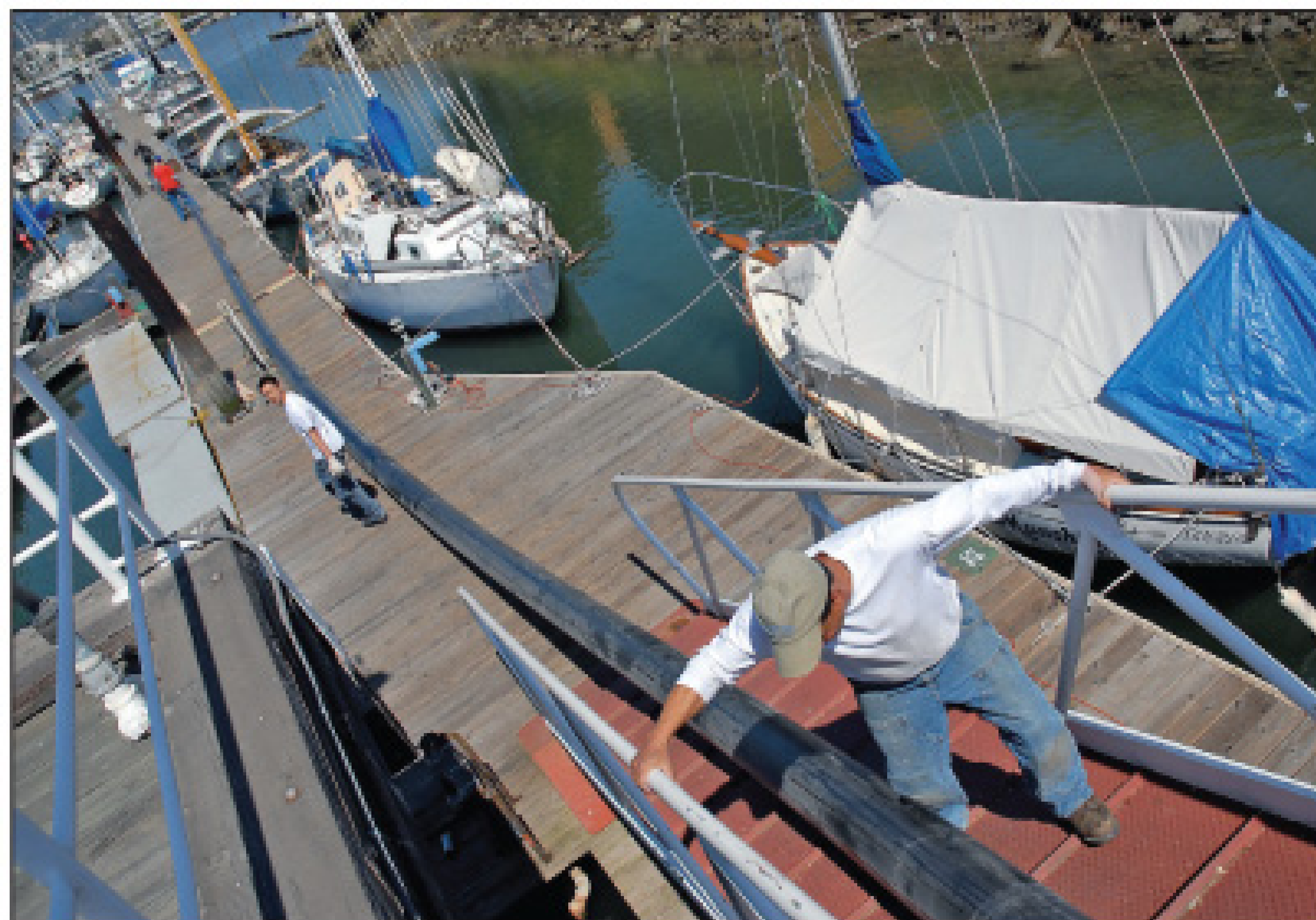
The last portion of the 175-foot length of 10-inch PE pipe is coaxed down the gangplank.
