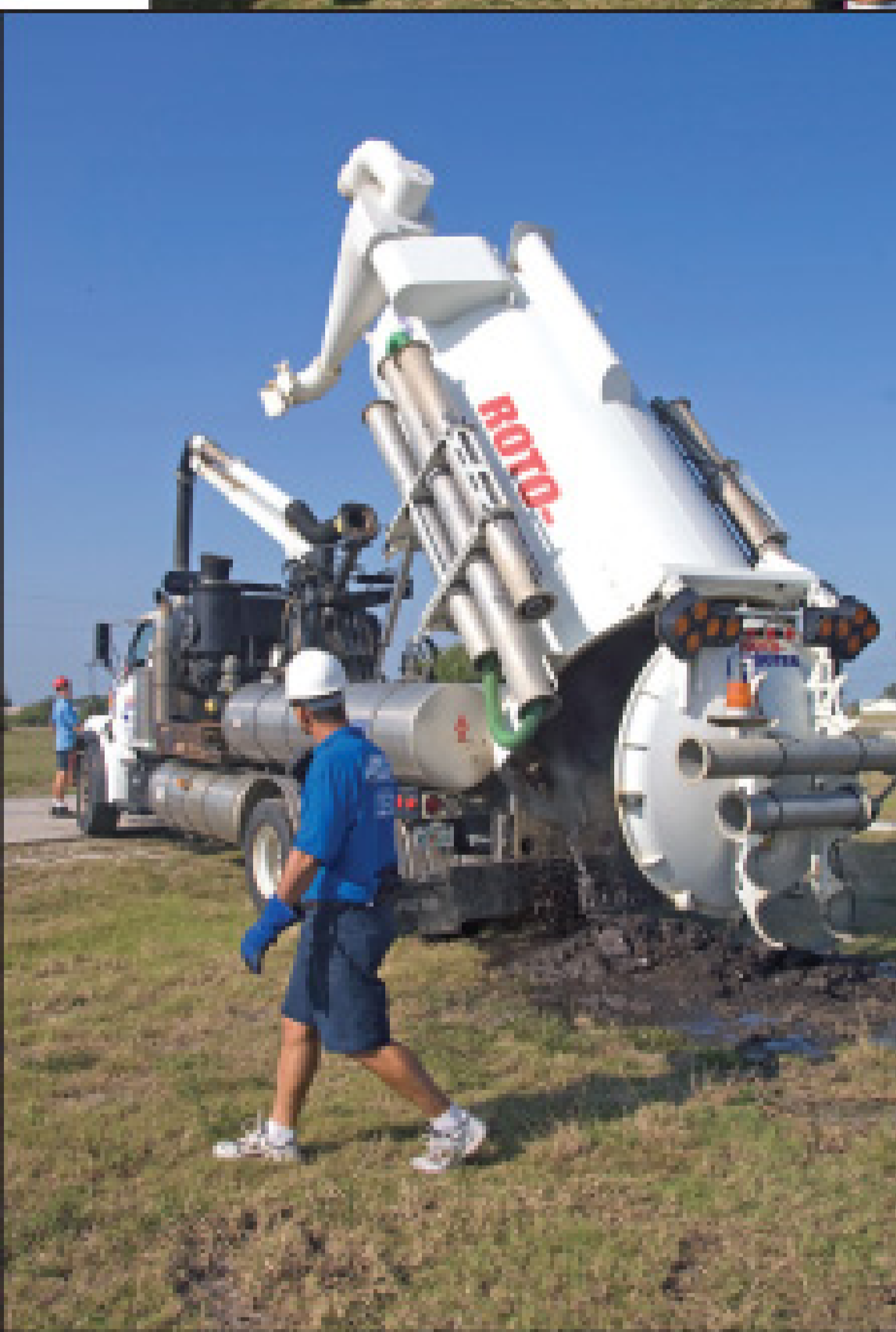
Jeff Caponi, a service manager for Roto-Rooter Plumbing & Drain Service in Cape Coral (Fla.) walks by the Vactor 2100 while employee Mike Chastain operates the truck during uploading.
