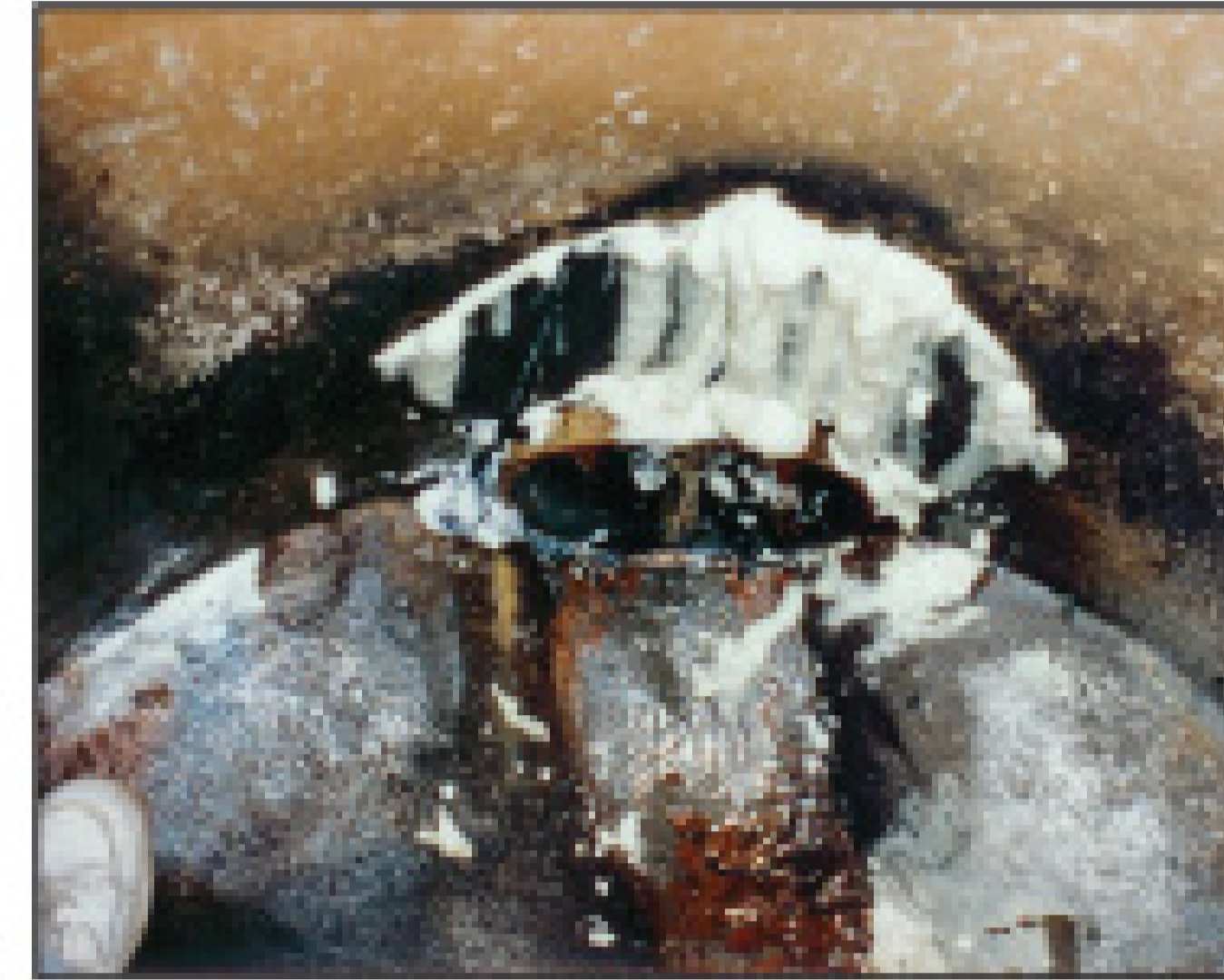
Hydrophilic chemical grout is injected around the area. Activated by the water, the grout expands to seal off any leaks.
