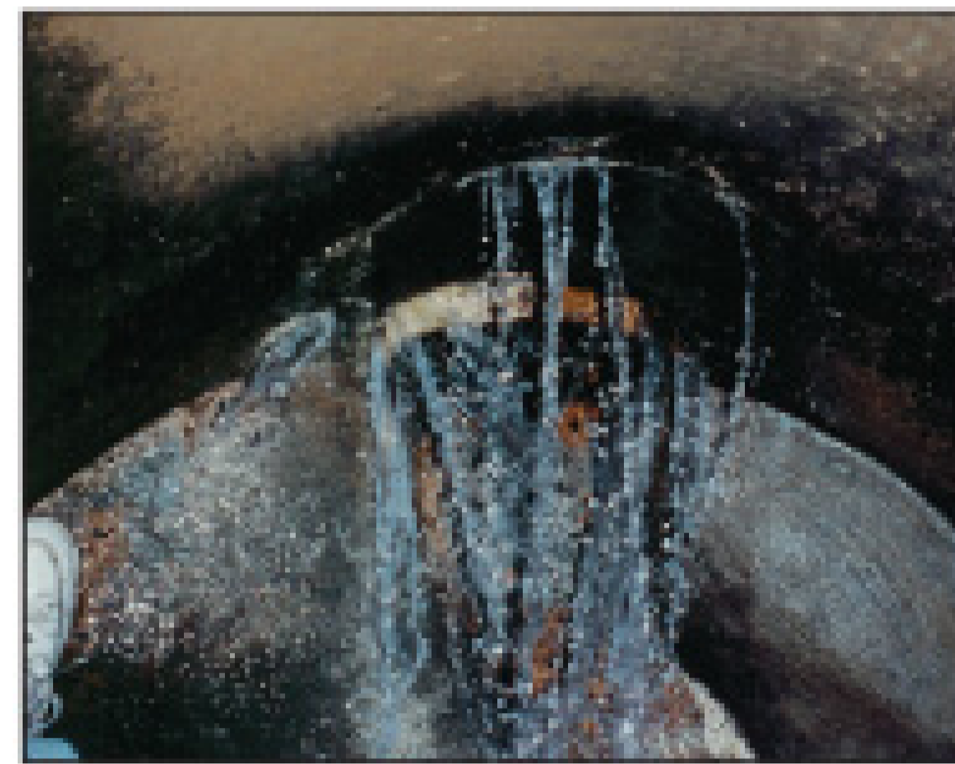
Water enters the manhole due to a pipe penetration.
