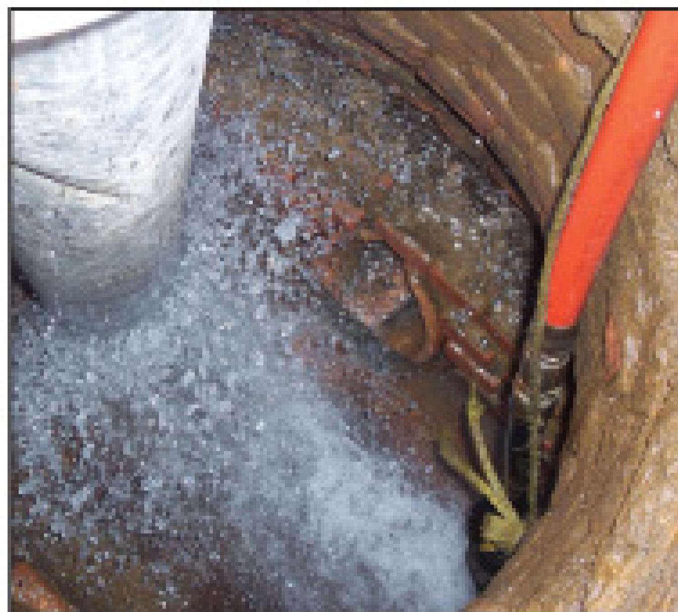
The KEG floor cleaner brings debris back to the manhole for removal by the Vac-Con's three-stage blower.
