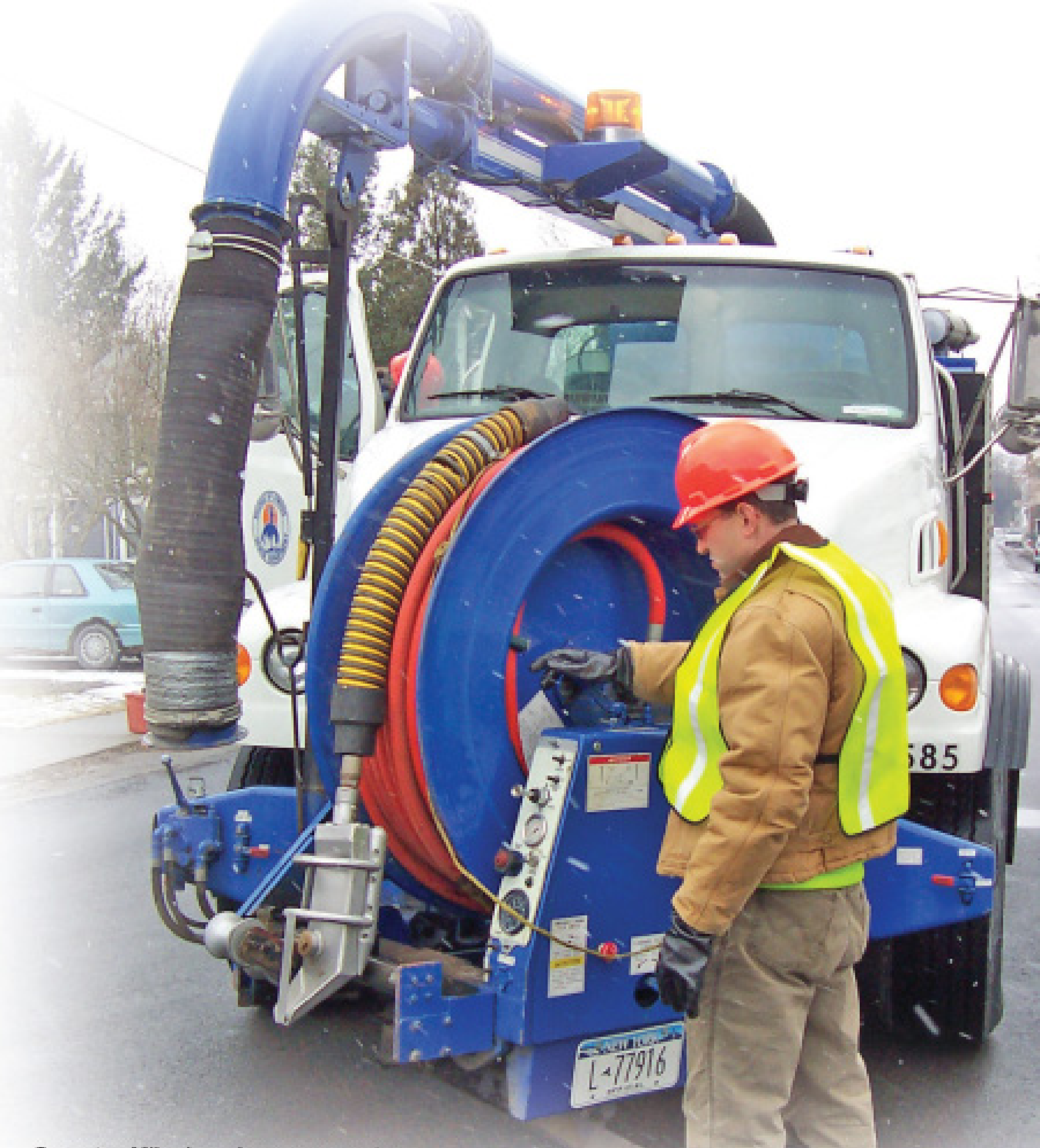
Operator Mike Lanning prepares to lower the KEG floor cleaner into the 24-inch combined sewer line.
