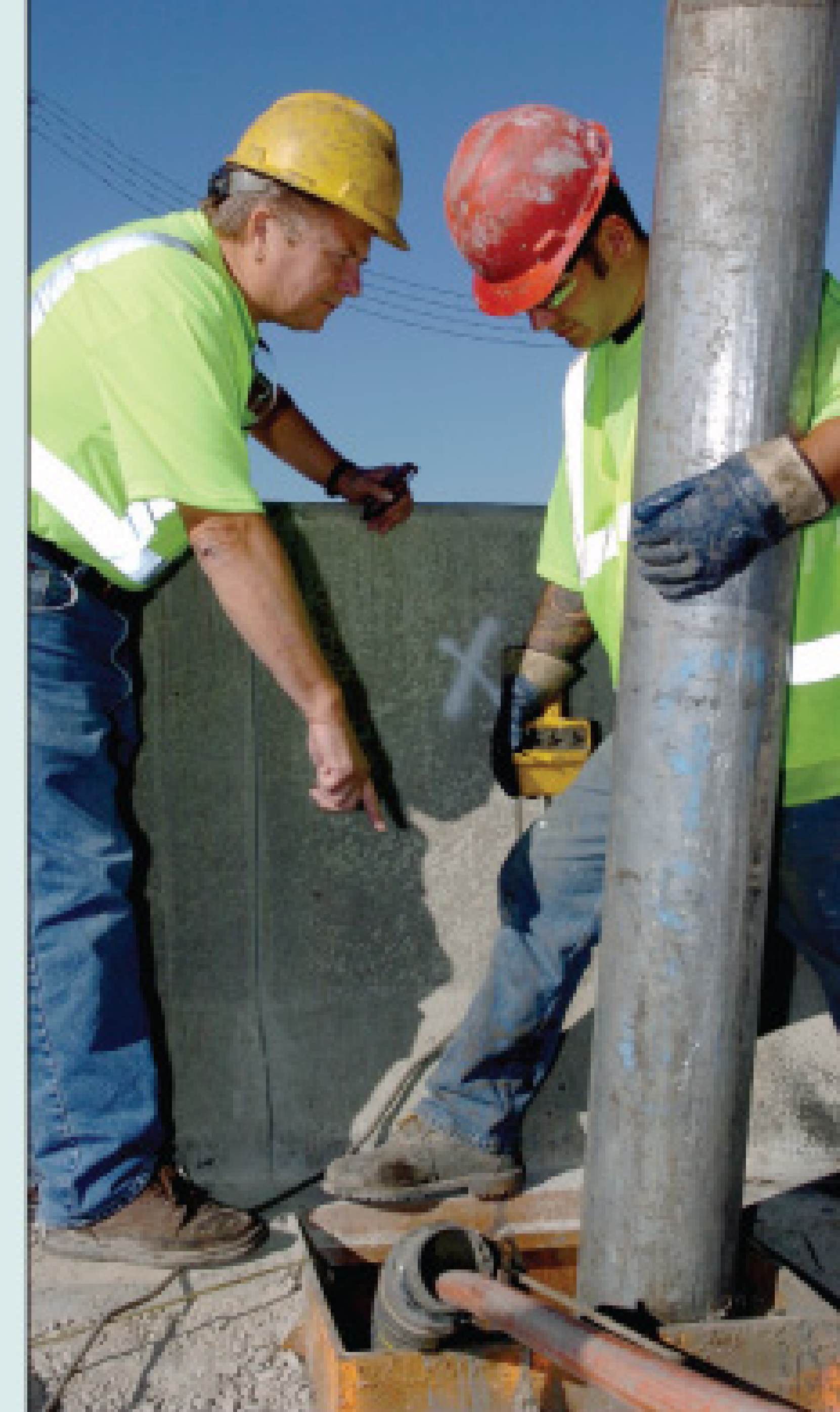
Owner Al Kulig (left) and operator Chuck Cushing discuss progress on an obstructed sewer line.
