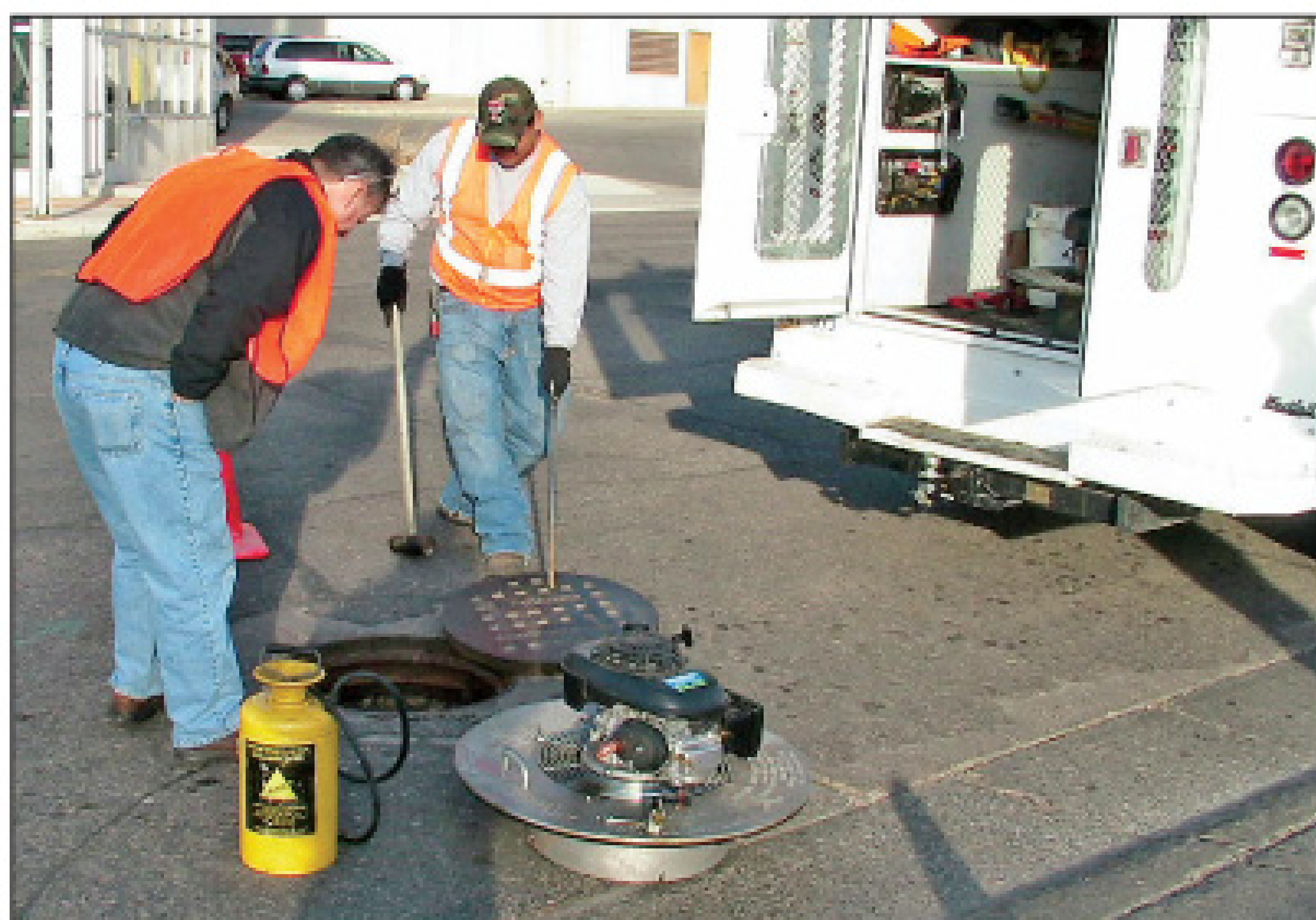
Smoke testing requires little more than a smoke-generating device, a blower, and a knowledgeable crew. (Photo courtesy of Cherne Industries Inc.)
