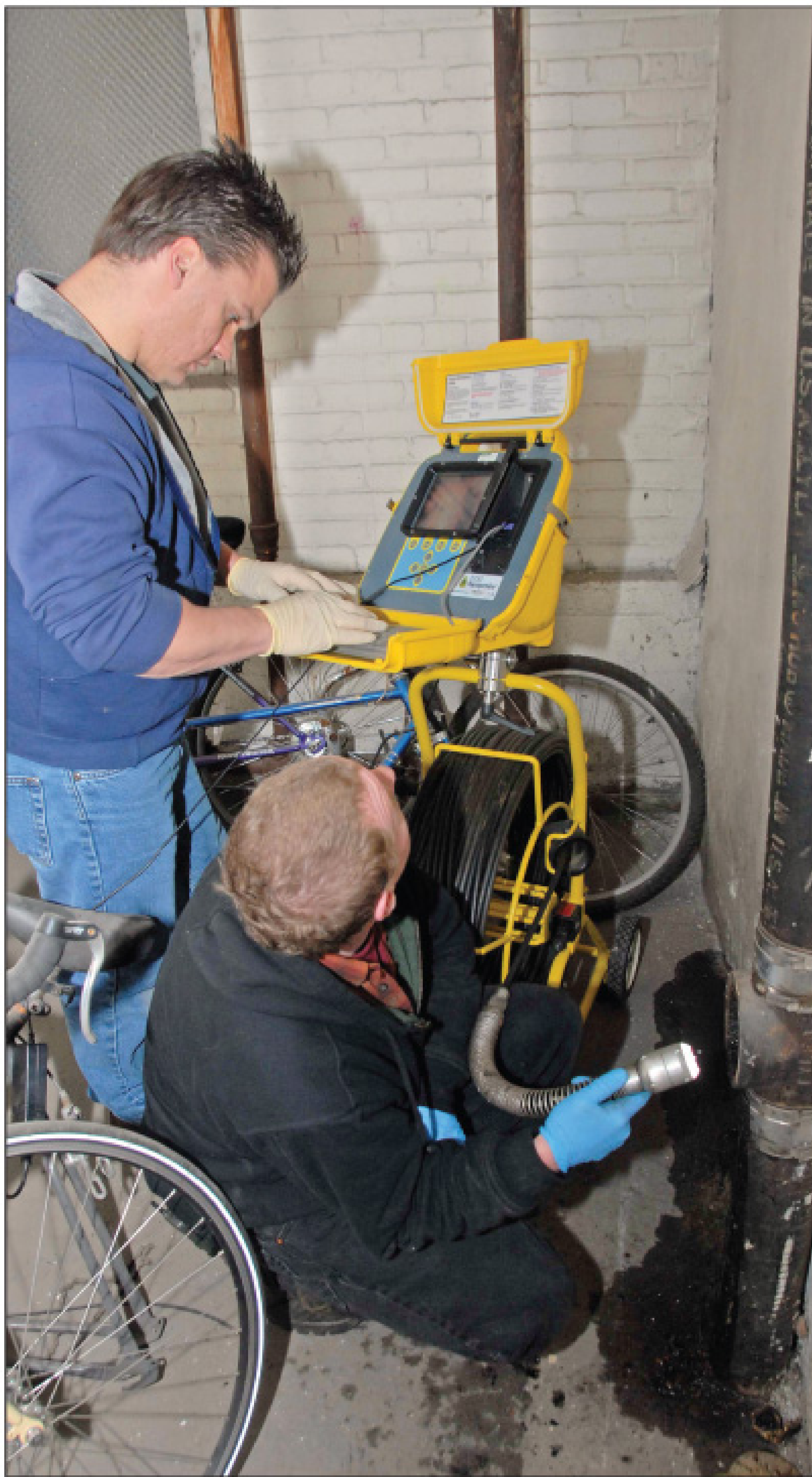
Mass Sewer & Drain owner Kenny Litalien and technician Barry Nelson prepare a Flexiprobe P330 system from Pearpoint for an inspection. The company has made inroads to its market with an emphasis on inspection and locating. (KarwanPhotos.com)
