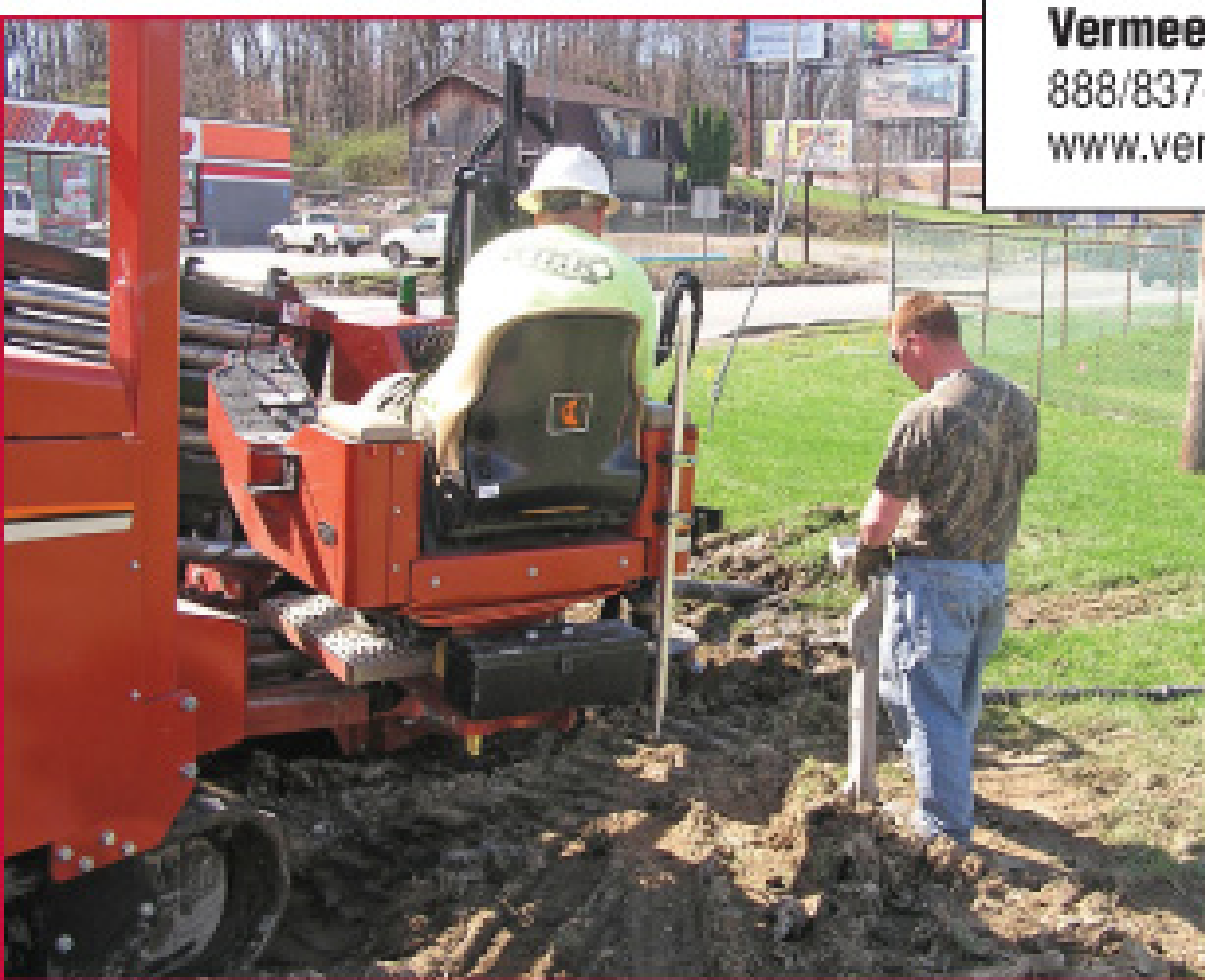
Scott Heston of Kirk Excavating operates a Ditch Witch JT4020 Mach 1 directional drilling machine while co-worker Casey Applegate uses a sonde to locate the boring head.
