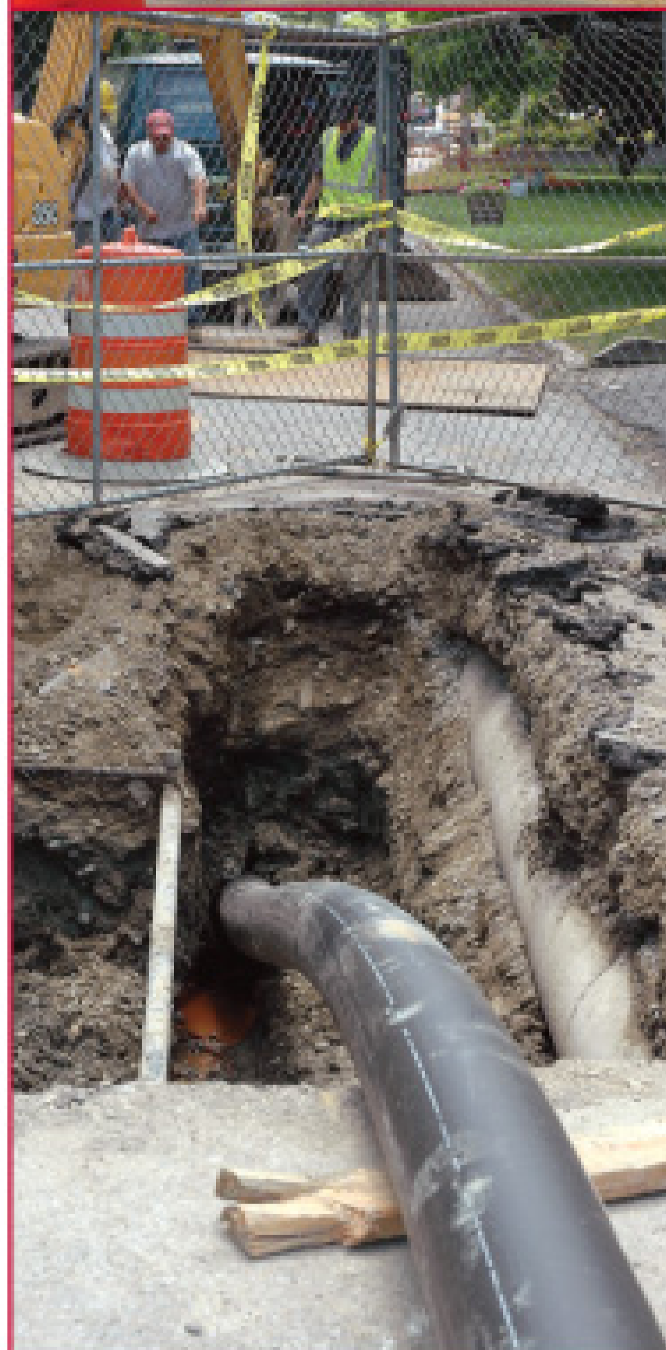
An 8-foot entry pit is excavated in front of the first manhole. A 4- by 3-foot exit (pull) pit is located 300 feet farther up the street.
