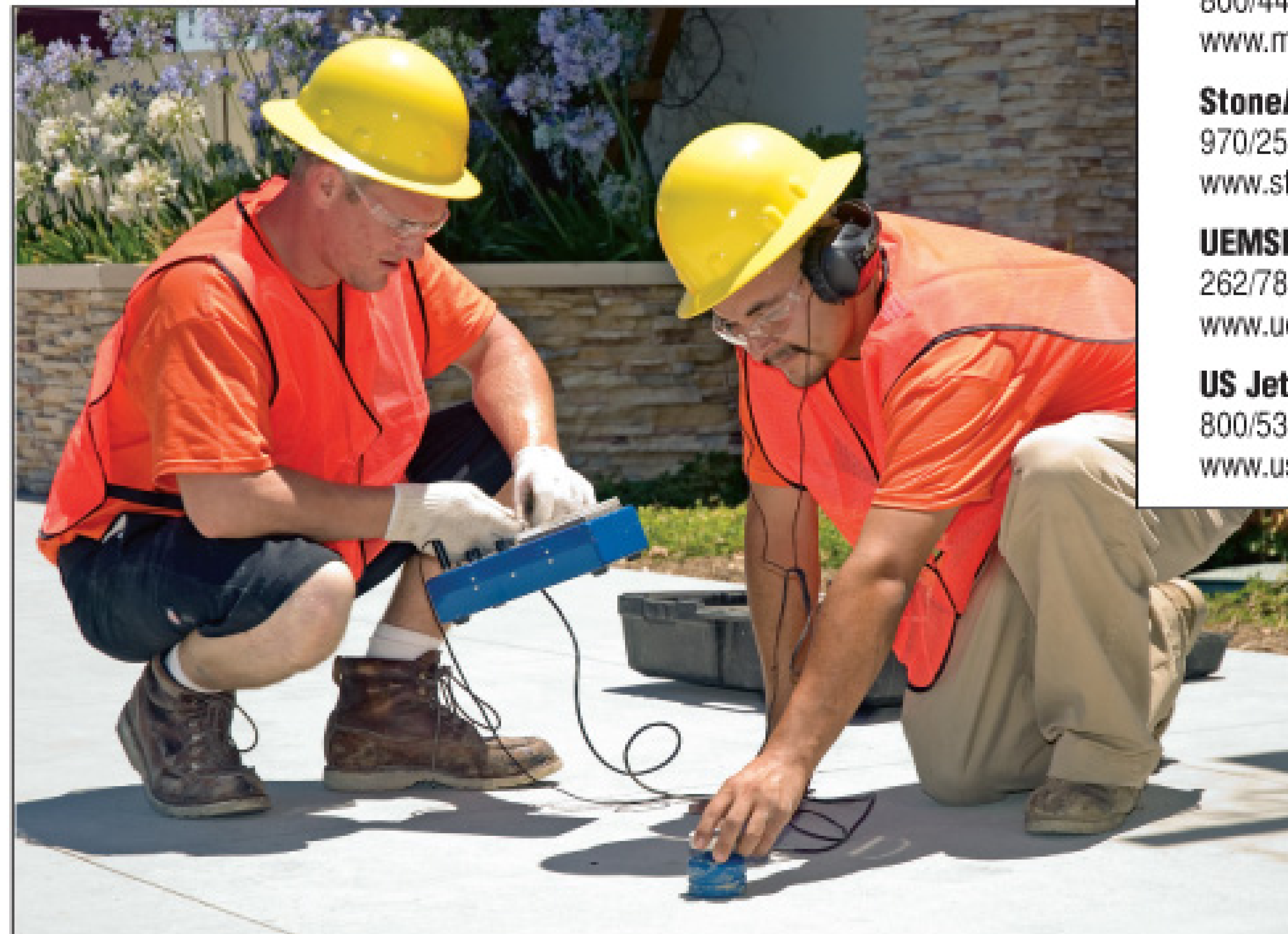
Robert McKechnie and Rafael Manzo (right) use a Goldak locator to pinpoint a leak at a California shopping mall.
