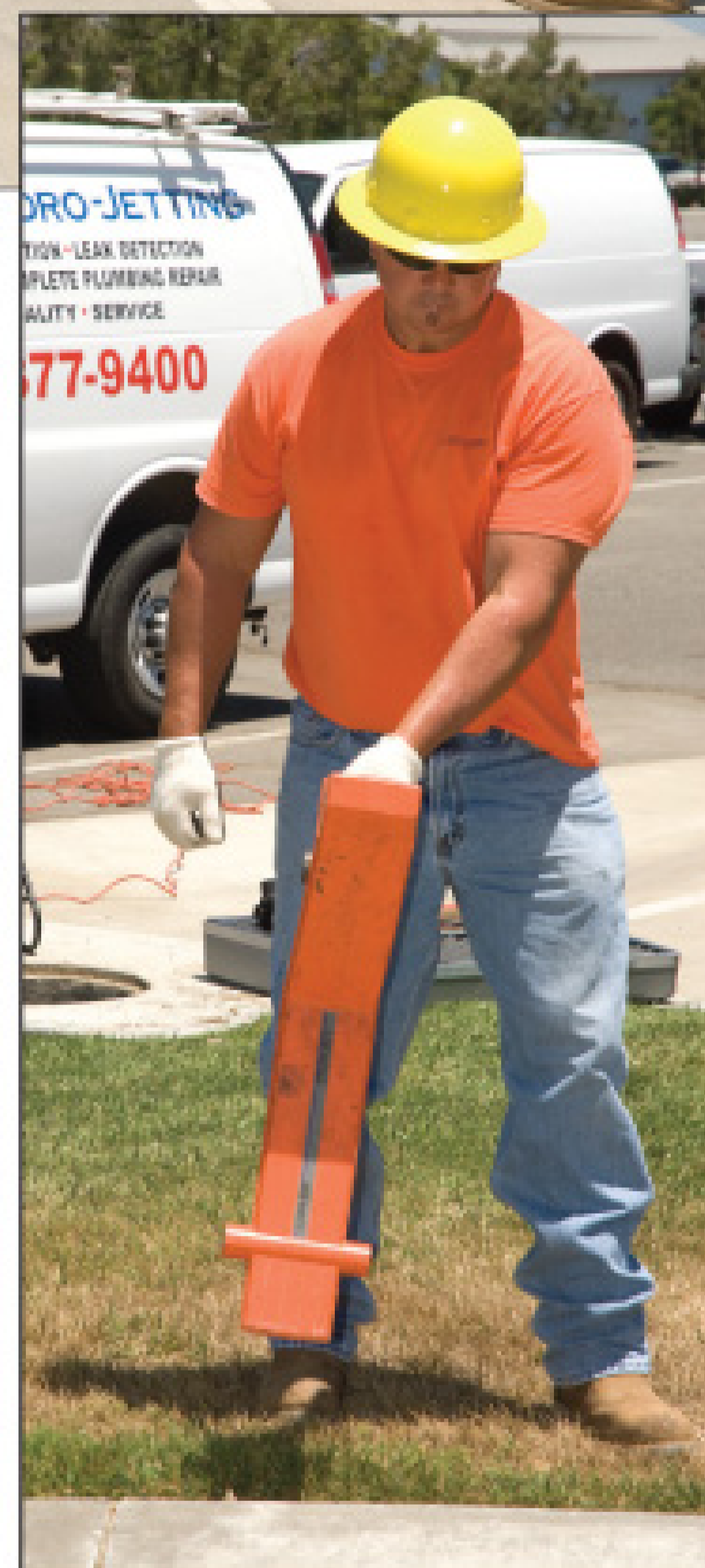
Dennis Carver uses a UEMSI locator to find where the storm drain connects to the trunk line.
