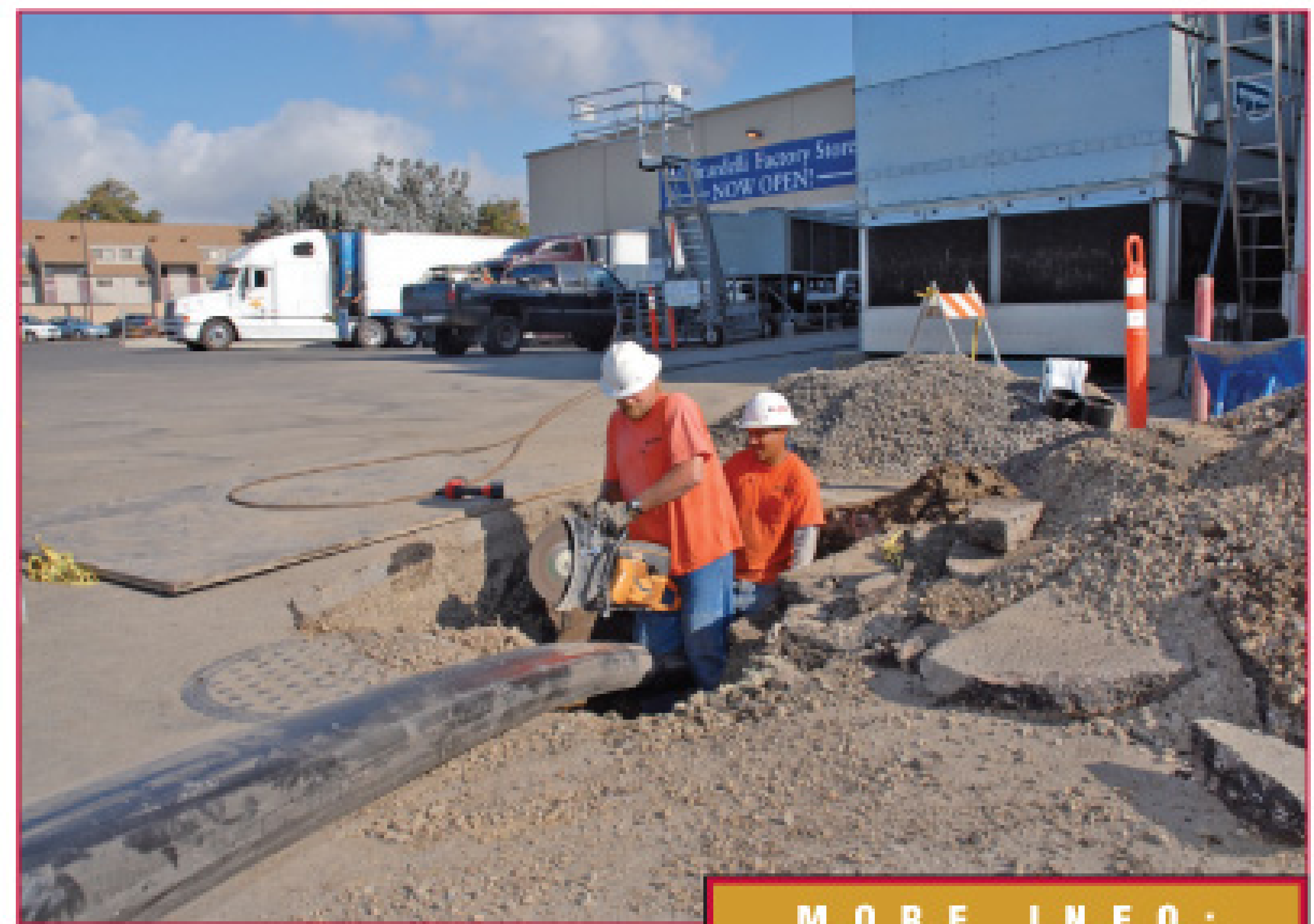
After the pull, a Nielson Construction crew cuts off excess pipe at entry pit.
