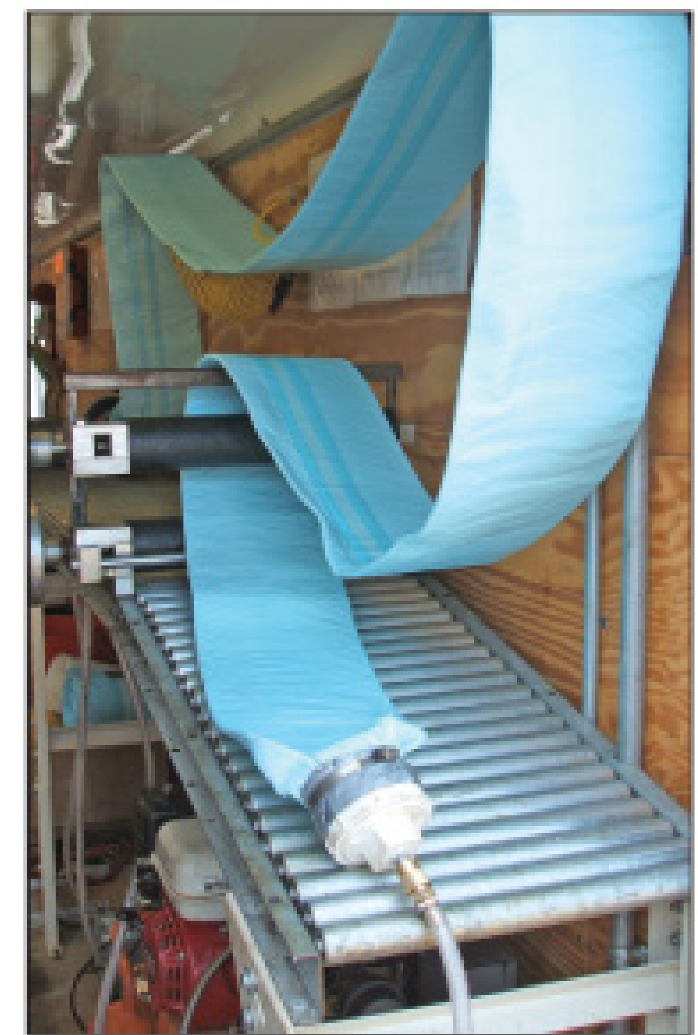
Cured-in-place pipe lining accounts for about 15 percent of Expert Plumbing Service's revenue. The division has seen extraordinary growth in the past year.
