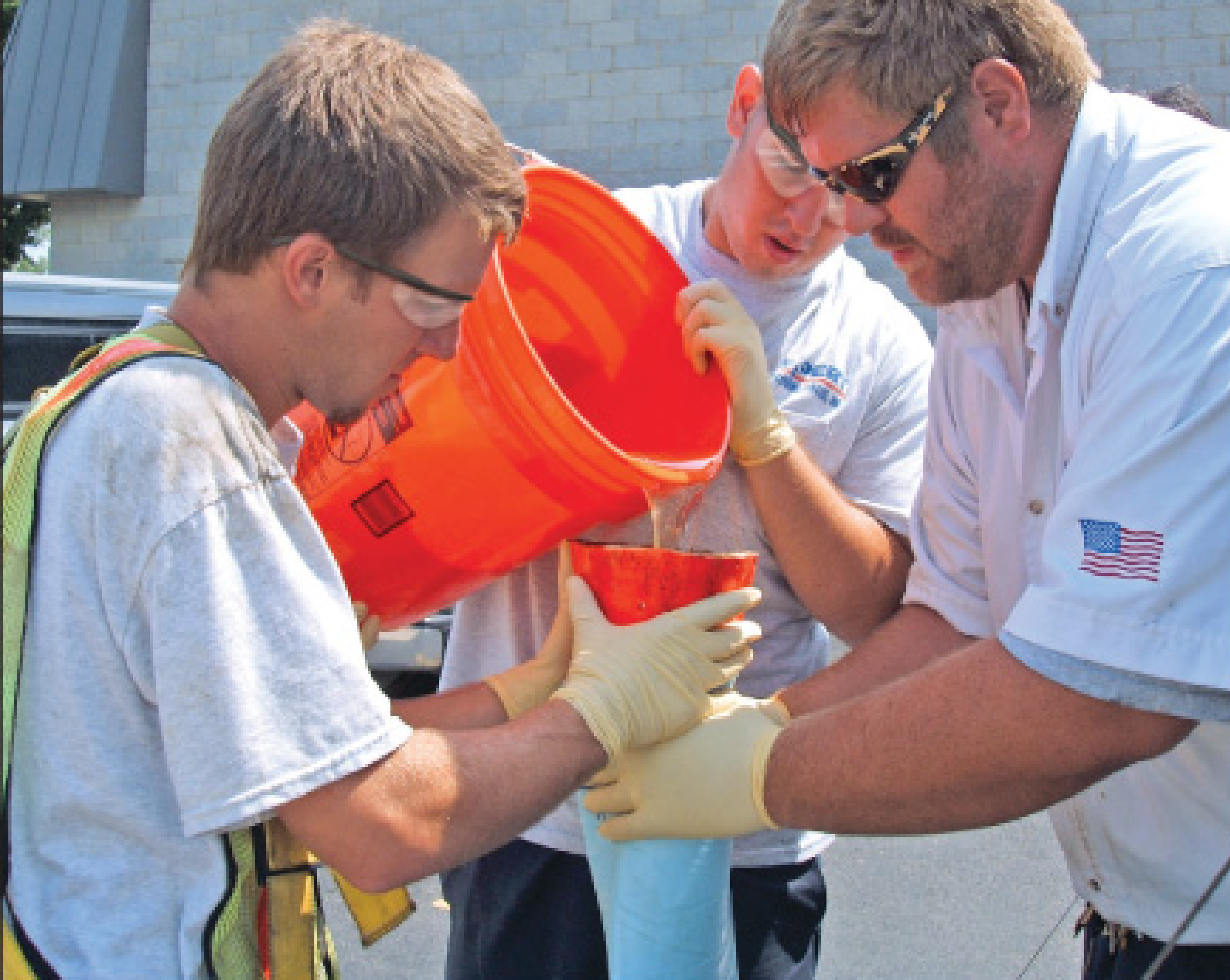
Anthony Coldwater, Matt Brennan and Mike Kampenga add resin to the liner. Expert Plumbing's three divisions enables the company to avoid laying off highly trained personnel by rolling them from one division to another during slow periods.
