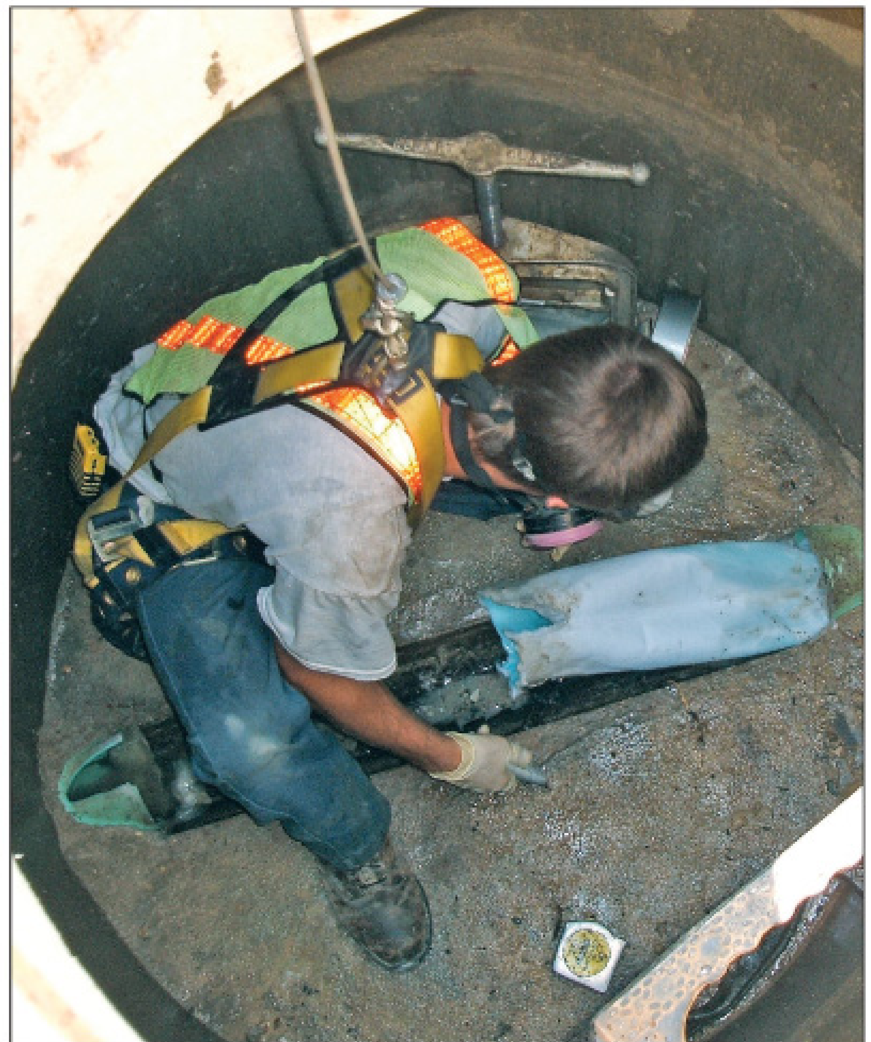
Anthony Coldwater works on relining a sewer lateral at an office strip mall in New Lenox, Ill. Pipe lining represents one-third of the services offered by Expert Plumbing Service Inc. The company's other two divisions specialize in plumbing and jetting. (Photography by Dave Kenik)
