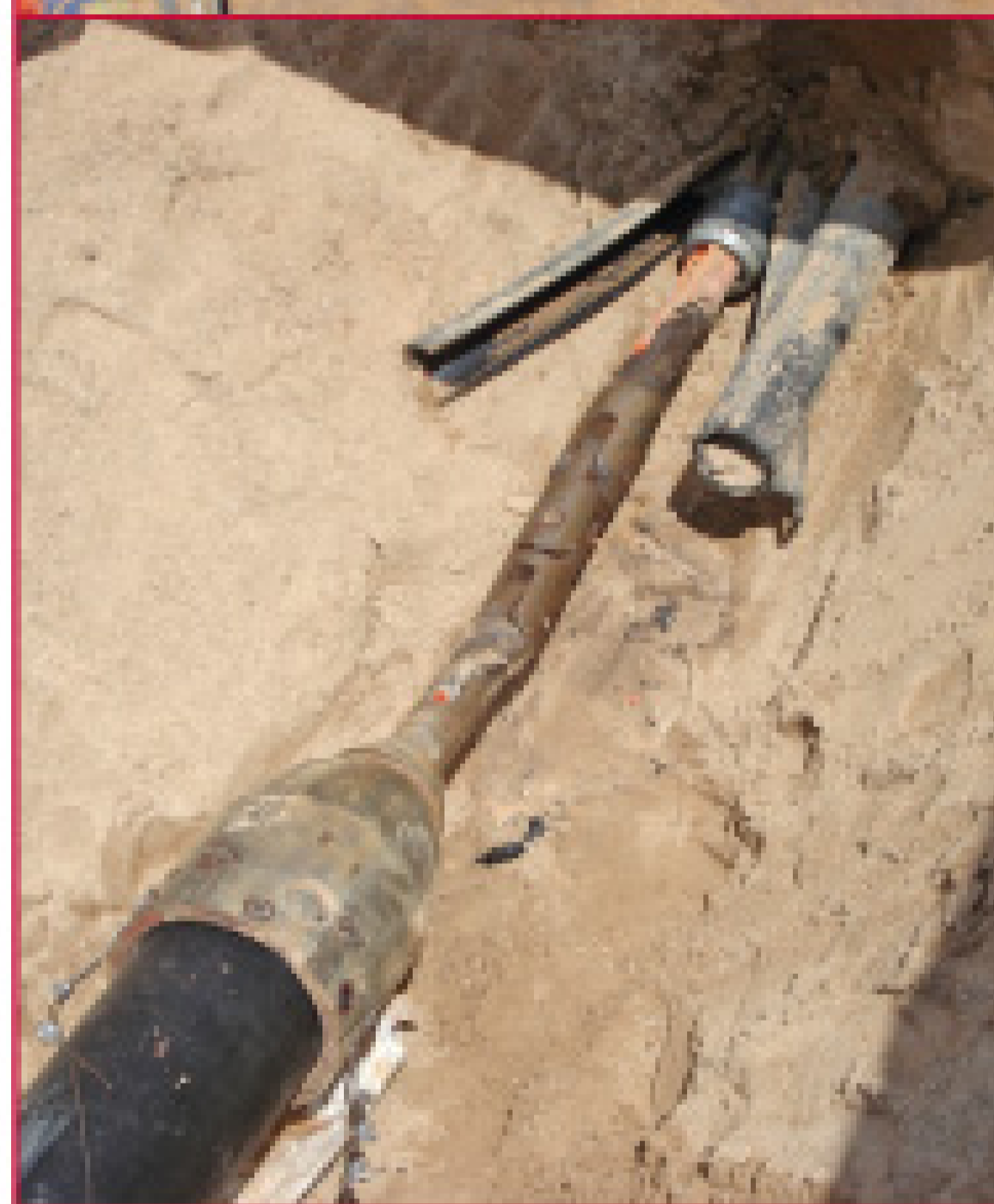
Crews used a specially designed quad cutter to split the existing 4-inch HDPE force main and replace it with 8-inch HDPE.
